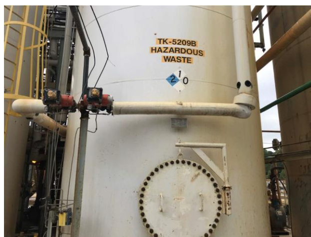
Photo 53: Slurry Tank TK-5209B.
