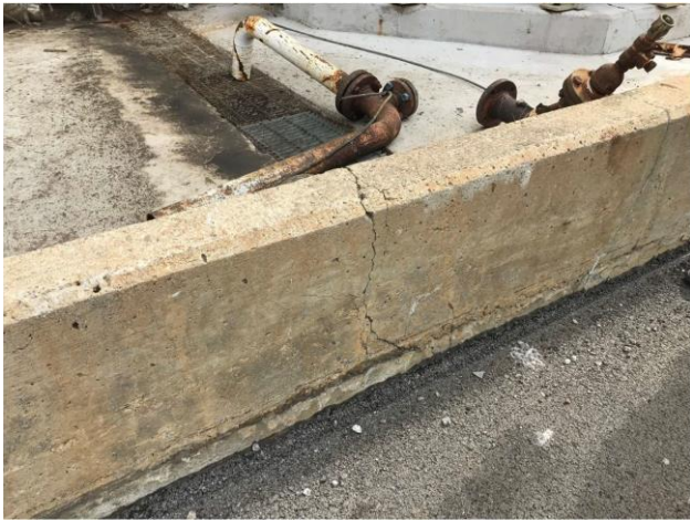
Photo 60: Cracks in secondary containment near Slurry Tank TK-5210.
