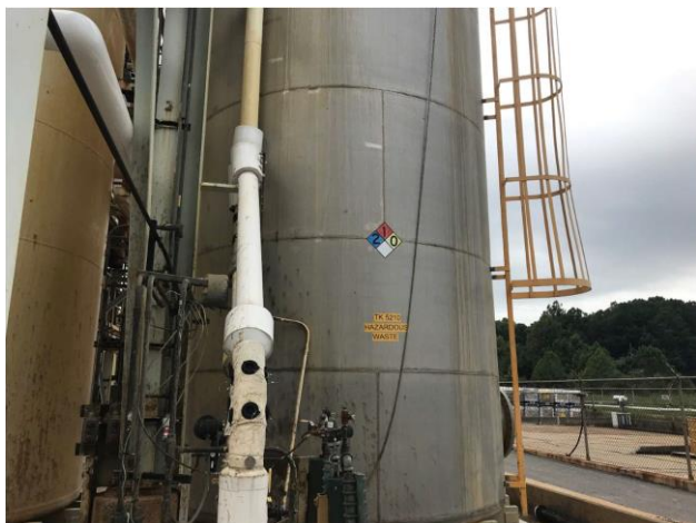
Photo 54: Slurry Tank TK-5210.
