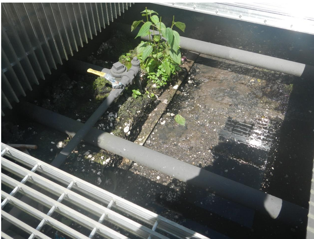
Photo 2: Vegetation and clog within clarifier.
