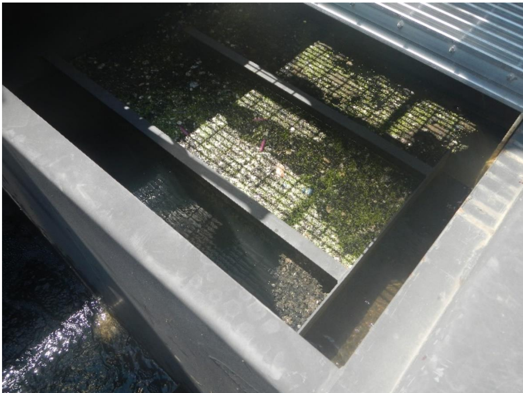
Photo 4: Sludge backup in clarifier.
