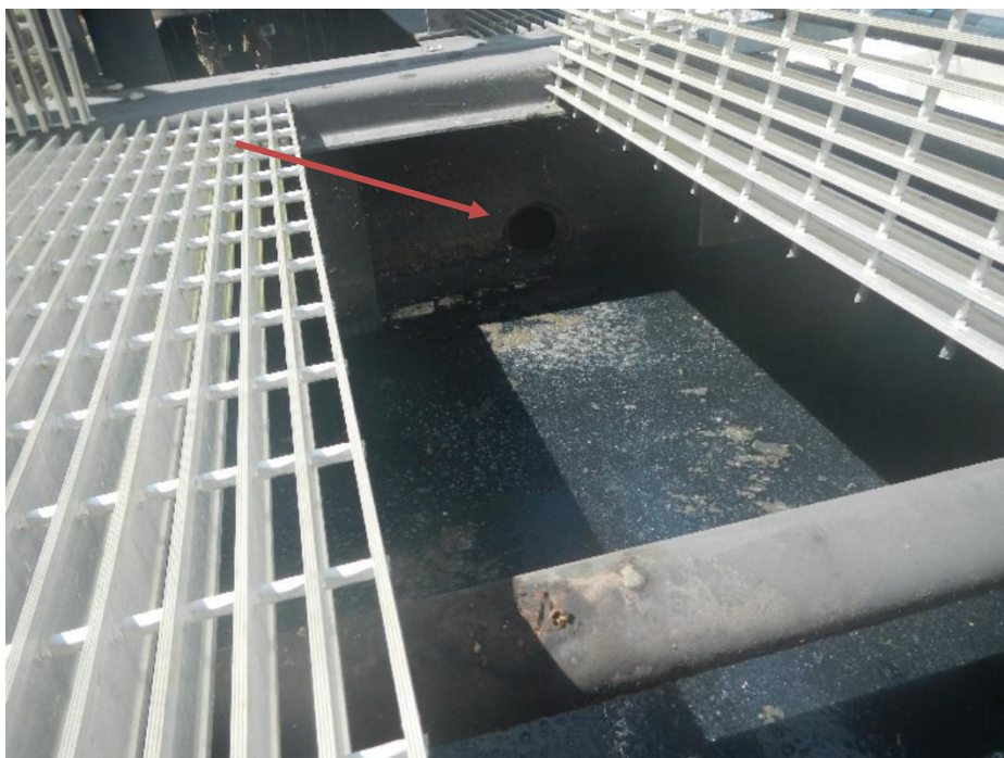
Photo 1: Hole located in wall of wasting tank section causing flow to move improperly through the facility.
