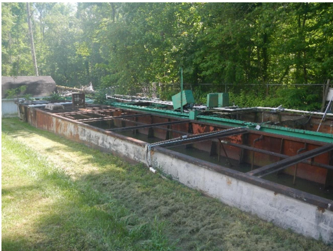
Photo 8: Decommissioned original package plant
