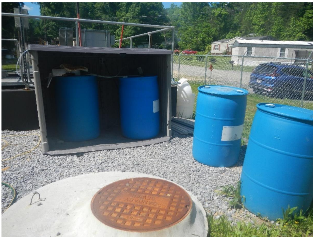
Photo 6: Open storage for chlorination/dechlorination chemicals.
