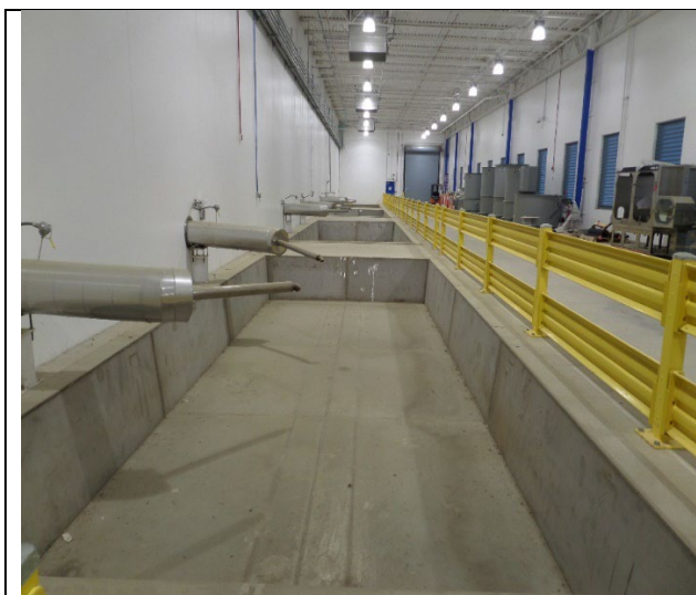
Corning. Salt Shed. The inspectors observed four stainless-steel lined concrete pits (pit) that store potassium nitrate (D001) generated from the ion-exchange unit IOX-104. Observed guard rails. Photograph 3 taken at 11:55 a.m.
