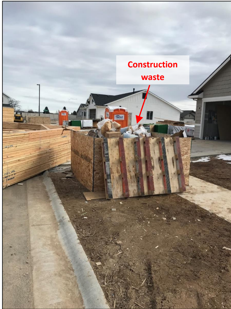
Photograph 8. View, facing east, of uncovered construction plywood container holding waste and debris at the eastern end of East Whig Drive.
