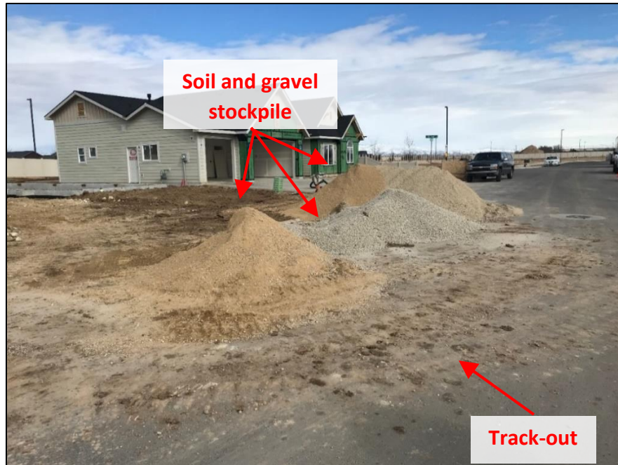
Photograph 6. View, facing southwest, of a location of three unstabilized soil and gravel stockpiles located at the intersection of North Destiny Avenue and East Sweet Pearl Street. Note the sediment track-out on East Sweet Pearl Street.
