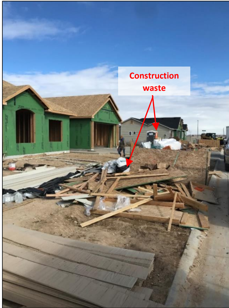
Photograph 10. View, facing east, of uncontained construction waste and an uncovered plywood container containing construction waste outside of house lot 876 on the western end of East Sweet Pearl Street.
