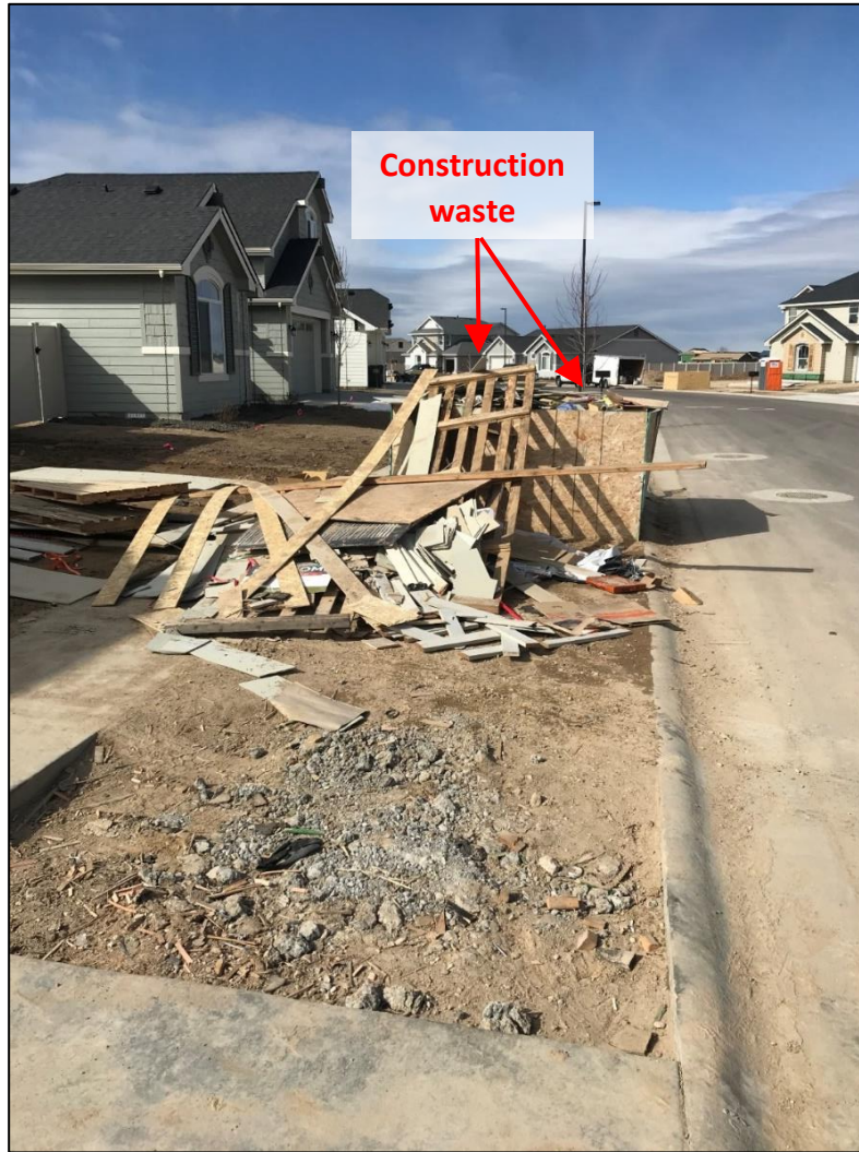
Photograph 9. View, facing east, of uncontained construction waste and an uncovered plywood container containing construction waste outside of house lot 2009 at the center of the Site on North Windmill Way.
