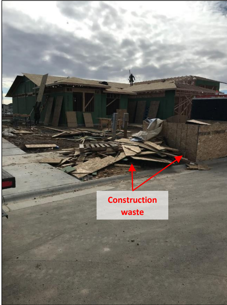
Photograph 11. View, facing south, of uncontained construction waste and an uncovered plywood container containing construction waste at the southern end of North Elk Creek Avenue.
