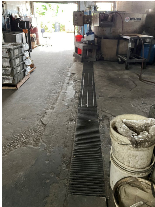
Photo #2. Process waste streams are directed into the floor drain then to the collection pit.
