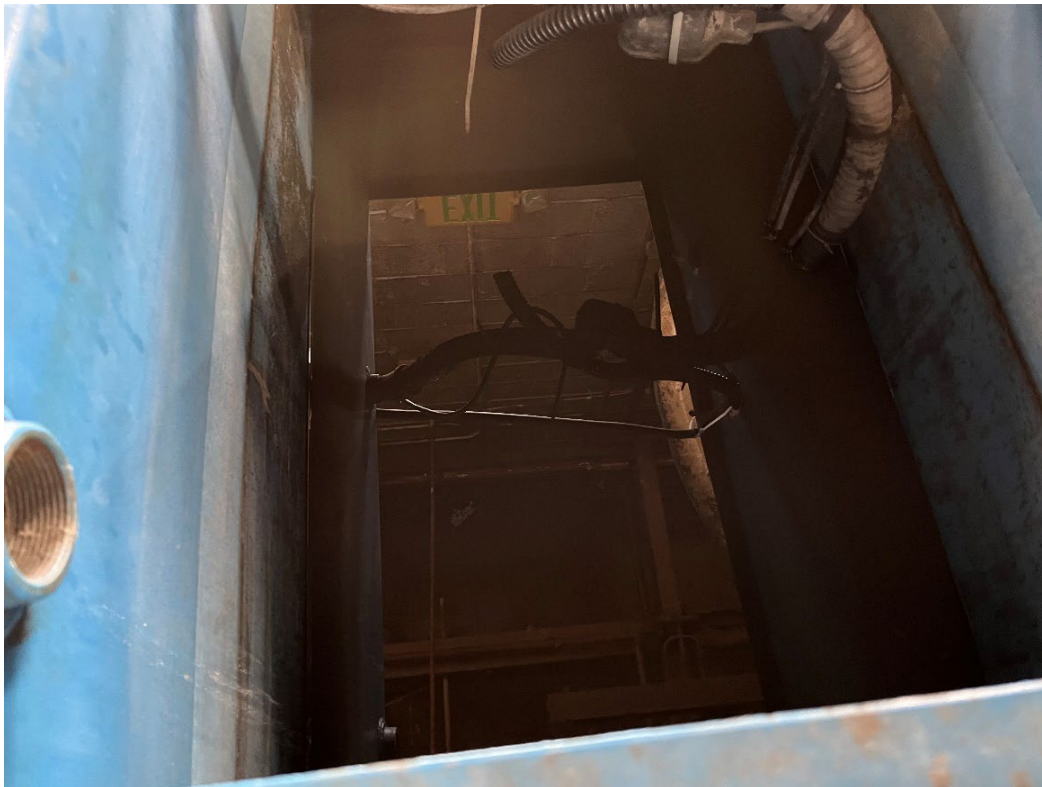
Photo #6. Wastewater is pumped into the influent receiving chamber.
