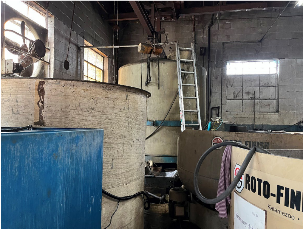
Photo #3. Wastewater in the collection pit is pumped to the receiving tank.
