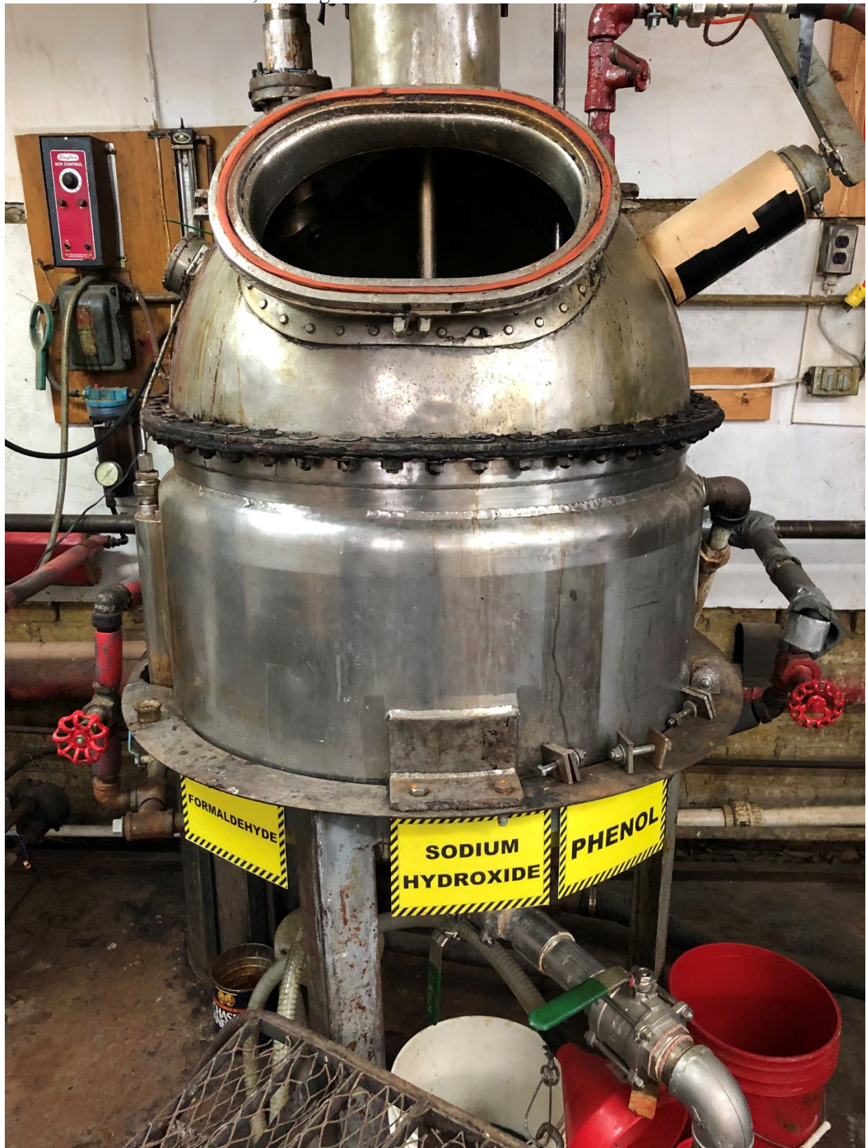
Photo #2: View of Kettle 3, the large reactor.
