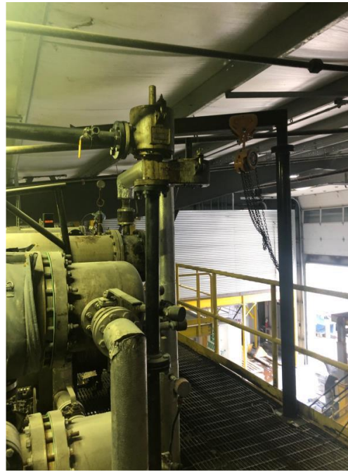
Vapor Collection Line for Decanter #1
