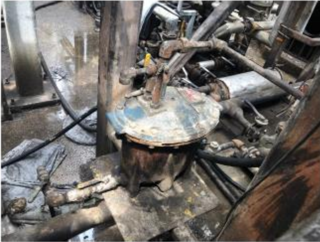
Methanol Condensate Pump.
