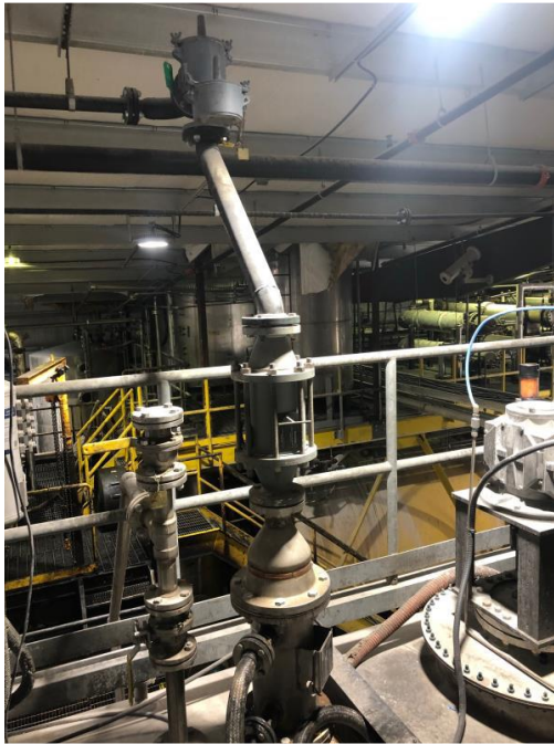
Vapor Collection Line for the Acid Esterification Reactor
