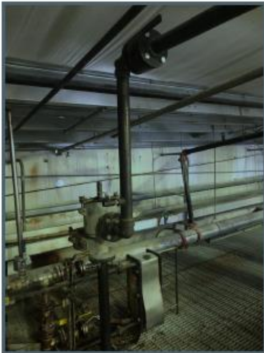
Vapor Collection Line for Decanter #2
