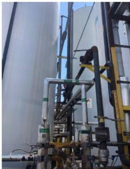
Vapor Collection Line for Tanks 901 (SMO), 902 (Methanol), 903 (Glycerin), 904 (Methanol), and Methanol Distillation Column
