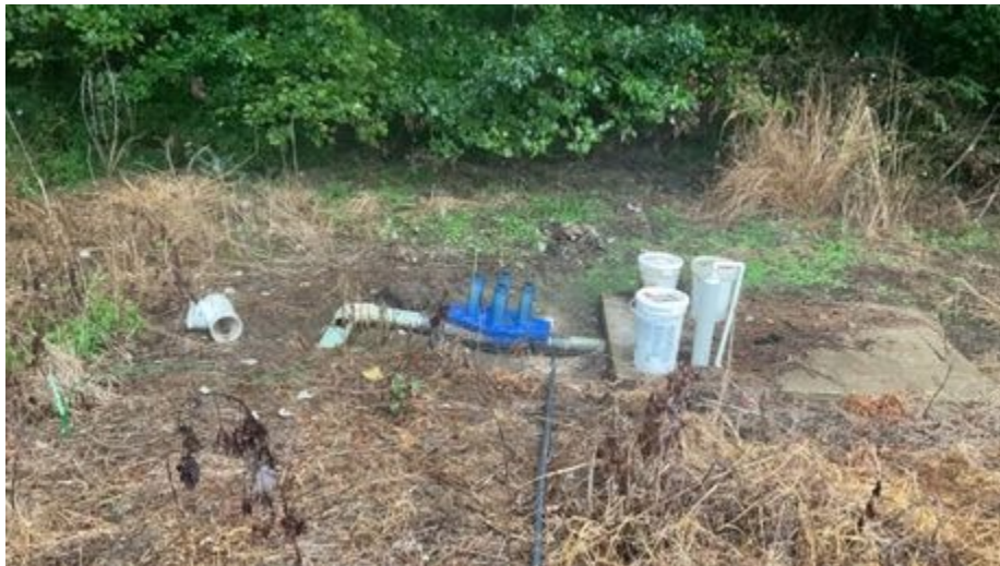
Figure 2: Effluent Discharge Chlorine Tablet feed system. Taken 8/8/23 Taken 15:00
