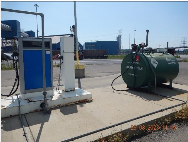
Photograph 14. DTE - Monroe Plant DSCN0100.JPG Description: View, facing east, of a fueling station across from the Motor Pool Building. The 500 gallon, double-walled diesel storage tank is visible on the right side of the photo.
