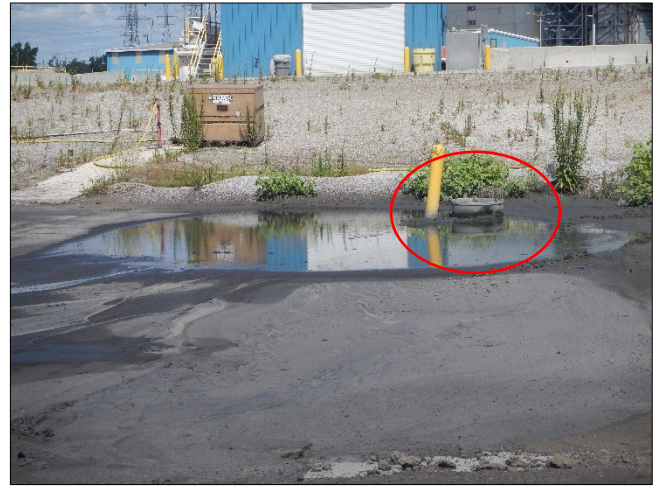
Photograph 107. DTE - Monroe Plant DSCN0193.JPG Description: The Bottom Ash Transfer Pad is equipped with a sump in each corner (circled). The sumps pump stormwater back to the sedimentation basins.
