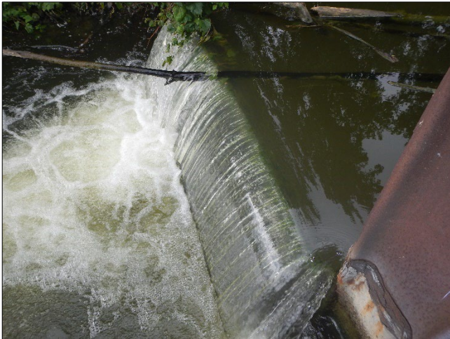
Photograph 66. DTE - Monroe Plant DSCN0152.JPG Description: Close view of the Outfall 001F effluent weir. The permittee referred to the weir as "v notch" but looked to be a rectangular weir.
