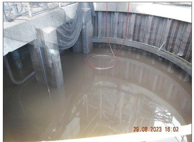
Photograph 40. DTE - Monroe Plant DSCN0126.JPG Description: General view of SS#3.
