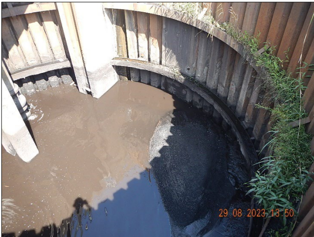
Photograph 2. DTE - Monroe Plant DSCN0088.JPG Description: Additional view of SS#6 seen in Photograph 1.
