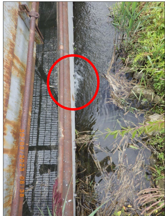
Photograph 122. DTE - Monroe Plant RIMG3199.JPG Description: View of additional leaks in the containment wall on the western side of the inactive bottom ash basin.
