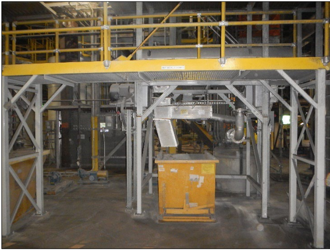
Photograph 105. DTE - Monroe Plant DSCN0191.JPG Description: General view of the centrifuges and OWSs inside the Generating Building.
