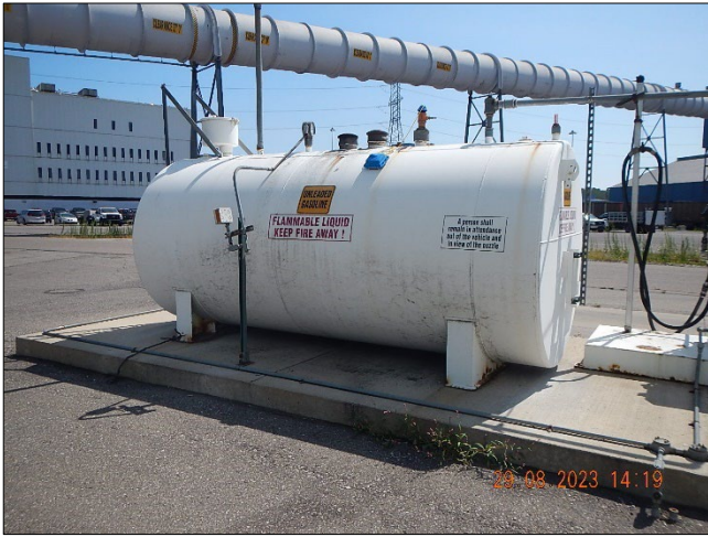
Photograph 13. DTE - Monroe Plant DSCN0099.JPG Description: View, facing east, of the double-walled gasoline tank at the fueling station seen in Photograph 14.
