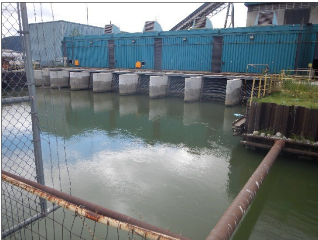
Photograph 86. DTE - Monroe Plant DSCN0172.JPG Description: View, facing south, of the cooling water intakes.
