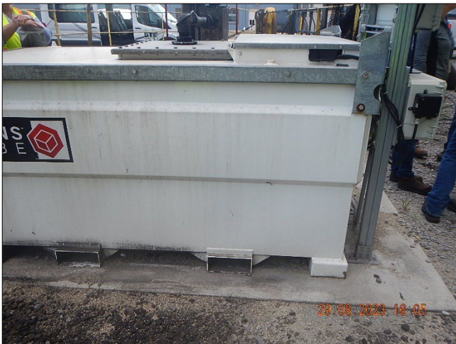
Photograph 42. DTE - Monroe Plant DSCN0128.JPG Description: General view of the double-wall used oil tank at SS#3.
