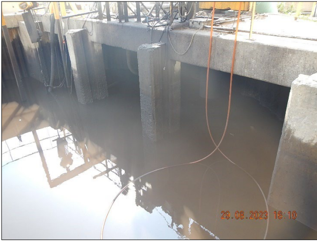
Photograph 45. DTE - Monroe Plant DSCN0131.JPG Description: General view of the SS#2 skimmer.
