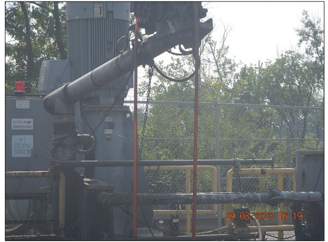
Photograph 51. DTE - Monroe Plant DSCN0137.JPG Description: General view of the SS#1 skimmer.
