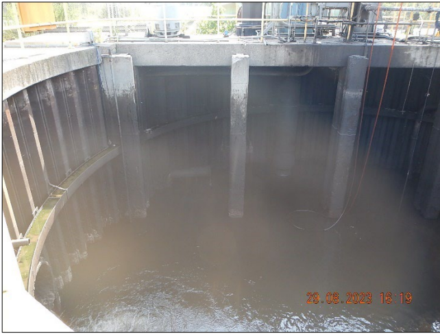
Photograph 49. DTE - Monroe Plant DSCN0135.JPG Description: General view inside SS#1.
