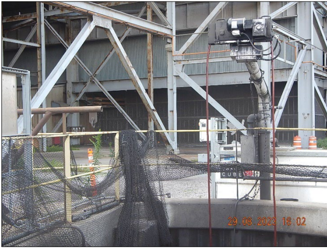
Photograph 41. DTE - Monroe Plant DSCN0127.JPG Description: General view of the SS#3 skimmer.
