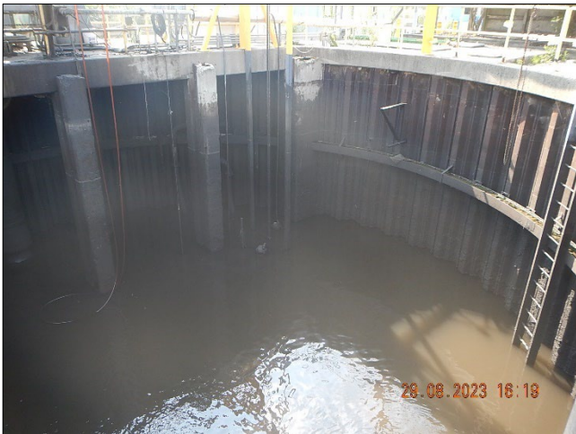
Photograph 50. DTE - Monroe Plant DSCN0136.JPG Description: General view inside SS#1.
