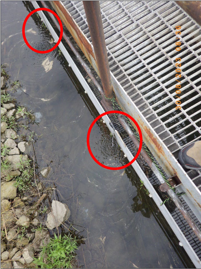
Photograph 117. DTE - Monroe Plant RIMG3194.JPG Description: View of additional leaks in the containment wall on the western side of the inactive bottom ash basin.
