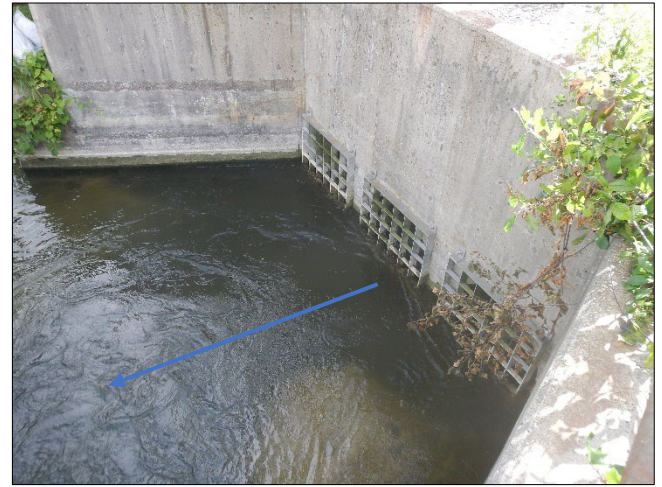
Photograph 59. DTE - Monroe Plant DSCN0145.JPG Description: General view of outflow from the Box Weirs Discharge Control Structure to the channel between the Fly Ash Basin and Outfall 001F.
