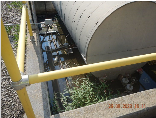
Photograph 46. DTE - Monroe Plant DSCN0132.JPG Description: View of the concrete containment area around the SS#2 single-wall used oil tank.
