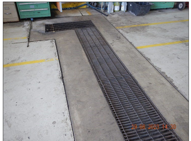
Photograph 20. DTE - Monroe Plant DSCN0106.JPG Description: General view of a trench drain inside the Motor Pool. The trench drain connects to SS#2 via an oil water separator (OWS).
