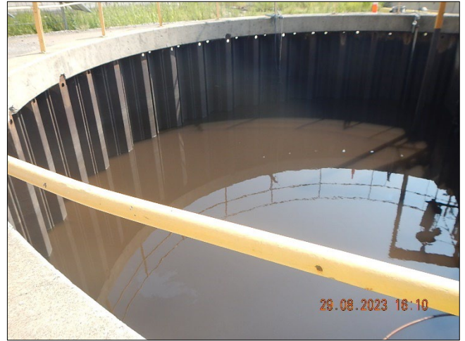
Photograph 44. DTE - Monroe Plant DSCN0130.JPG Description: General view of SS#2.
