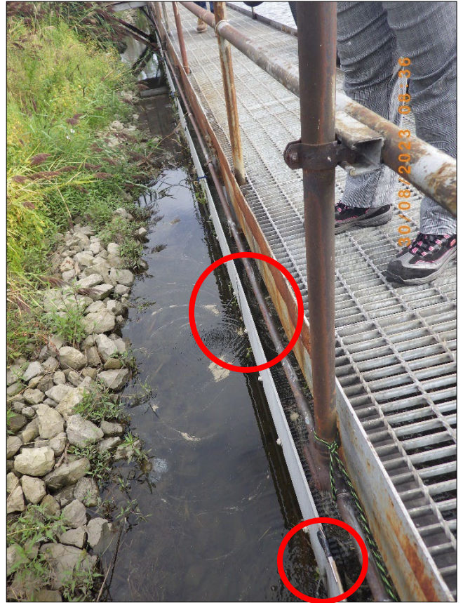
Photograph 118. DTE - Monroe Plant RIMG3195.JPG Description: View of additional leaks in the containment wall on the western side of the inactive bottom ash basin.
