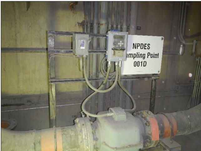
Photograph 102. DTE - Monroe Plant DSCN0188.JPG Description: General view of NPDES Sampling Point 001D inside the Generating Building. Flow is monitored with a mag meter.
