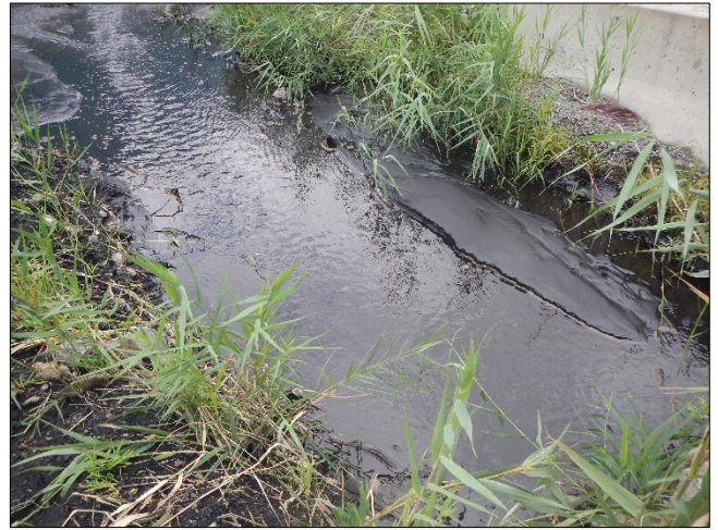
Photograph 99. DTE - Monroe Plant DSCN0185.JPG Description: The Process Swale starts east of SS#4.
