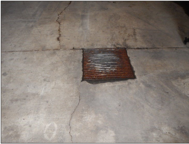
Photograph 101. DTE - Monroe Plant DSCN0187.JPG Description: Floor drains inside the Generating Building connect to the Oily Waste Treatment System.
