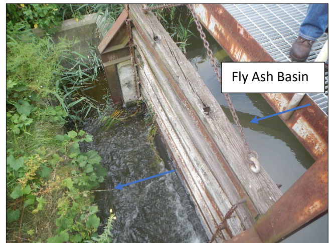
Photograph 60. DTE - Monroe Plant DSCN0146.JPG Description: The Box Weirs Discharge Control Structure uses a three stop log structure to control the elevation of the Fly Ash Basin.
