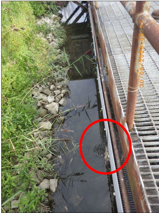
Photograph 119. DTE - Monroe Plant RIMG3196.JPG Description: View of additional leaks in the containment wall on the western side of the inactive bottom ash basin.
