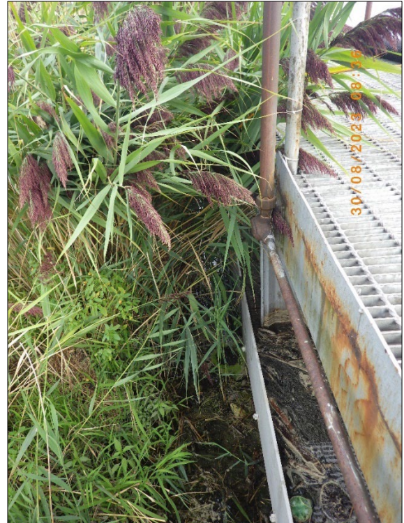
Photograph 116. DTE - Monroe Plant RIMG3193.JPG Description: View of standing water on the drainage canal side of the inactive bottom ash basin.
