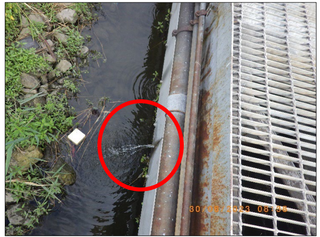
Photograph 121. DTE - Monroe Plant RIMG3198.JPG Description: View of additional leaks in the containment wall on the western side of the inactive bottom ash basin.
