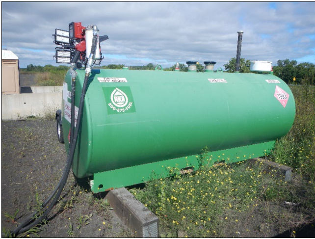
Photograph 77. DTE - Monroe Plant DSCN0163.JPG Description: General view of the double wall diesel tank at the CCR Vertical Extension equipment staging area.
