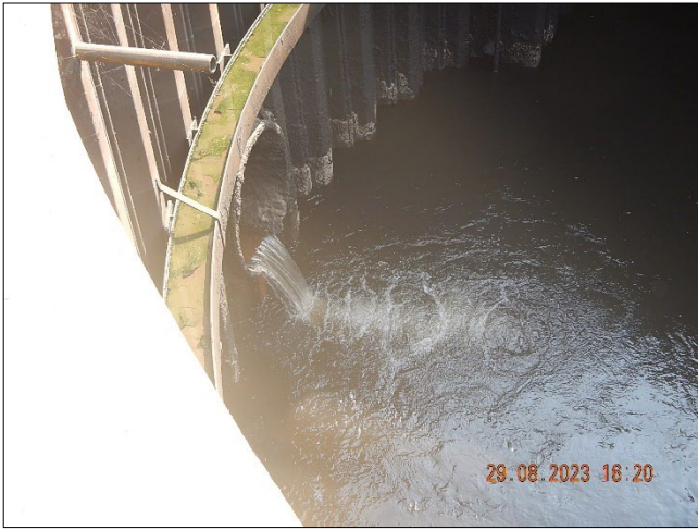
Photograph 53. DTE - Monroe Plant DSCN0139.JPG Description: General view of water entering SS#1.
