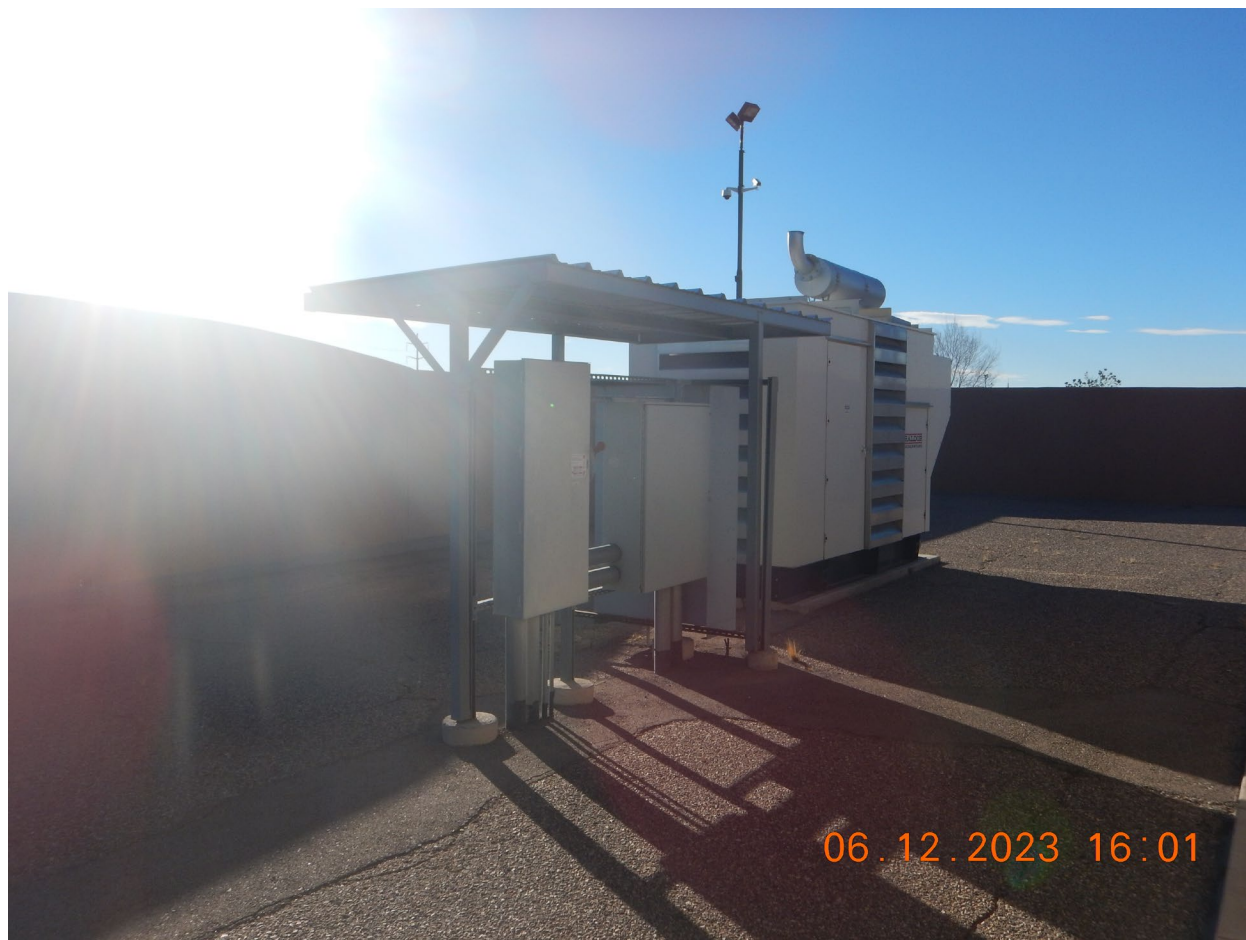
View of the onsite back-up generator. (DSCN2685). Photographed by D. Esparza
