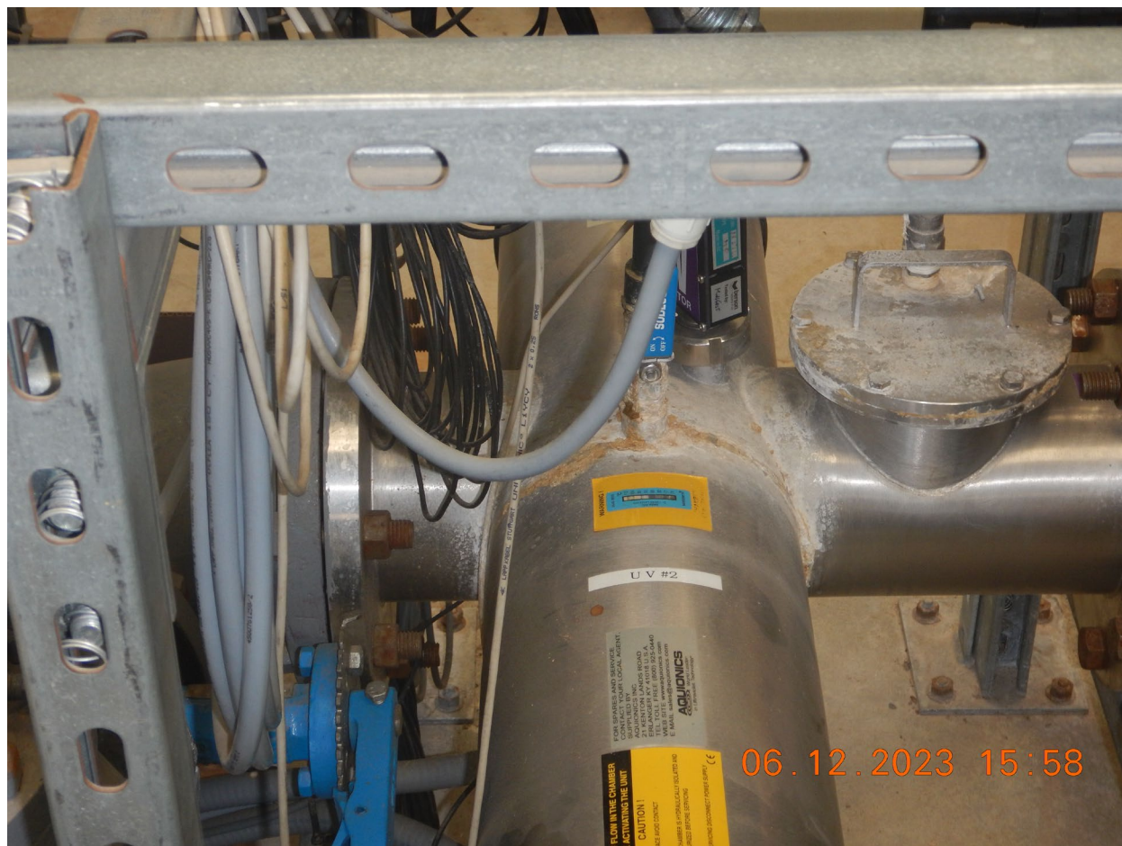
View of the one (1) of the ultraviolet (UV) disinfection treatment systems (UV-2) injection ports exhibiting corrosion. (DSCN2683). Photographed by D. Esparza
