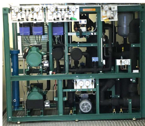
The pilot cooling plant
