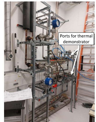
The cooling test rig
