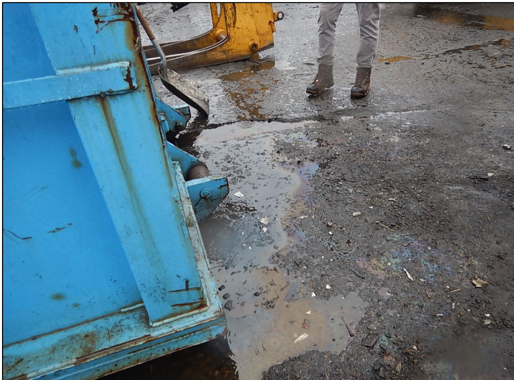
DSCN3934. View of petroleum sheen underneath the dumpster shown in DCN3930 and DCN3933 .
