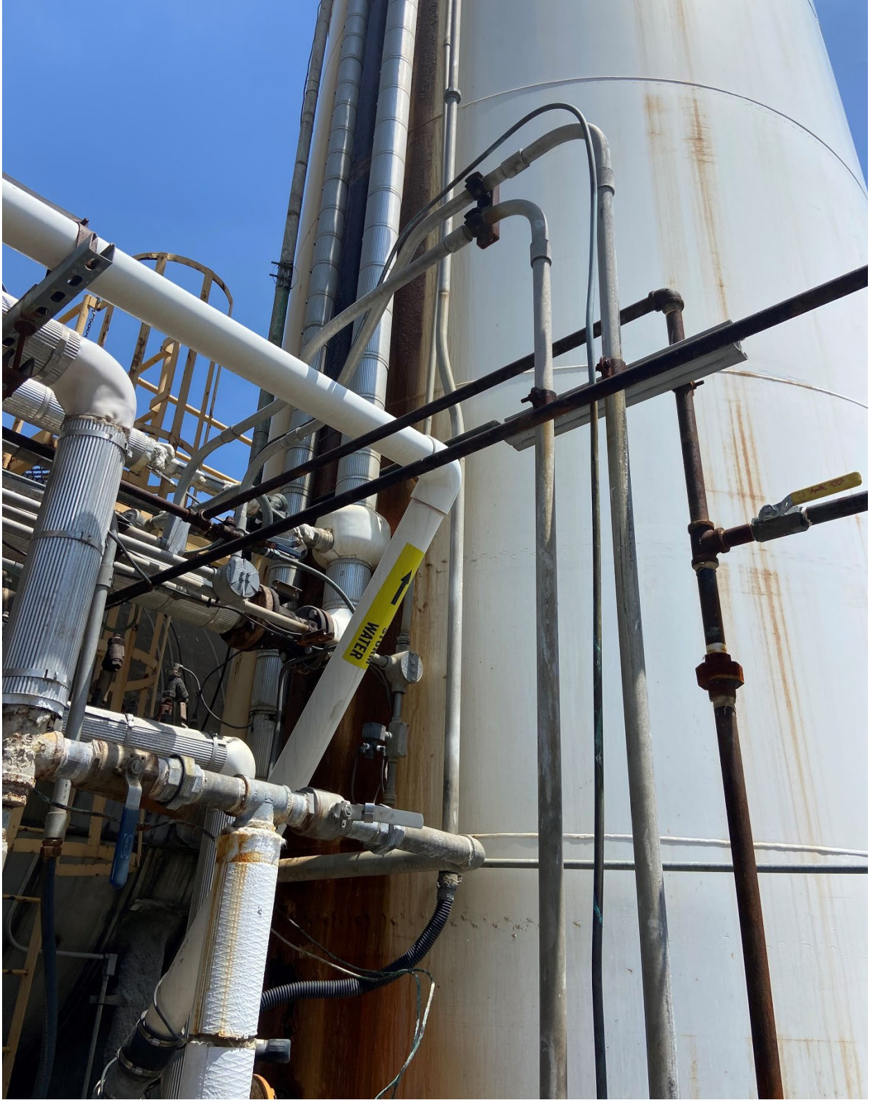
Figure 4: Corrosion along the side of Tank 75 in the Column Pad.
