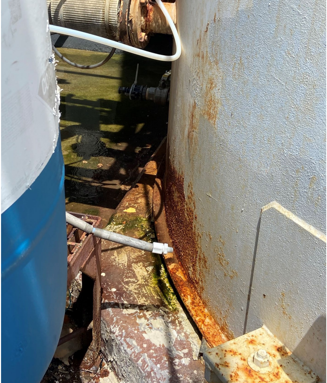
Figure 3: Corrosion and open valve on wastewater Tank 75 in the Column Pad.
