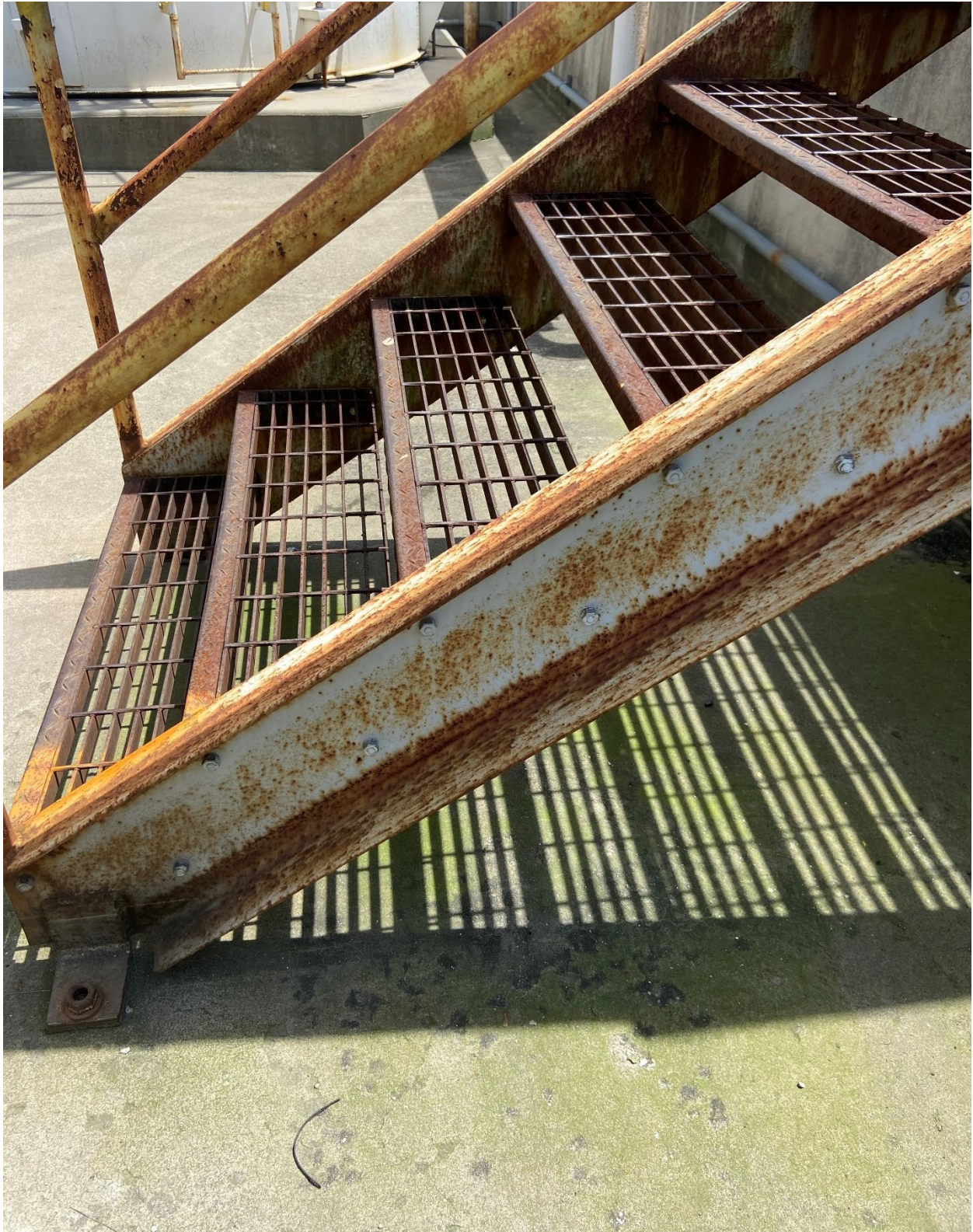
Figure 9: Pitting beneath the staircase leading into Tank Farm #4.
