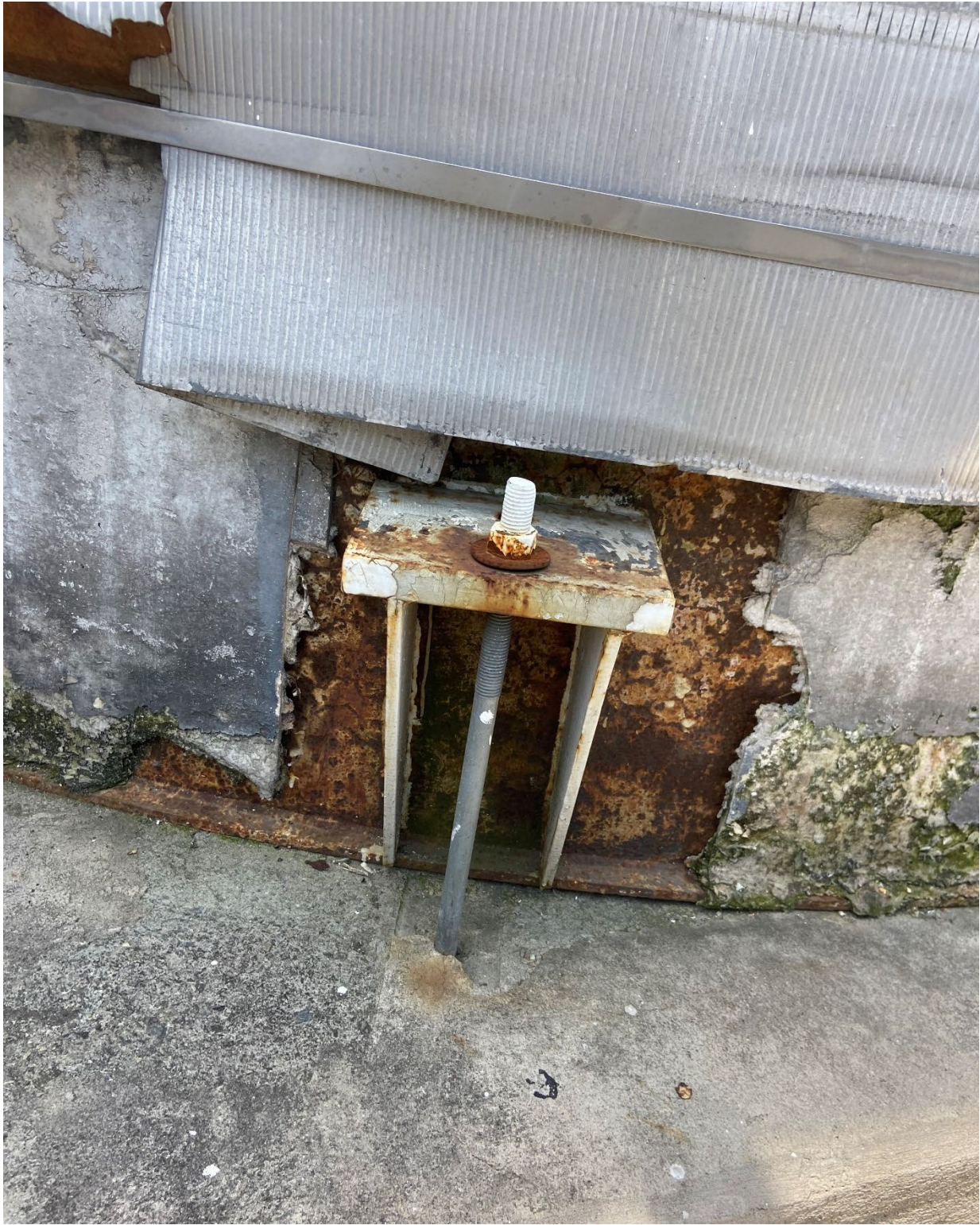
Figure 8: Pitting at the base of Tank 4403 in Tank Farm #4.
