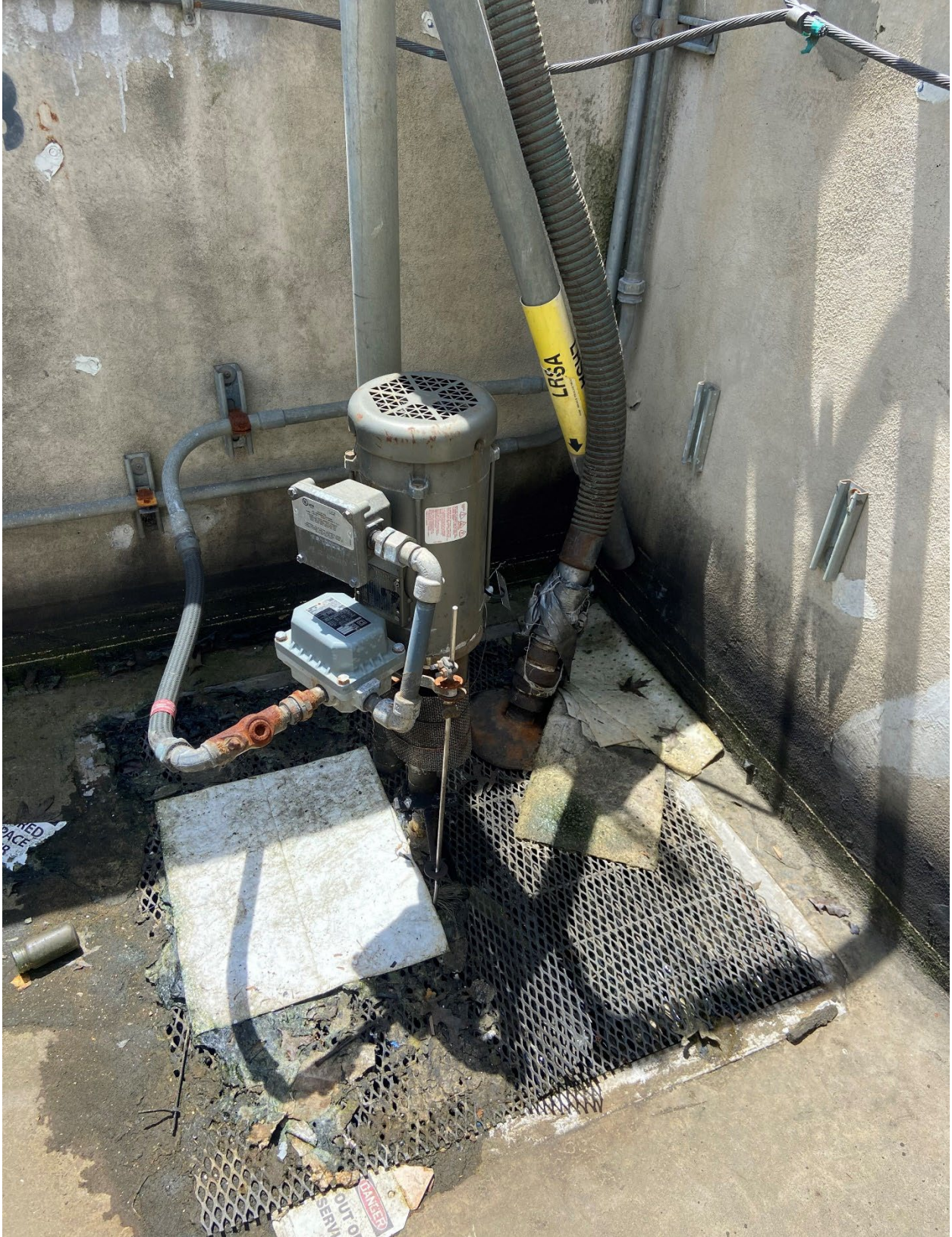
Figure 6: Soiled rags and open vial on its side on the floor inside Tank Farm #4.
