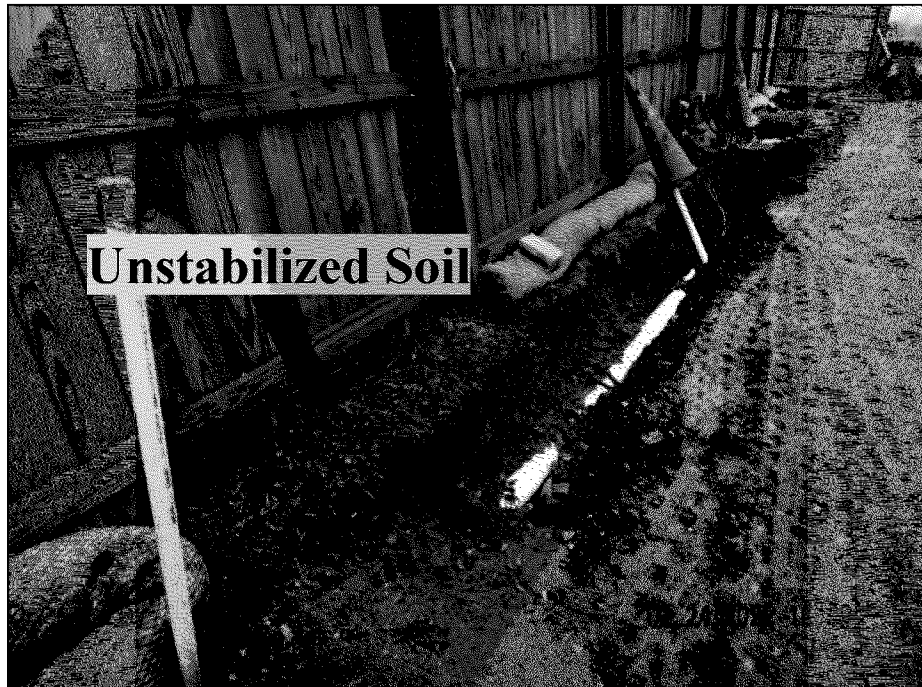
Photograph 39. (DSCN3951.JPG) View, facing northwest, of a location along the west perimeter that lacked perimeter controls. Unstabilized soil was adjacent to the perimeter.
