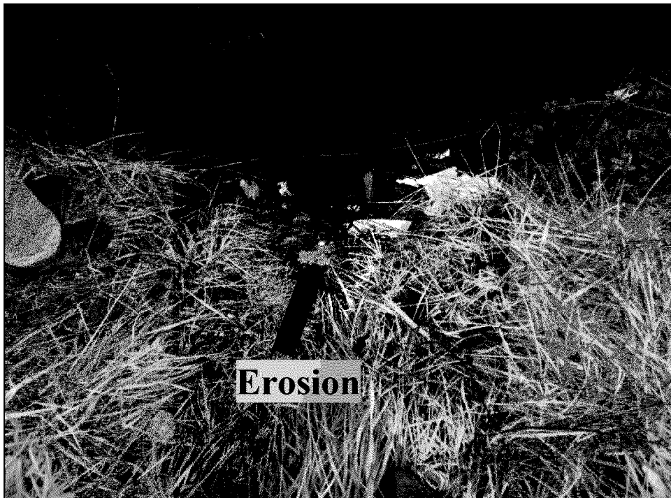
Photograph 60. (DSCN3971.JPG) View of erosion underneath the silt fence shown in Photograph 59.
