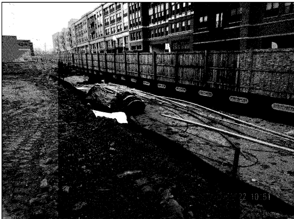
Photograph 24. (DSCN4053.JPG) View, facing south, of a silt fence along the west perimeter.
