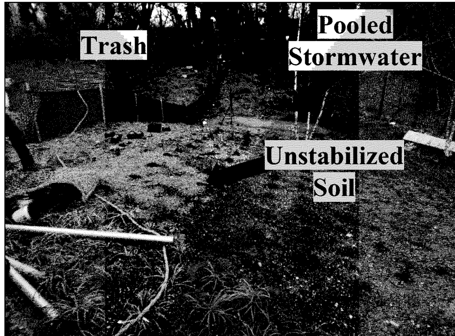
Photograph 32. (DSCN3927.JPG) View, facing east, of the sediment-laden stormwater pooled at the southeast corner of the site. Note the unstabilized soil and trash upgradient of the pooled stormwater.
