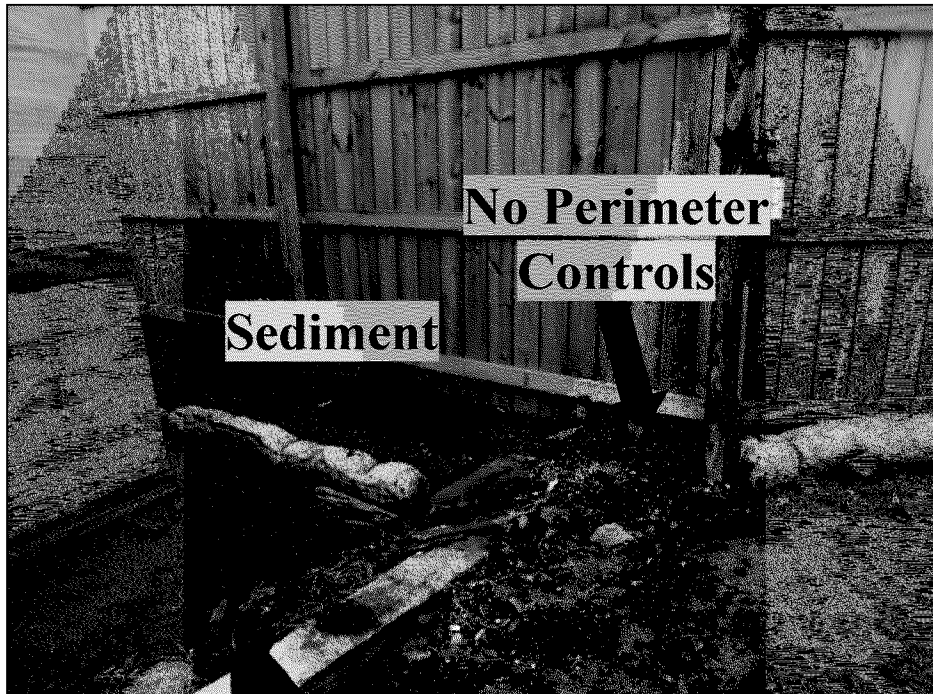
Photograph 37. (DSCN4055.JPG) View, facing west, of the west perimeter near the southwest corner that lacked perimeter controls. Note the sediment that traveled off-site.
