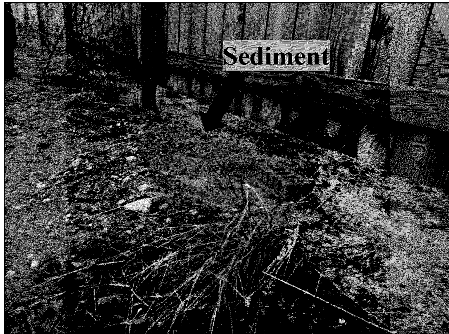
Photograph 49. (DSCN4022.JPG) View, facing south, of the mid-west perimeter downgradient of the pooled stormwater in the north area of the site shown in Photographs 46 through 48. Note the sediment. The EPA Inspection Team did not observe perimeter controls at this location.
