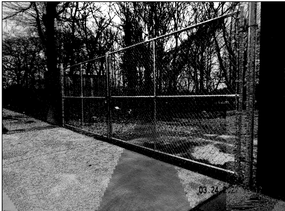
Photograph 28. (DSCN4068.JPG) View, facing northeast, of the stabilized construction entrance at the northwest corner of the site. Permit-required elements were not posted on a sign at this location.
