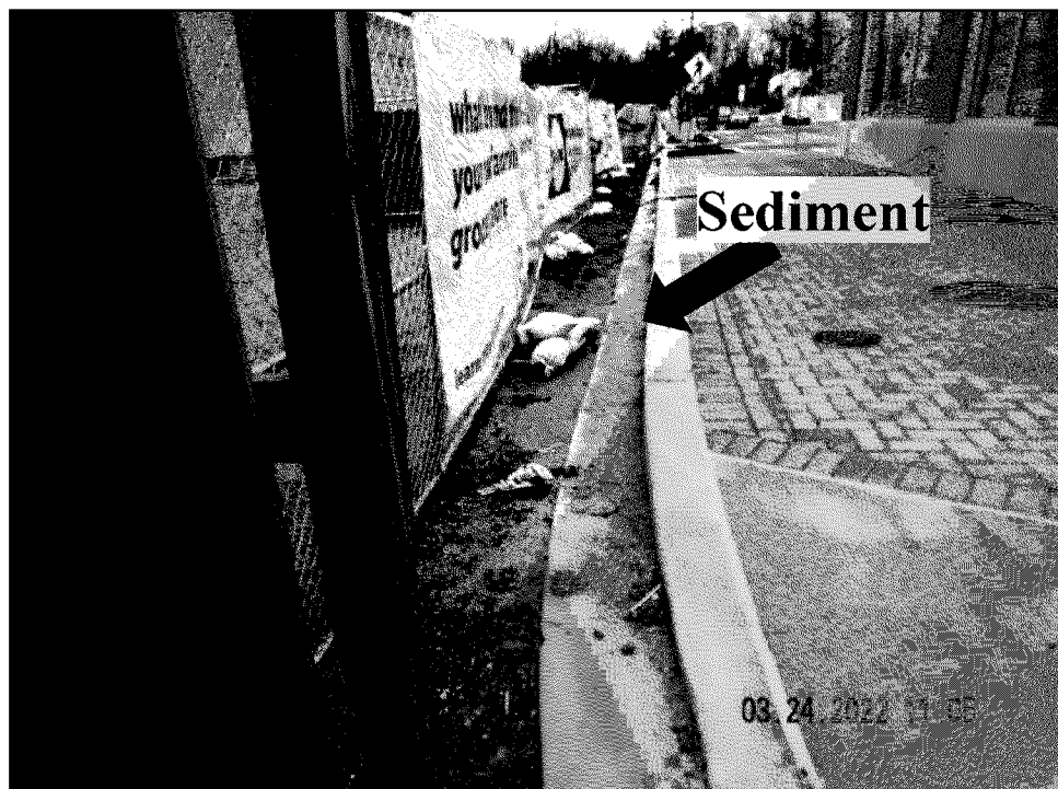
Photograph 54. (DSCN4059.JPG) View, facing east, of the south perimeter that lacked perimeter controls. Note the sediment transported offsite. Photograph was taken offsite.
