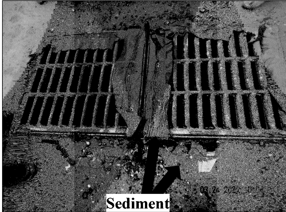
Photograph 1. (DSCN3938.JPG) View of stormwater inlets in the south area of the site. Note the sediment adjacent to the stormwater inlets.
