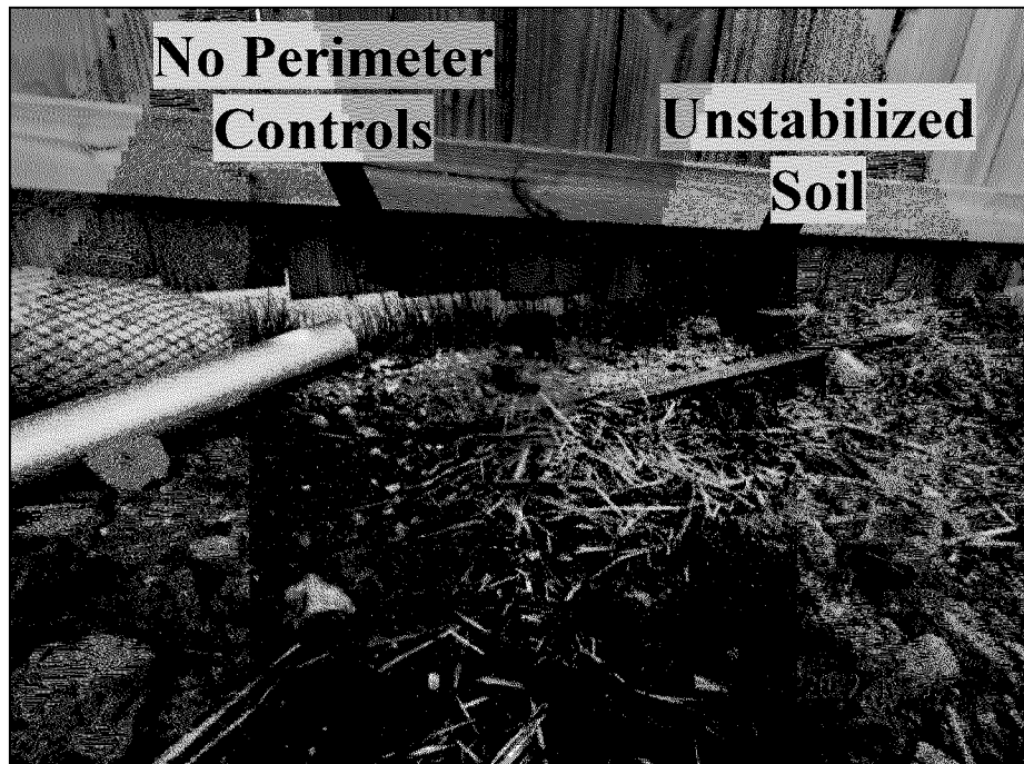
Photograph 41. (DSCN3953.JPG) View, facing west, of a location along the west perimeter that lacked perimeter controls as shown in Photograph 40. The EPA Inspection Team observed unstabilized soil adjacent to the perimeter.
