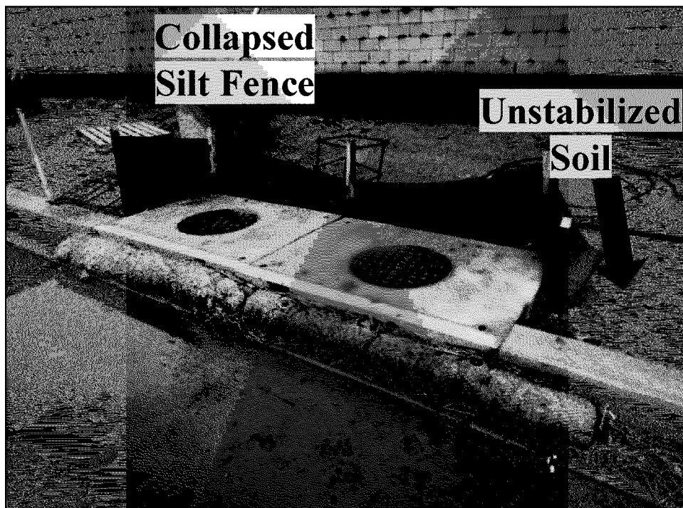
Photograph 6. (DSCN3946.JPG) View, facing north, of curb inlets in the south area of the site. The silt fence had collapsed and the surrounding soil was unstabilized.
