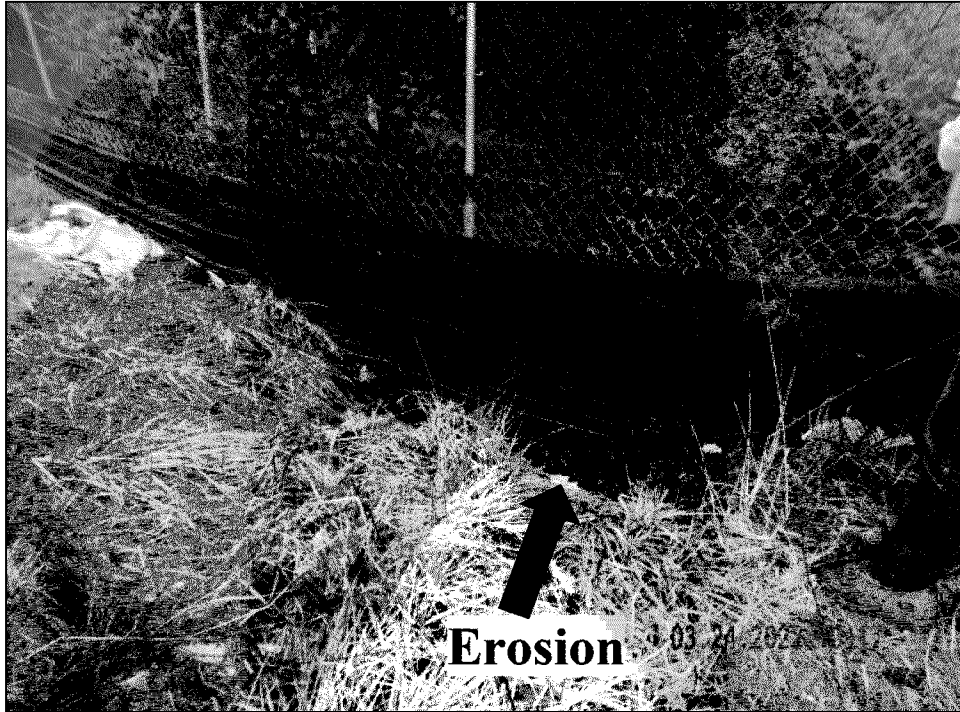
Photograph 59. (DSCN3969.JPG) View, facing east, of erosion by the mid-east perimeter. The silt fence was undercut by the erosion.
