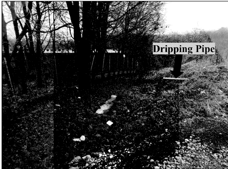
Photograph 75. (DSCN4006.JPG) View, facing east, of an unlabeled dripping pipe that ran underneath the stabilized construction entrance at the northeast corner of the site.
