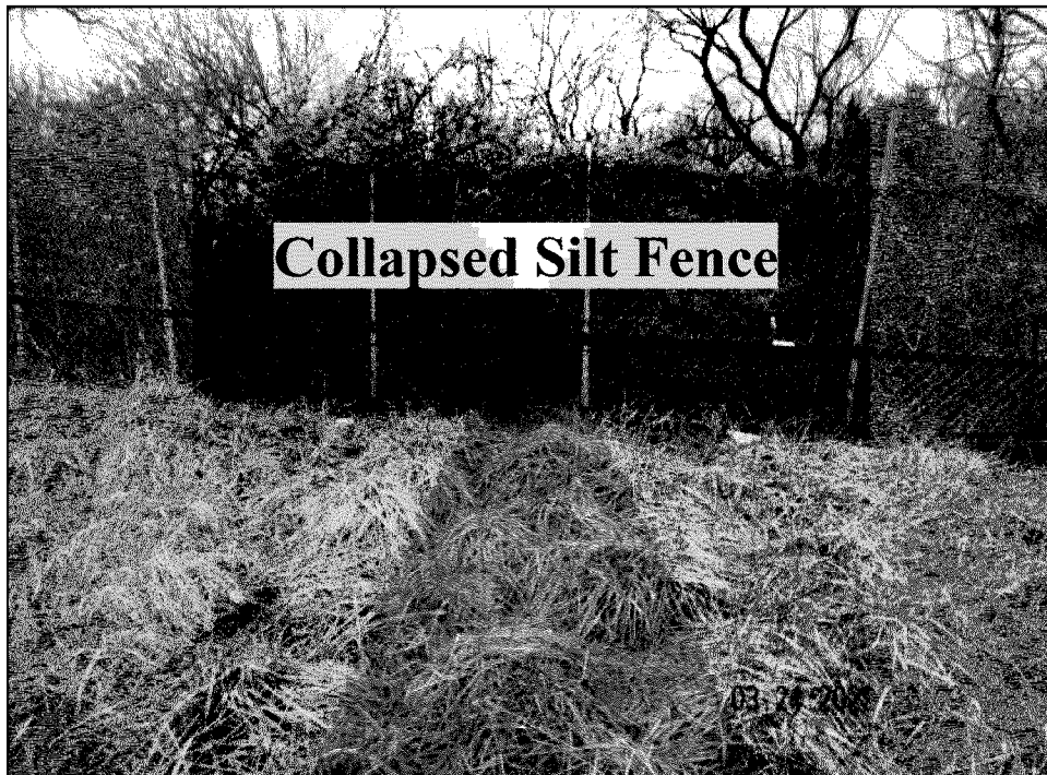
Photograph 62. (DSCN3977.JPG) View, facing east, of collapsed silt fencing along the east perimeter.
