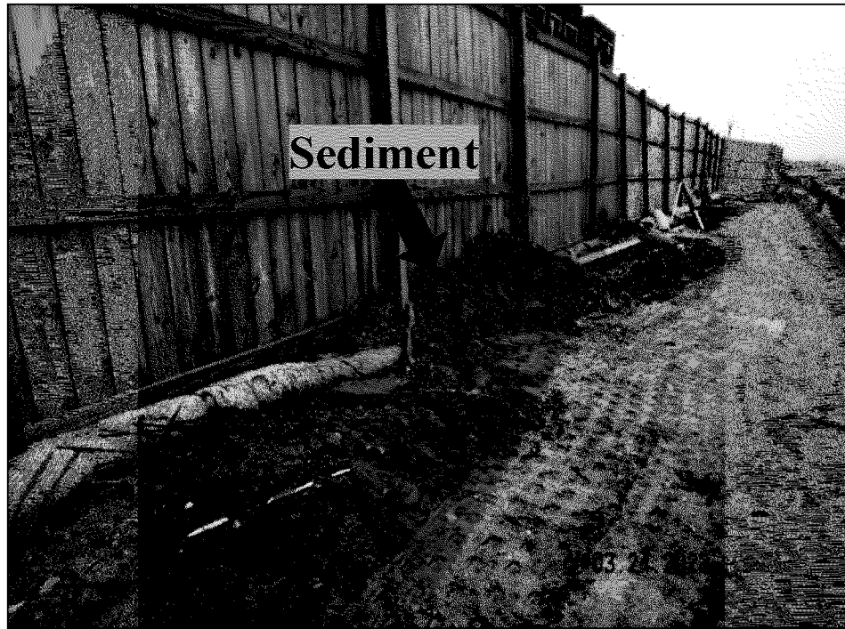
Photograph 55. (DSCN3950.JPG) View, facing northwest, of the filter sock along the west perimeter that had accumulated sediment above one-half the height of the filter sock.
