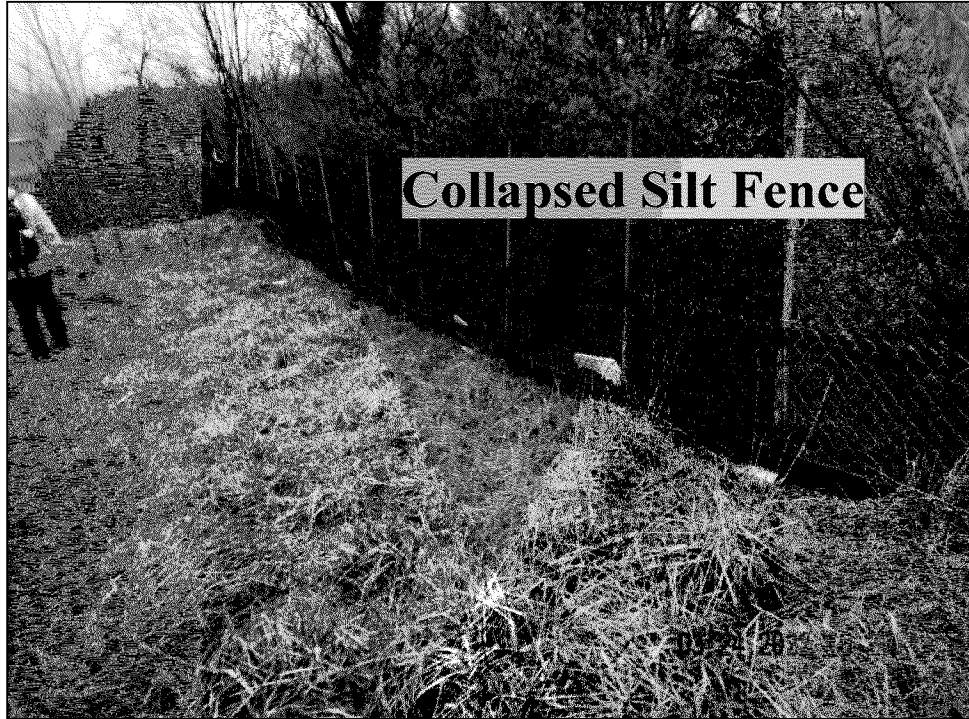
Photograph 63. (DSCN3980.JPG) View, facing northeast, of collapsed silt fencing along the east perimeter as shown in Photograph 62.
