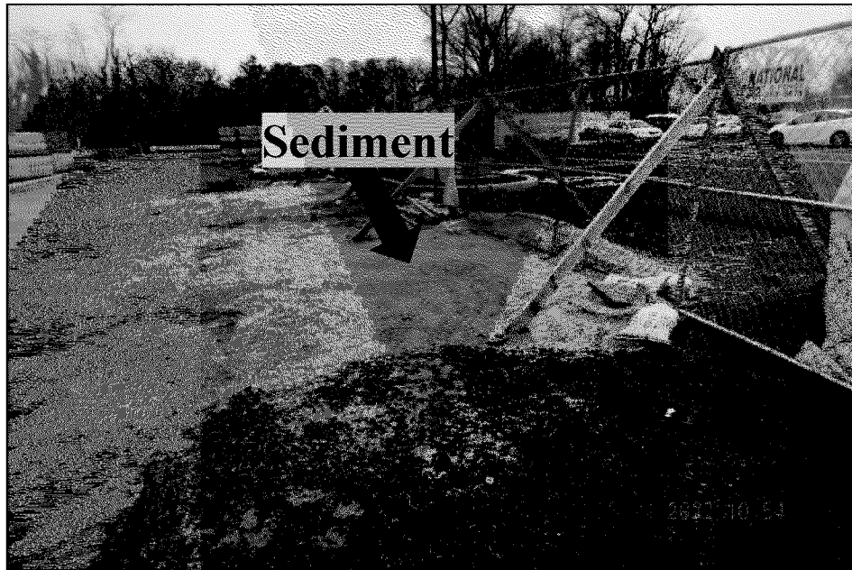
Photograph 53. (DSCN4058.JPG) View, facing east, of the south perimeter that lacked perimeter controls. Note the sediment that led offsite.
