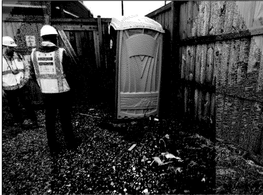
Photograph 51. (DSCN4019.JPG) View, facing south, of a portable toilet located adjacent to the mid-west perimeter in the north area of the site. The portable toilet did not have a containment pan or have any other observable secondary containment.
