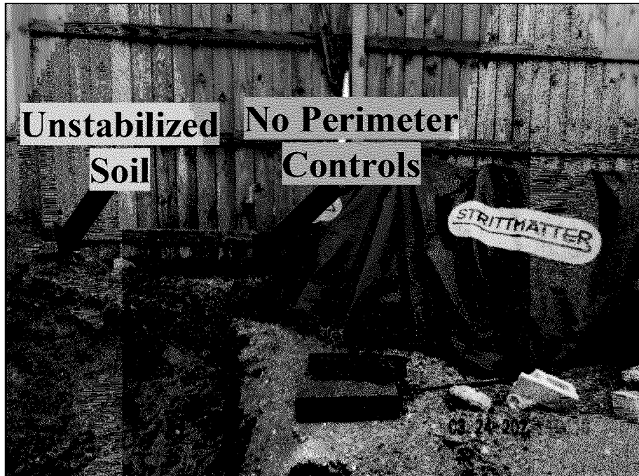
Photograph 43. (DSCN3954.JPG) View, facing west, of a location along the west perimeter that lacked perimeter controls. The EPA Inspection Team observed unstabilized soil adjacent to the location.
