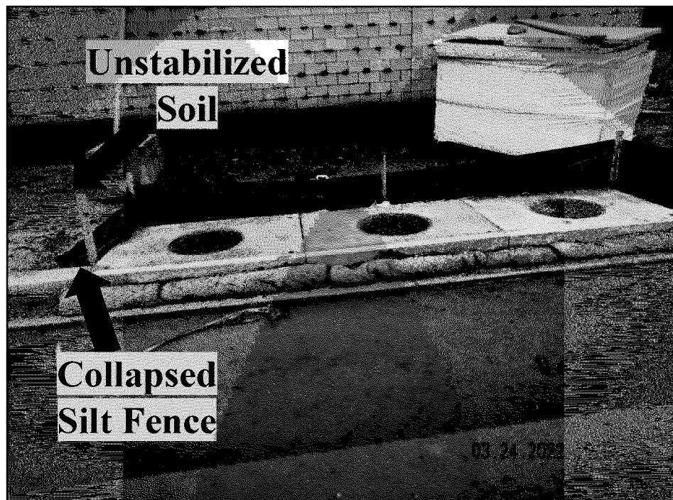
Photograph 4. (DSCN3942.JPG) View, facing north, of curb inlets in the south area of the site. Note that the silt fence was collapsed, and surrounding soil was unstabilized.
