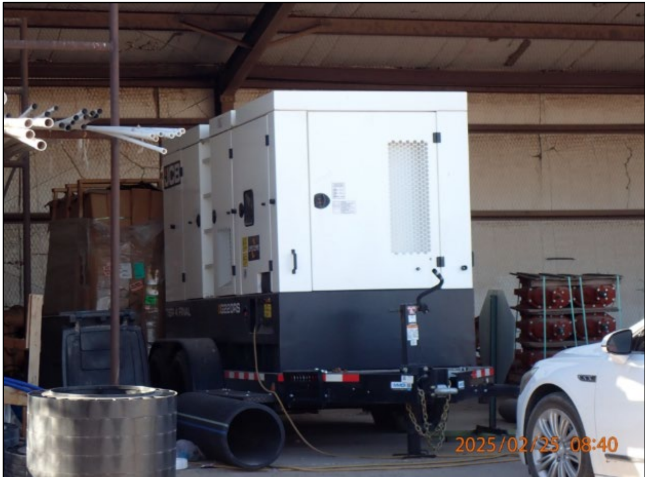
Photograph 12. 02/25/2025 08:40 P2250291.JPG Description: Portable generator located at Well #1.
