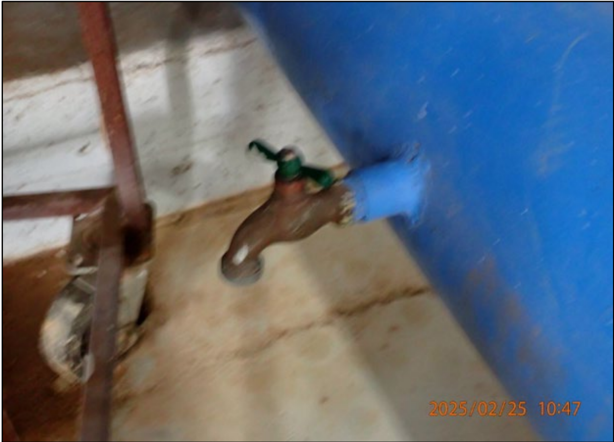
Photograph 25. 02/25/2025 10:47 P2250383.JPG Description: Threaded sample tap on the Well #17 discharge piping.
