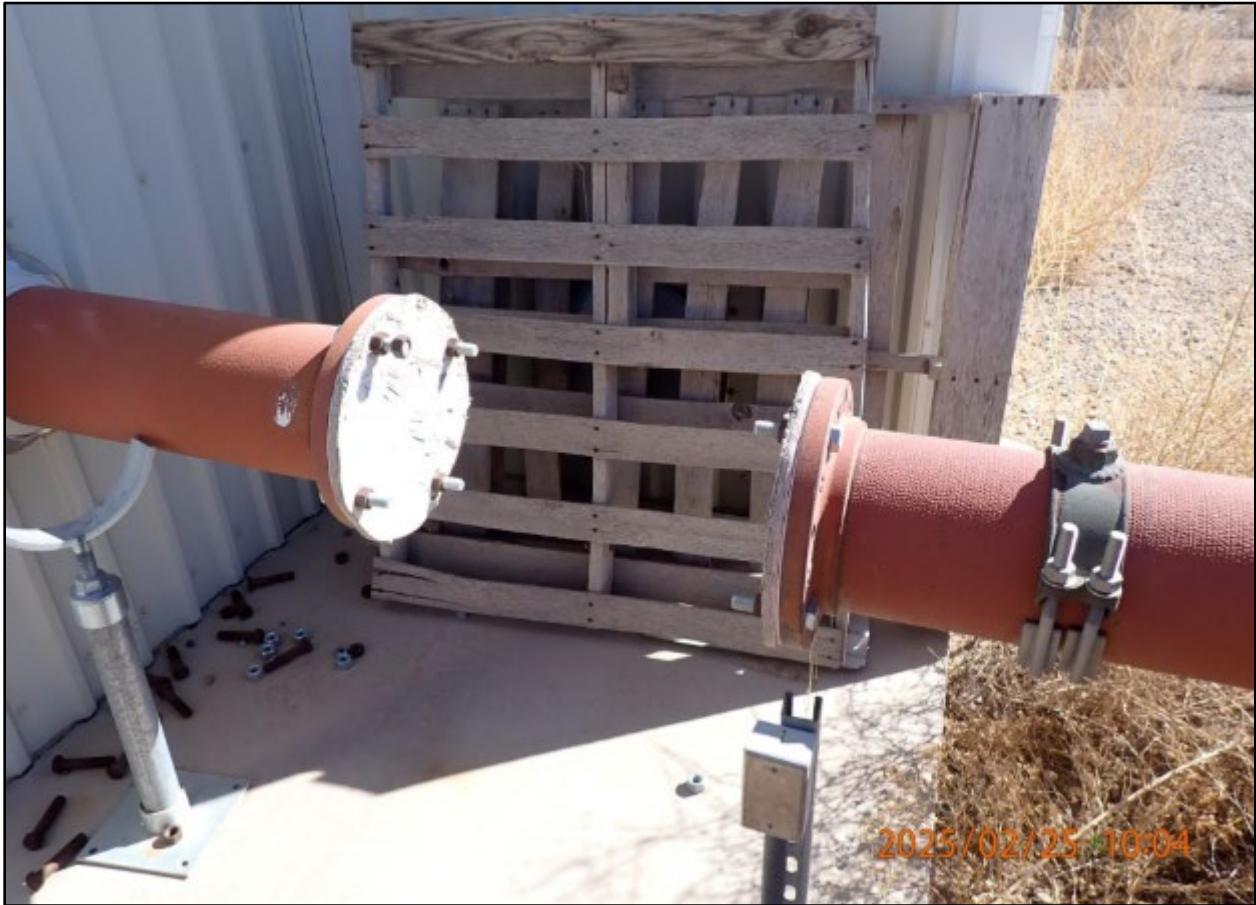
Photograph 2. 02/25/2025 10:04 P2250339.JPG Description: Inactive Well #18 severed discharge line.
