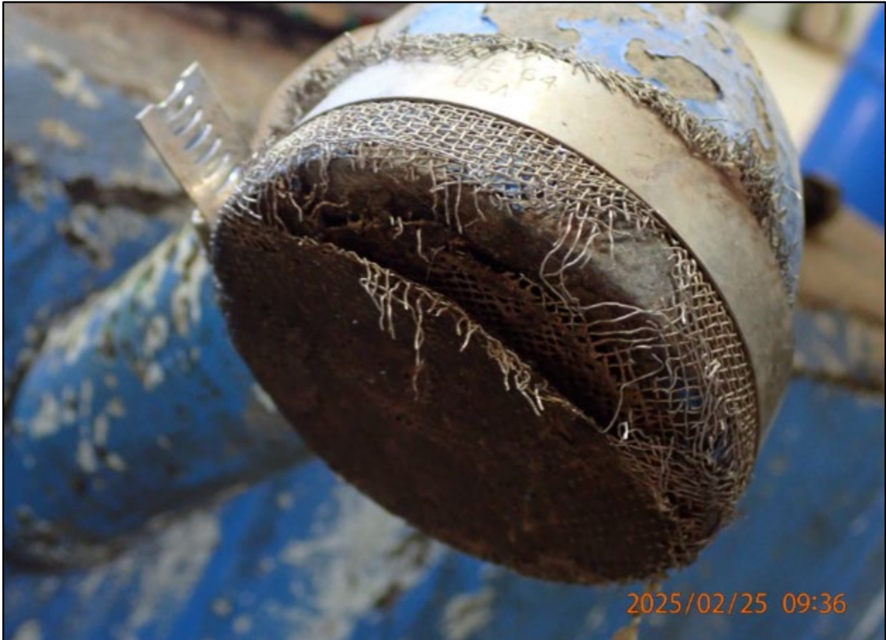
Photograph 20. 02/25/2025 09:36 P2250331.JPG Description: Well #2 vent screen with torn mesh.
