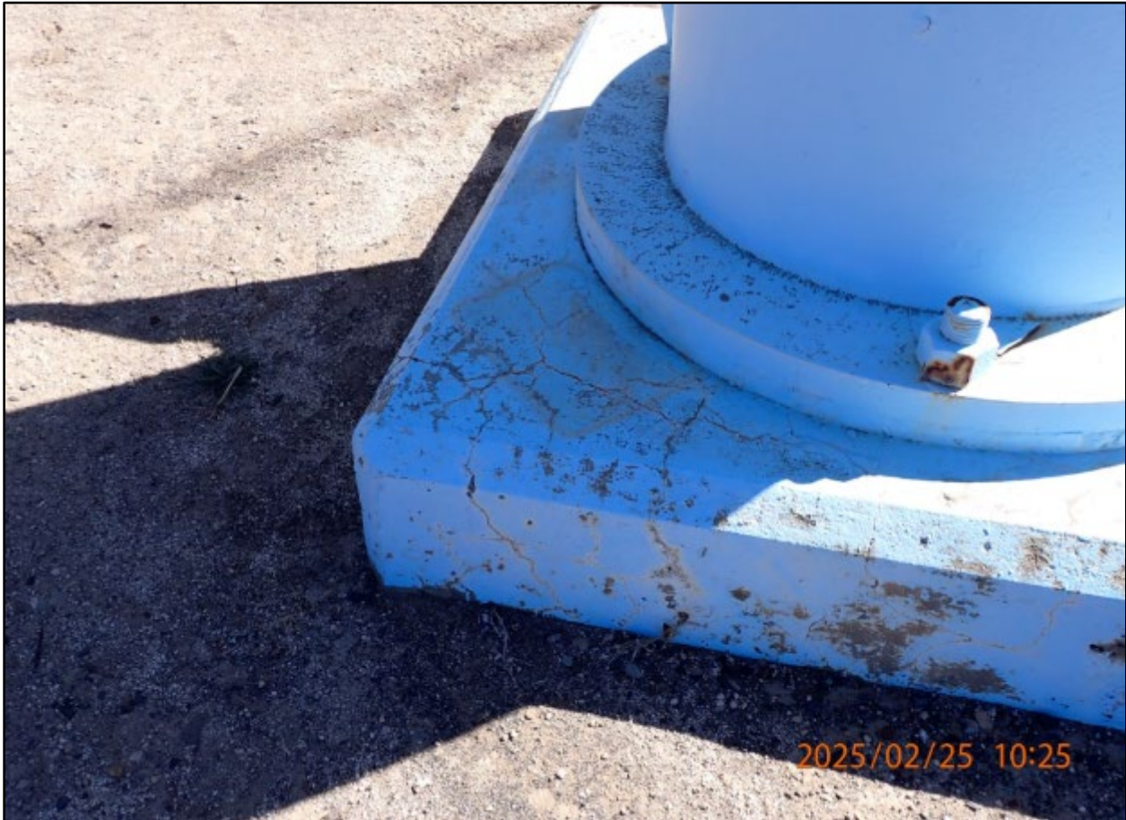
Photograph 30. 02/25/2025 10:25 P2250369.JPG Description: Cracking foundation of the Well #11 Tower.
