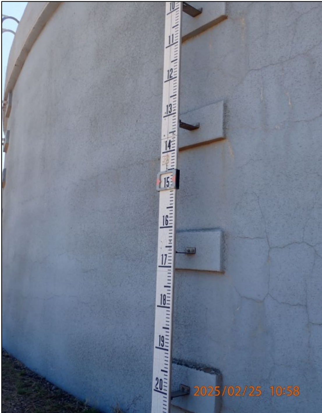
Photograph 26. 02/25/2025 10:58 P2250397.JPG Description: Minor cracking of 3-MG Storage Tank.
