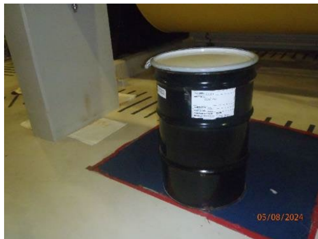
Picture 15 – Main Turbine Oil Tank used oil container
