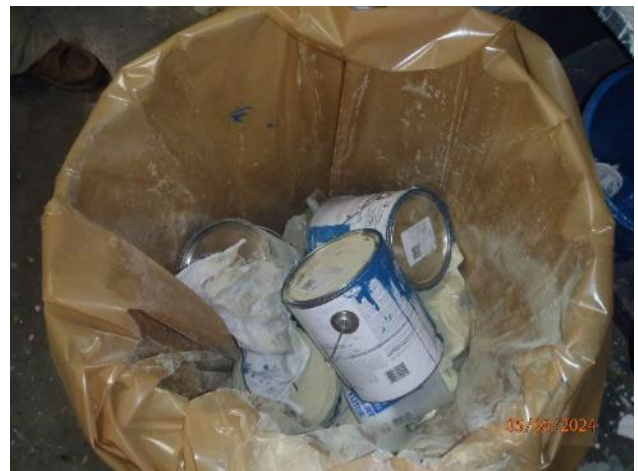
Picture 11 – Painter Cleanup SAA discarded epoxy paint cans in trash can
