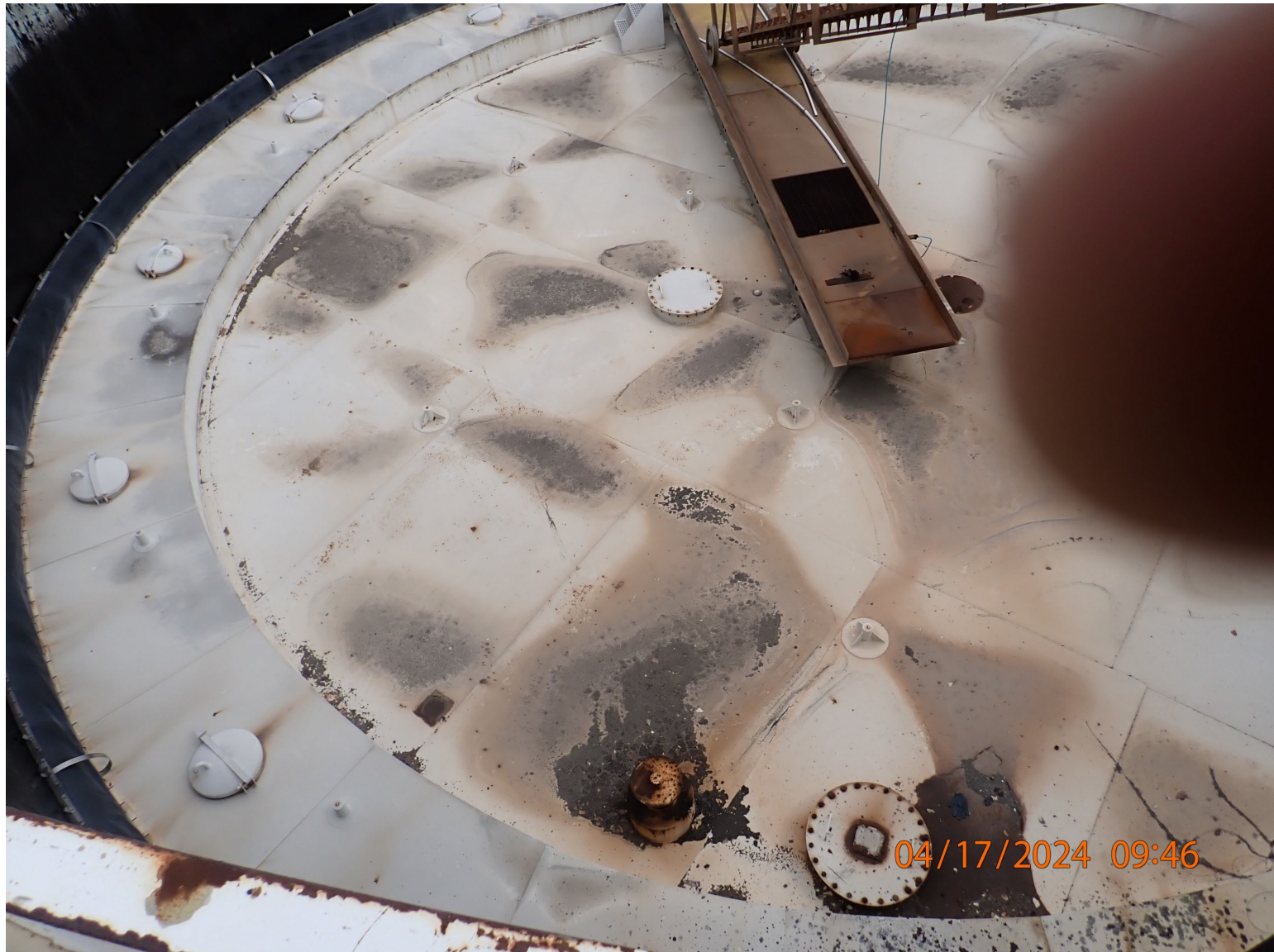
Photo 010: Equalization Tank T-302 Pop-up vent - 4/17/2024 09:46 P4170010.jpg
