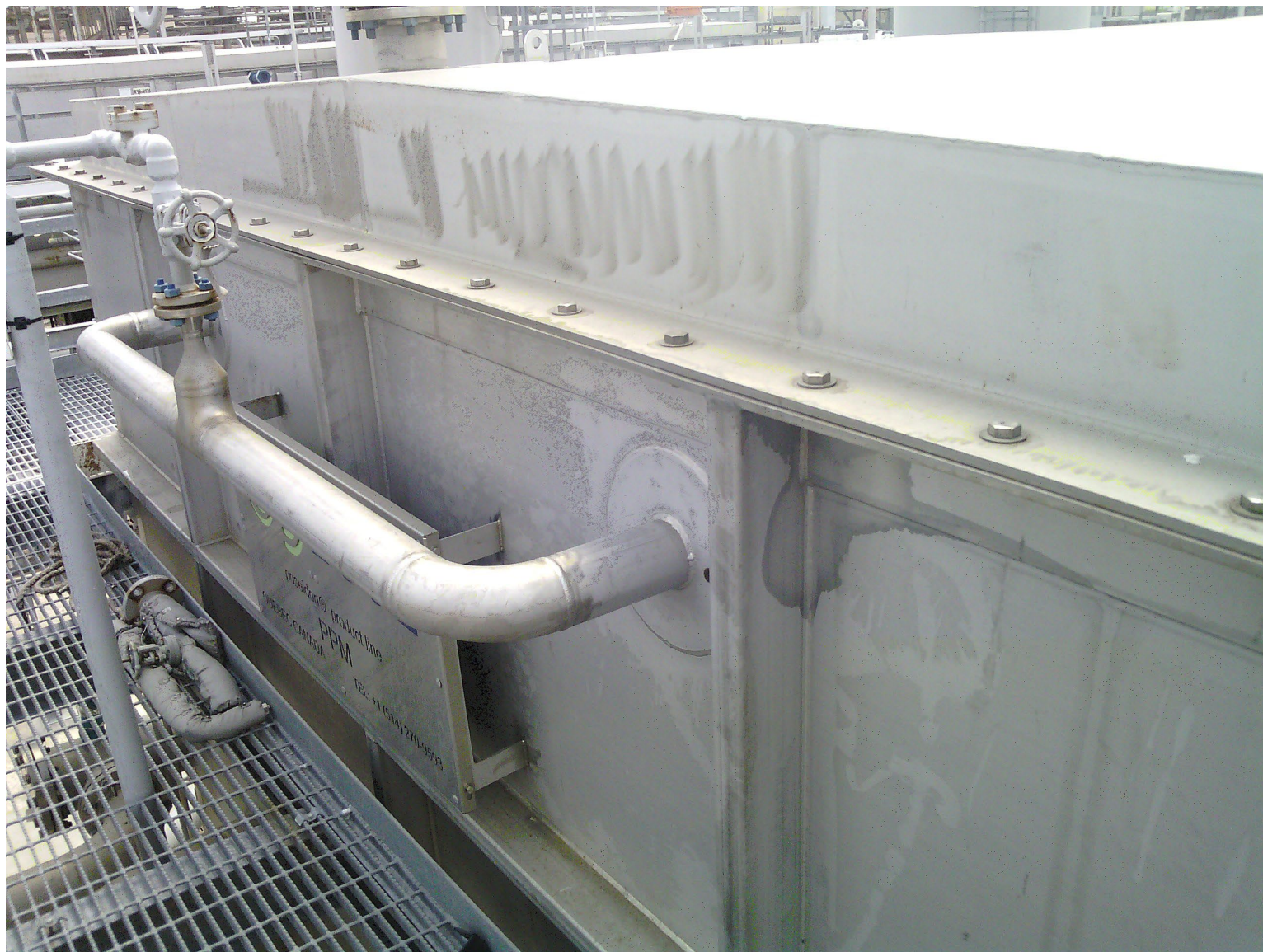
Photo 054: DNF TN-80010 flange - 4/18/2024 12:11 FLIR0054.jpg
