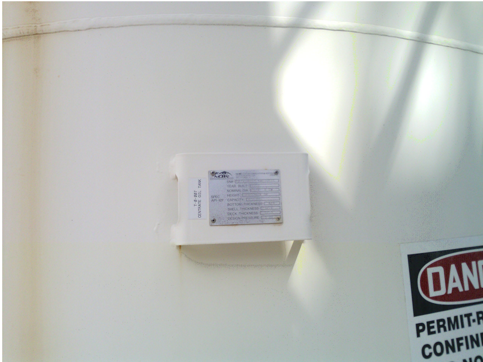
Photo 033: Centrate oil tank T-0-007 nameplate - 4/18/2024 09:58 FLIR0033.jpg
