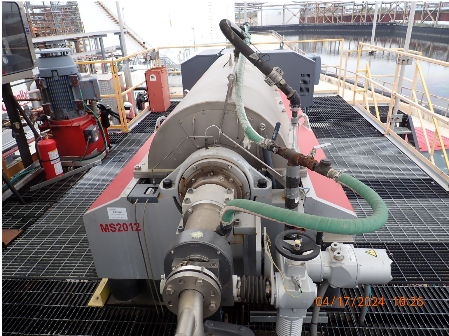
Photo 015: Clean Harbors sludge removal centrifuge 4/17/2024 10:26 P4170015.jpg
