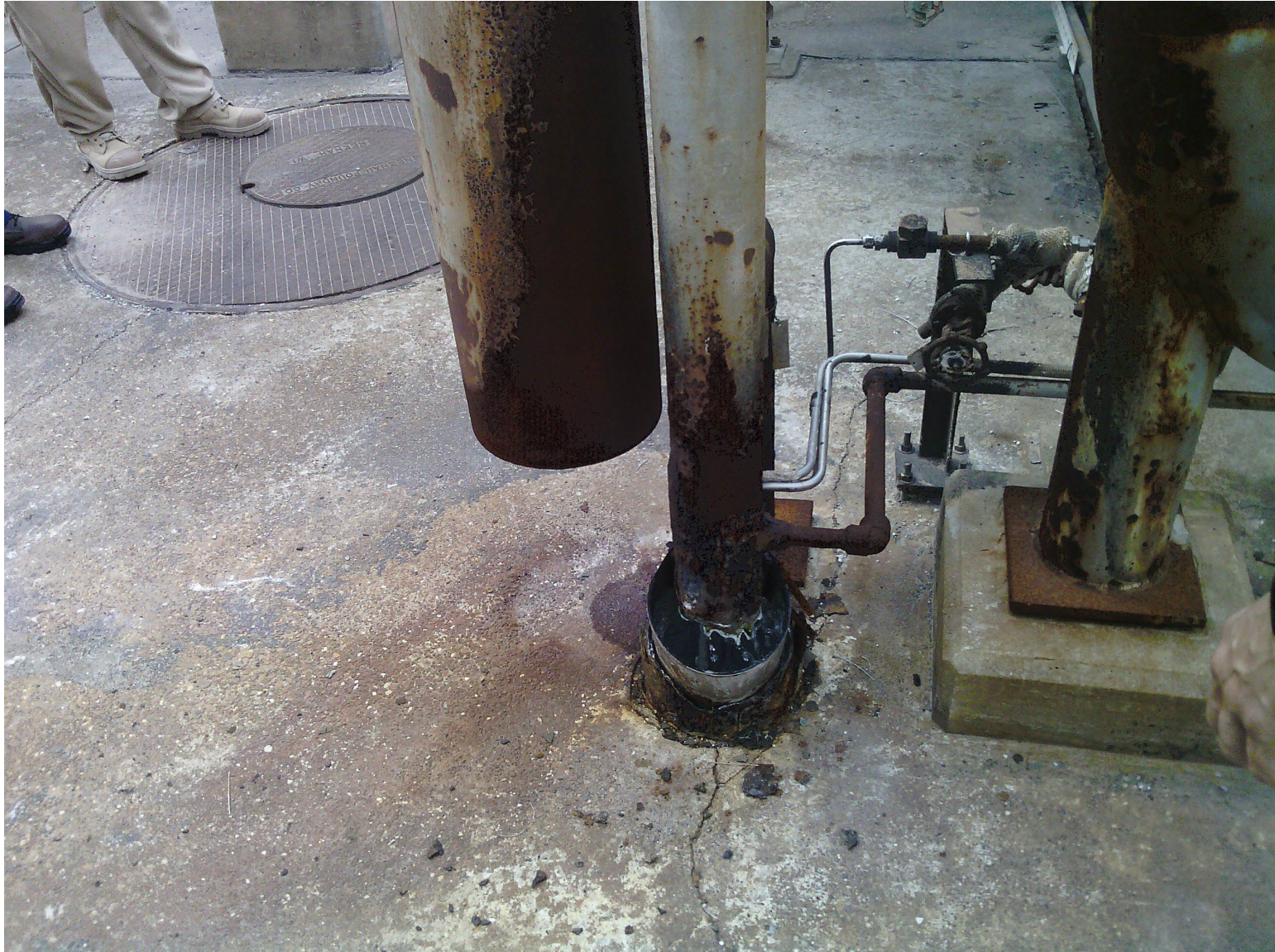
Photo 036: IGF #2 water seal drain - 4/18/2024 10:09 FLIR0036.jpg
