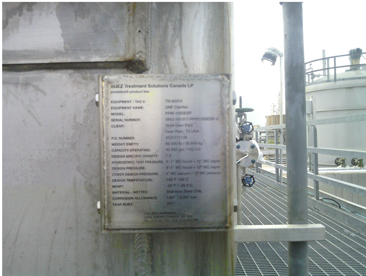
Photo 055: DNF TN-80010 nameplate - 4/18/2024 12:11 FLIR0055.jpg
