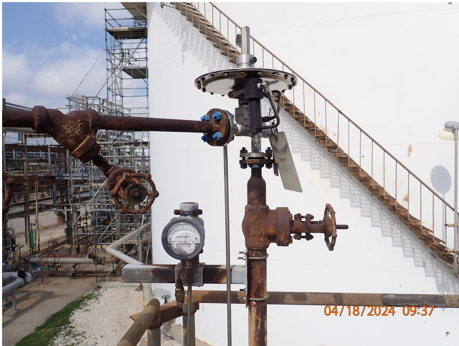
Photo 023: CPI#2 nitrogen blanket pressure gauge 4/18/2024 09:37 P4180023.jpg
