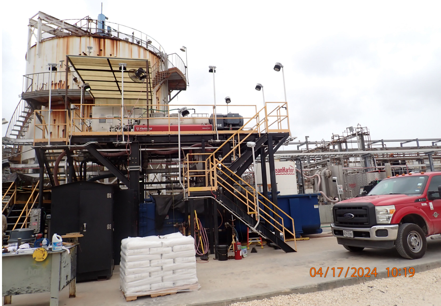
Photo 014: Clean Harbors sludge removal centrifuge 4/17/2024 10:19 P4170014.jpg
