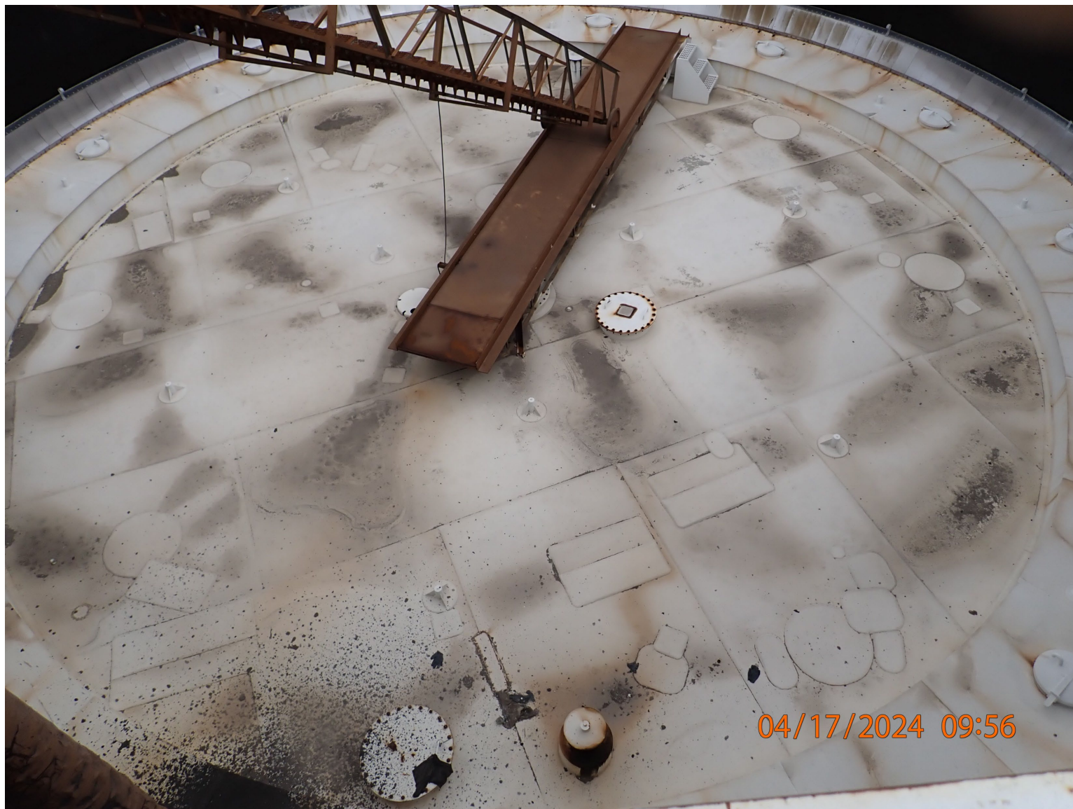
Photo 011: Diversion Tank T-301 Pop-up vent - 4/17/2024 09:56 P4170011
