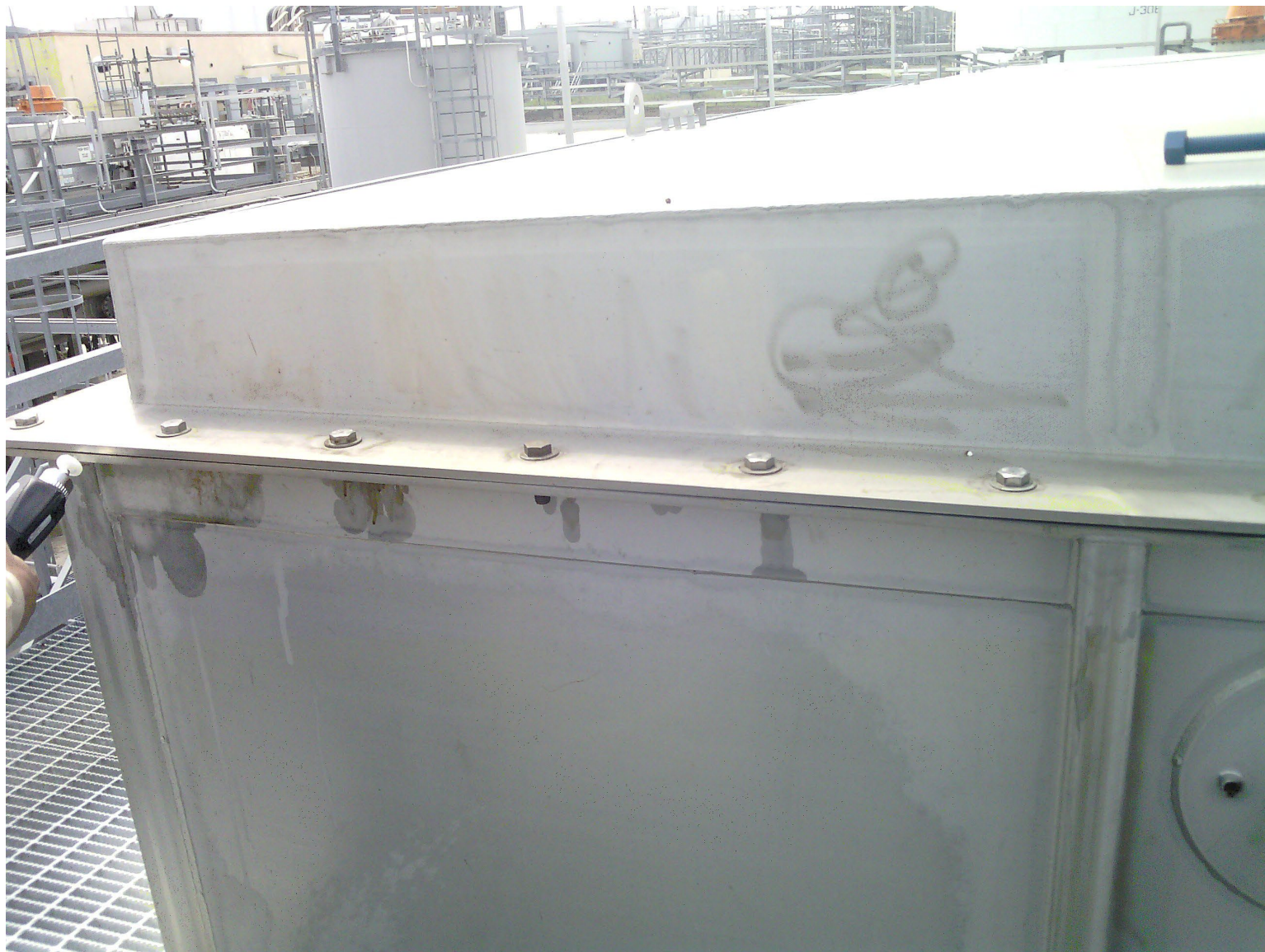
Photo 053: DNF TN-80010 flange - 4/18/2024 12:11 FLIR0053.jpg
