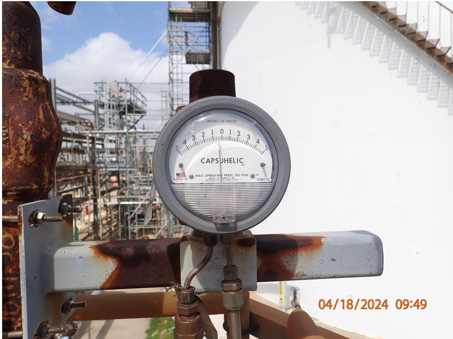
Photo 026: CPI #1 nitrogen blanket pressure gauge - 4/18/2024 09:49 P4180026.jpg
