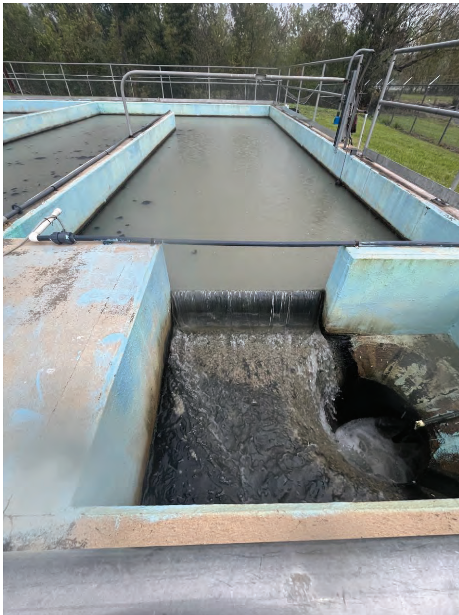
Woodland Treatment Chlorine Basin with visible solids discharging
