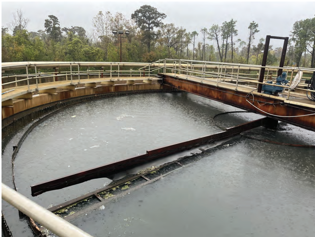
Woodland Treatment Clarifier with broken arm
