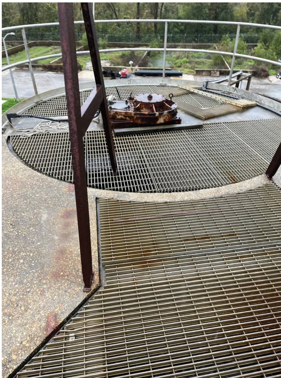
Woodland Treatment Grit Chamber
