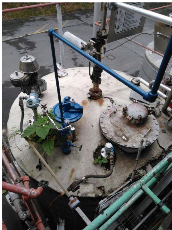
Photo 7: Bldg. 267 tank 1829: Vegetation observed growing on top of the tank.
