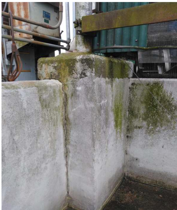
Photo 14: Building 285 HWDU-30. Crack in the wall of the secondary containment at the time of the inspection.
