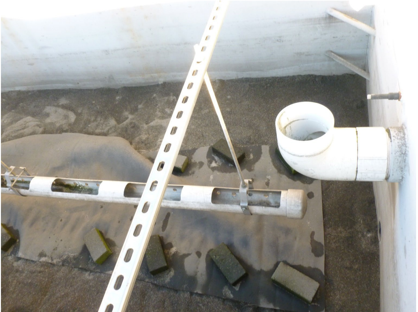
Photo 8 / P1010232 – Interior of Filtration System, effluent side
