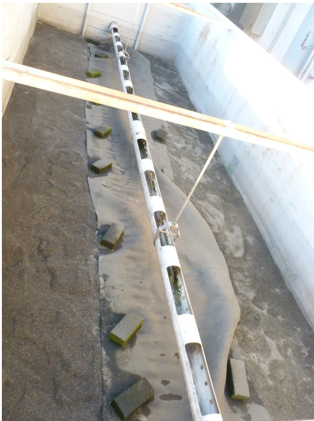
Photo 7 / P1010233 – Interior of Filtration System with Diffusion Pipe
