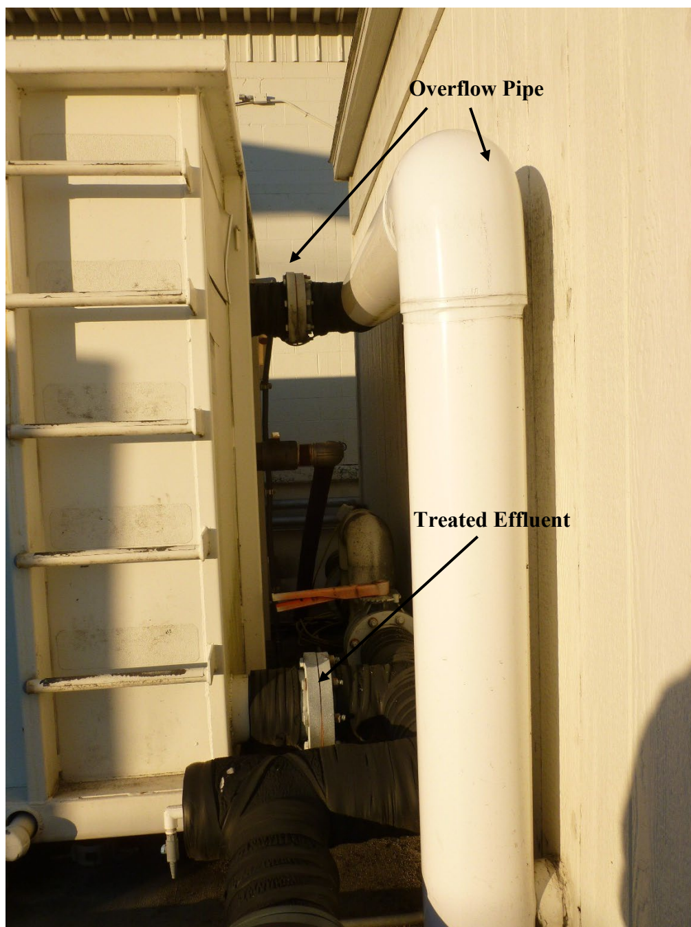
Photo 9 / P1010234 – Effluent Side of Filtration System
