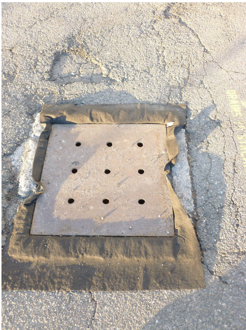
Photo 3 / P1010237 – Catch Basin with Filter
