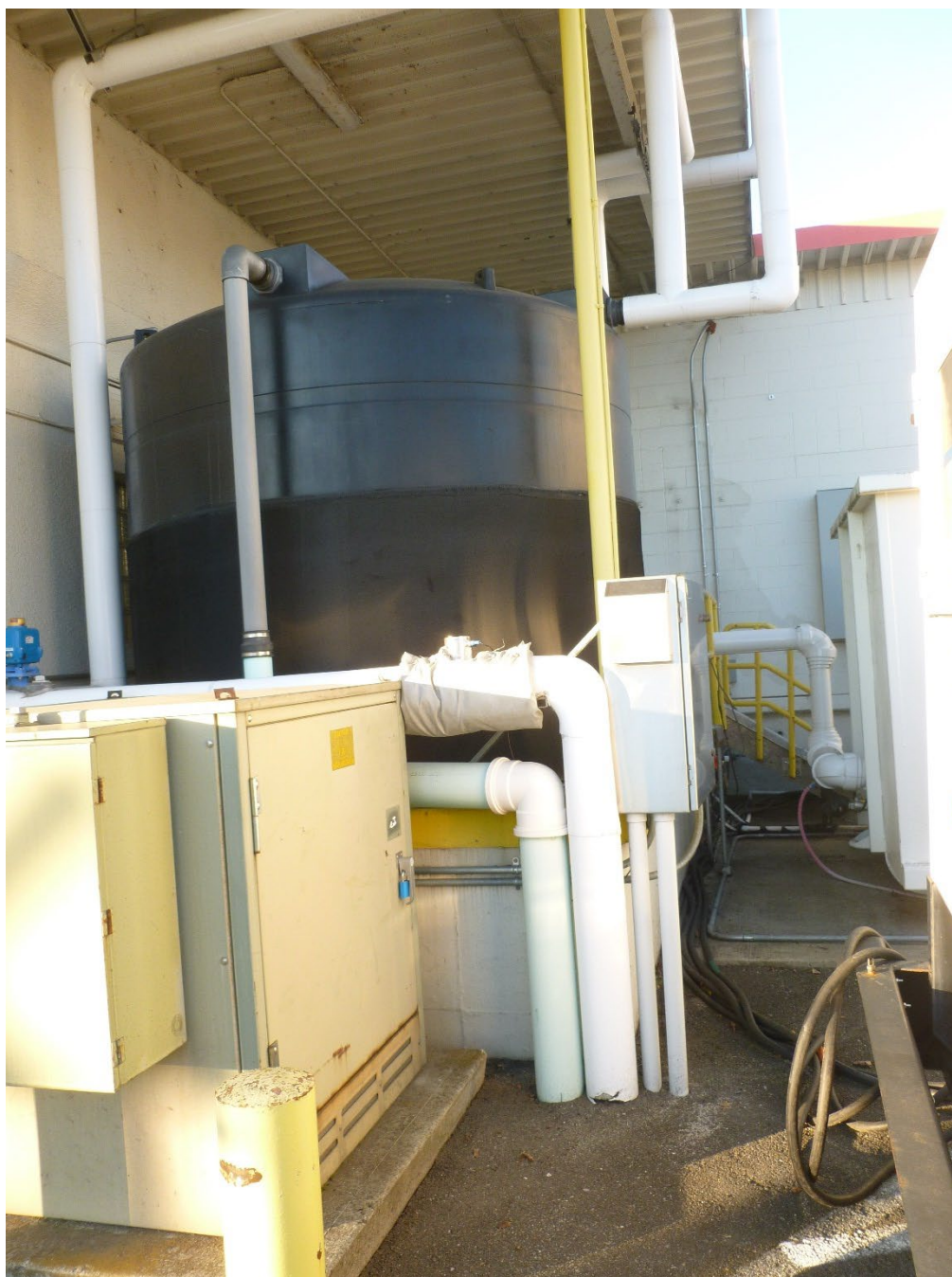
Photo 5 / P1010230 – 3,000 Gallon Stormwater Tank
