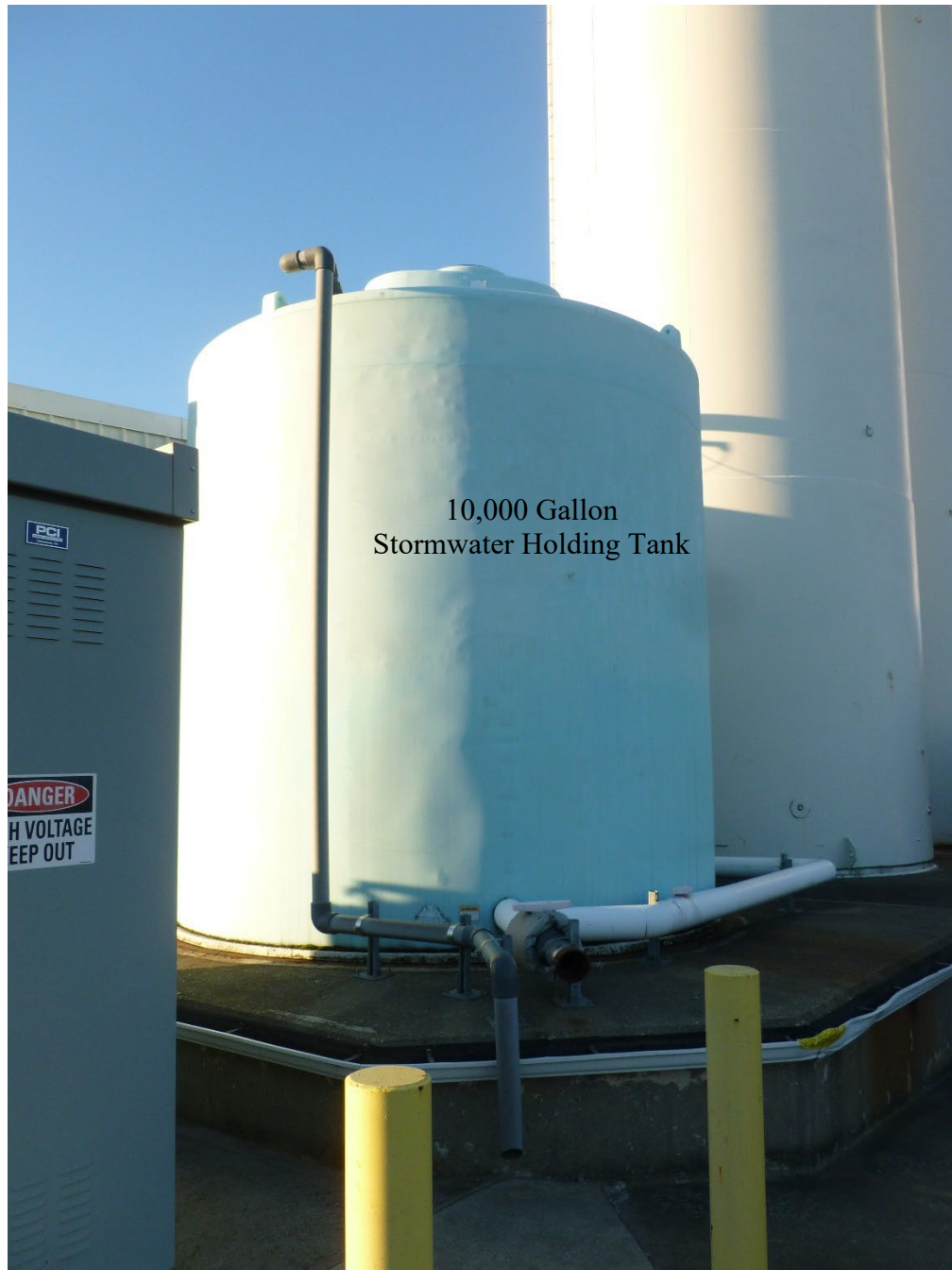
Photo 4 / P1010227 – 10,000 Gallon Stormwater Tank
