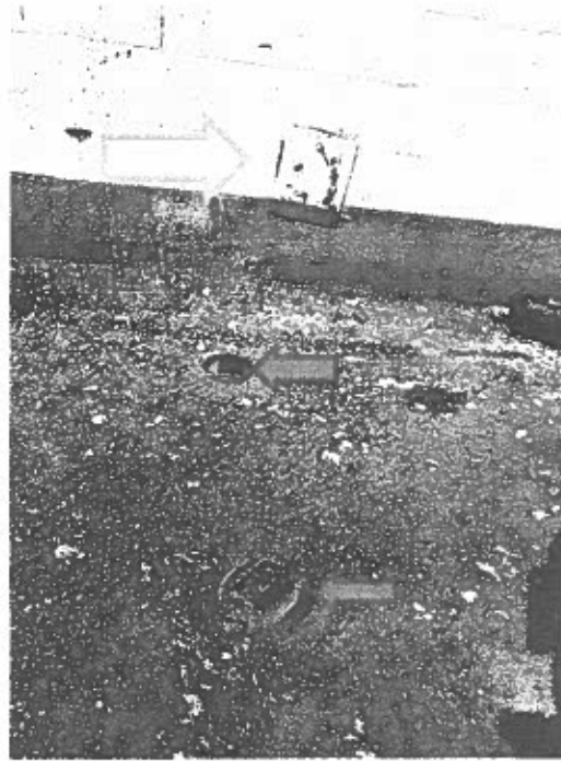
Picture of location: Door (white arrow) is pushed open, and interceptor is in the building – this is used for pumping out and not sampling. Sampler is setup outside, and two cleanouts are on the left side (blue arrows – both are Outfall 002 but bottom one is used for sampling.)
