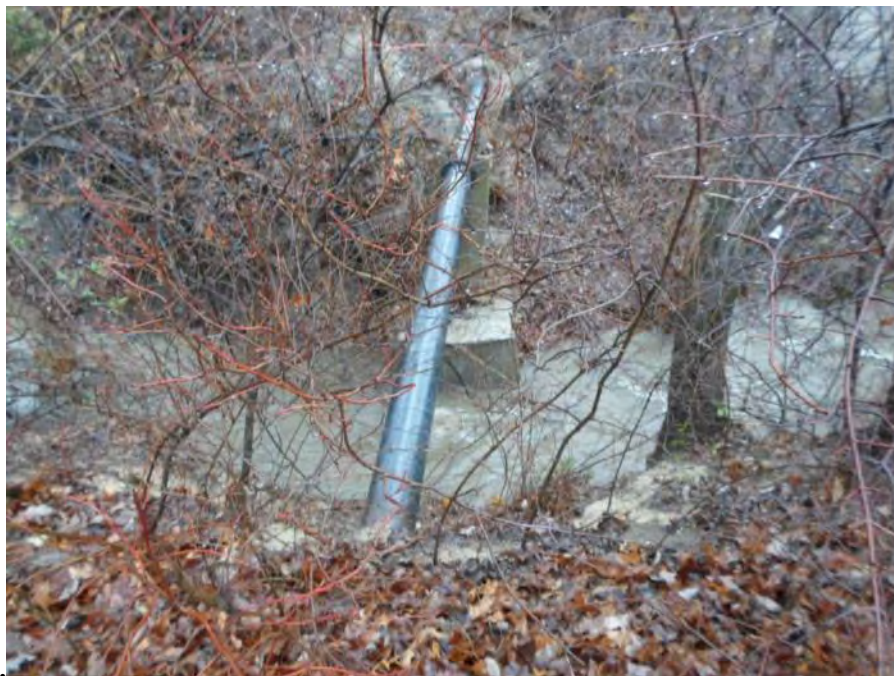
Photograph 17. Aerial Bypass Line from Collins Lift Station – View of the aerial line and its structural support, which is positioned in the stream.
