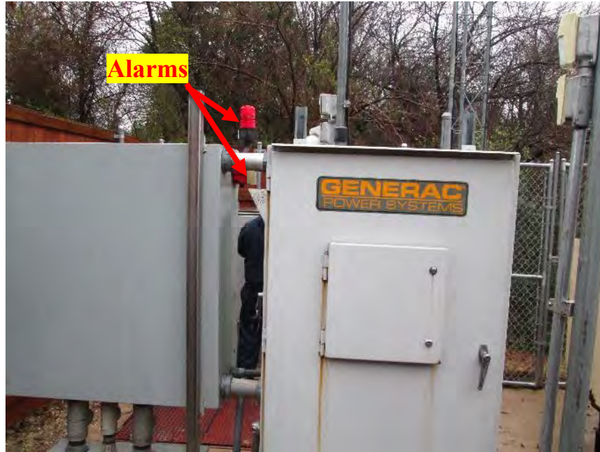
Photograph 45. Lookout Lift Station – View of the station's audio and visual alarms.
