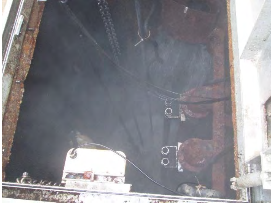
Photograph 47. Lookout Lift Station – View of the station's wet well.
