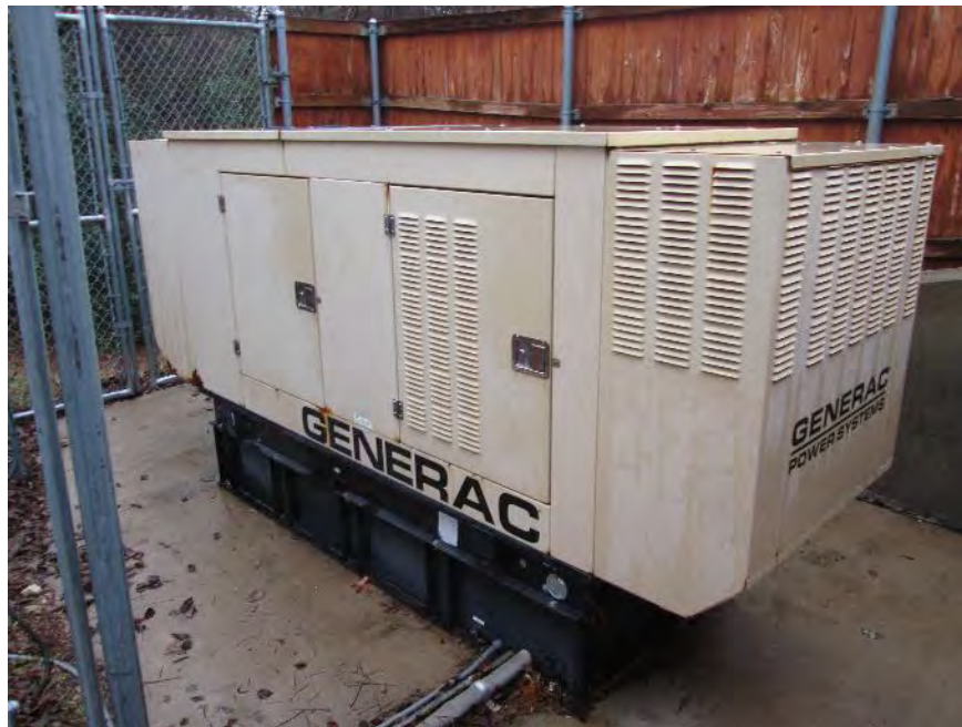
Photograph 44. Lookout Lift Station – View of the station’s onsite backup generator.
