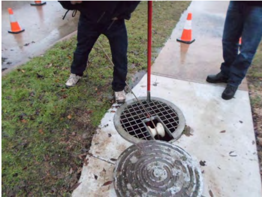
Photograph 31. CCTV Crew – View of a fall protection manhole cover used by operators while televising sewer lines. The manhole was located on a sidewalk in a residential area.
