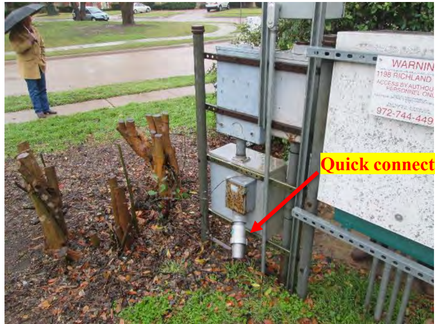
Photograph 7. Richland Park Lift Station – View of the station's quick connect socket.
