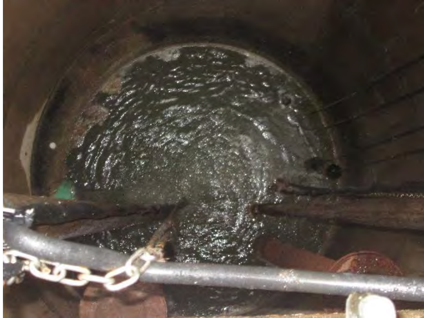
Photograph 39. Clear Creek Lift Station – View of the station's wet well. The influent sewer and station's activation floats were at the wastewater level.
