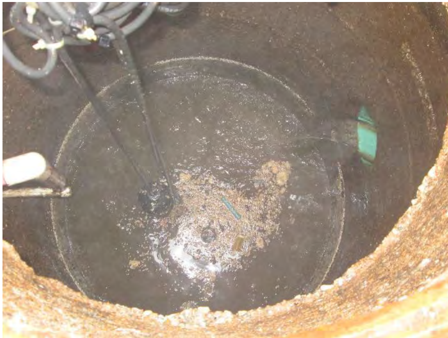
Photograph 14. Meredith Lift Station – View the station's wet well.
