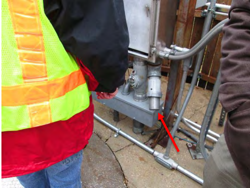
Photograph 41. Clear Creek Lift Station – View of the station's quick connect socket.
