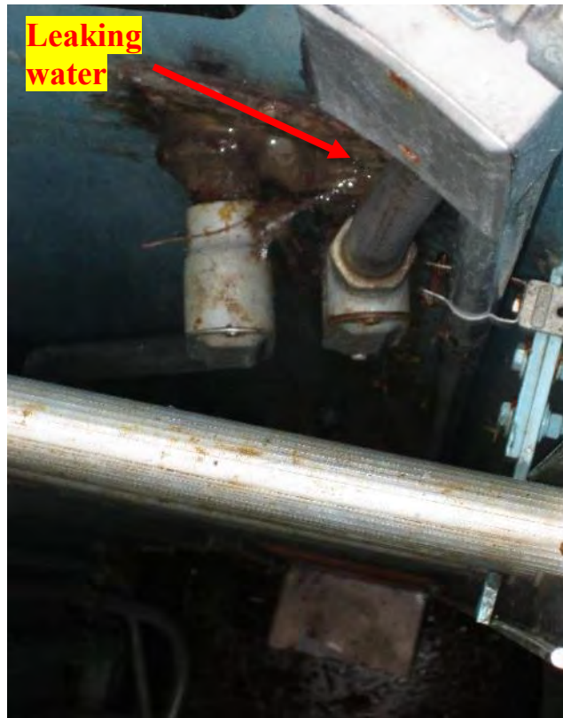
Photograph 24. Collins Lift Station – View of water leaking into the station's dry well. Note that the leak was close to an electrical housing.
