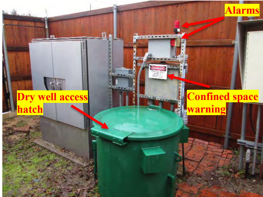
Photograph 11. Meredith Lift Station – View of the station’s dry well access hatch and audio and visual alarms.
