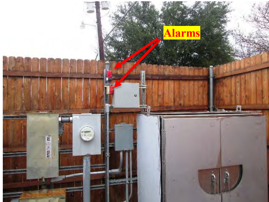
Photograph 21. Collins Lift Station – View of the station's audio and visual alarms.
