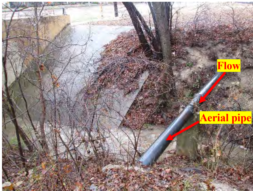
Photograph 16. Aerial Bypass Line from Collins Lift Station – View of the aerial line that delivers wastewater from the Collins Lift Station to the Meredith Lift Station.
