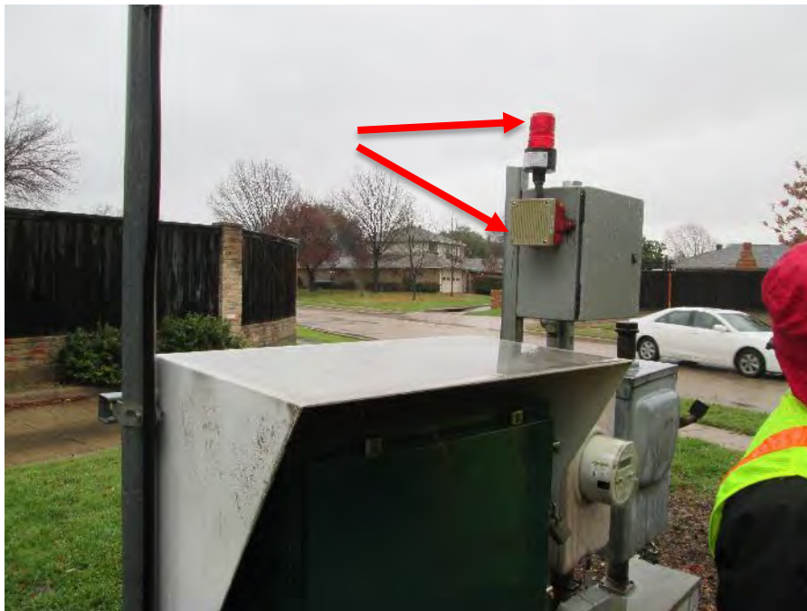
Photograph 4. Richland Park Lift Station – View of the station’s audio and visual alarms (noted by red arrows).
