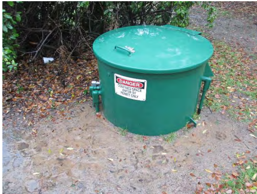
Photograph 6. Richland Park Lift Station – View of the dry well access hatch with confined space warning.
