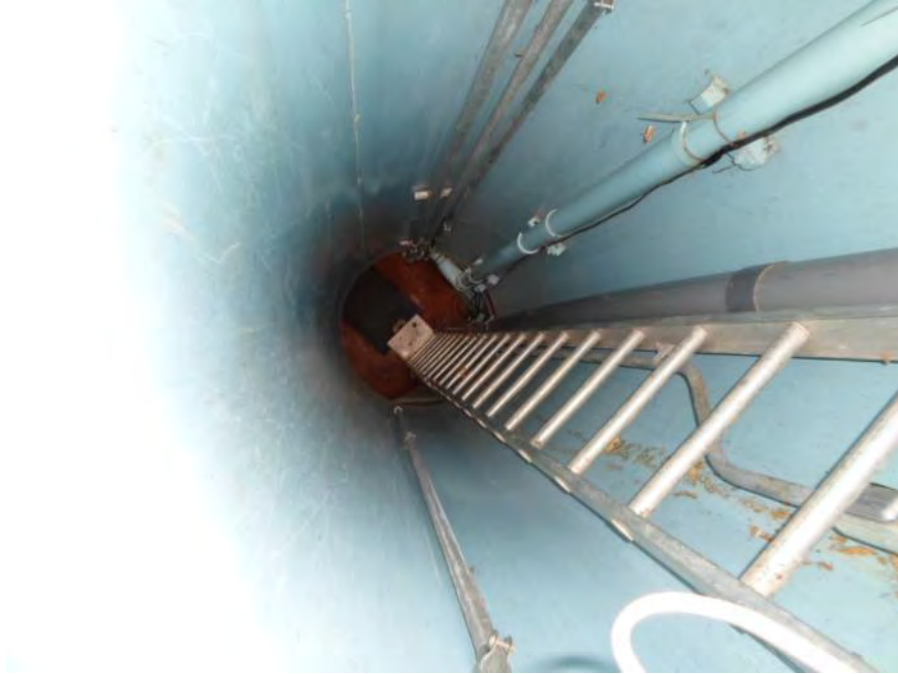
Photograph 5. Richland Park Lift Station – View inside the station’s dry well (approximately 18 feet deep). Note that the chamber was classified as a permit-required confined space.
