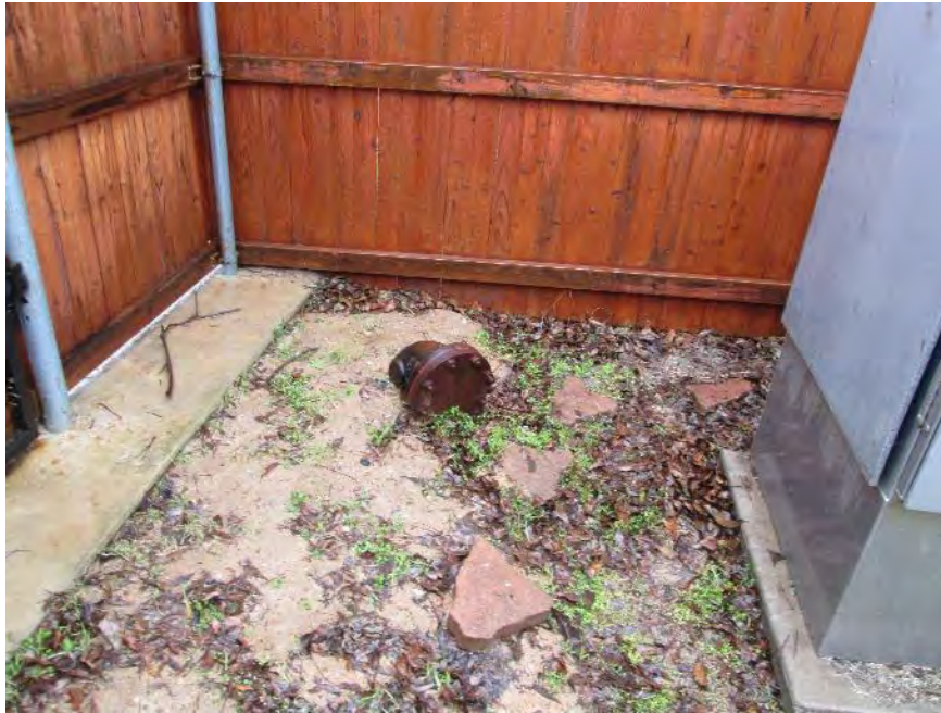
Photograph 19. Meredith Lift Station – View of the station’s bypass flange.
