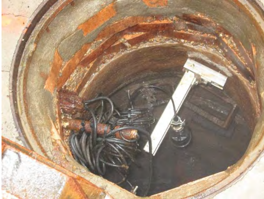
Photograph 27. Collins Lift Station – View inside the station's wet well.
