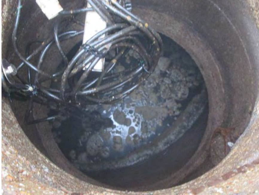
Photograph 9. Richland Park Lift Station – View inside the station’s wet well. Note that chunks of grease were observed floating on the water’s surface.
