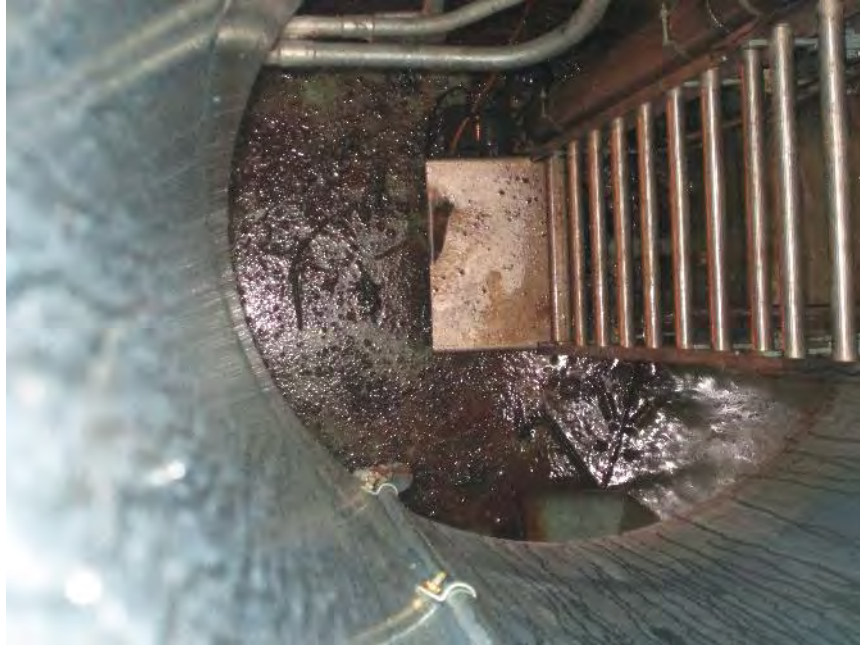
Photograph 23. Collins Lift Station – View inside the dry well. Note that water was observed leaking into the chamber and making the ground damp.
