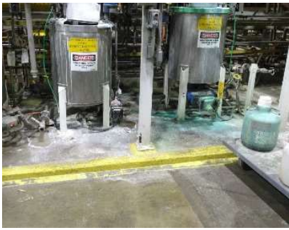
Photo-4 Leaks and Spills of Products near the Process tanks adjacent to the Lab.
