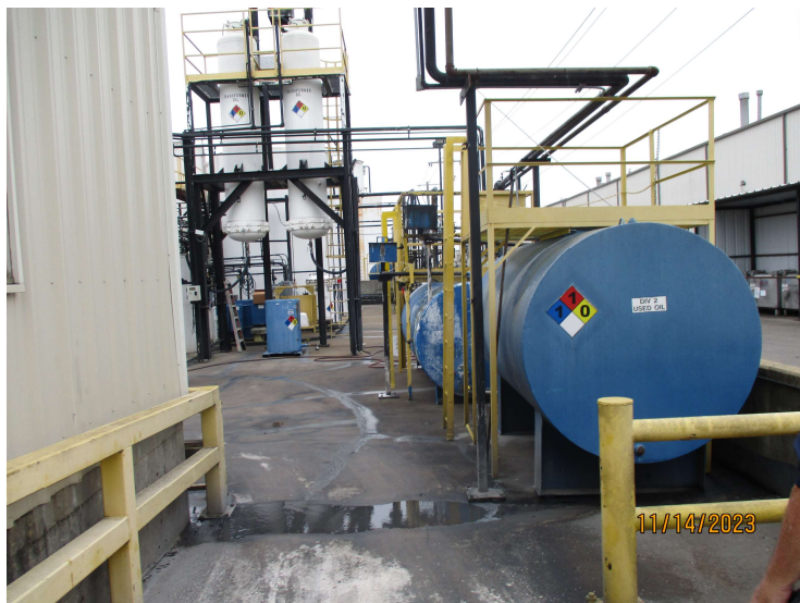
Photo #13 – General view used oil tanks in secondary containment.
