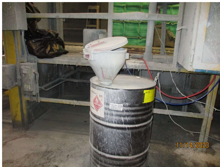
Photo #4 – Division 3 SA3-005, open container
