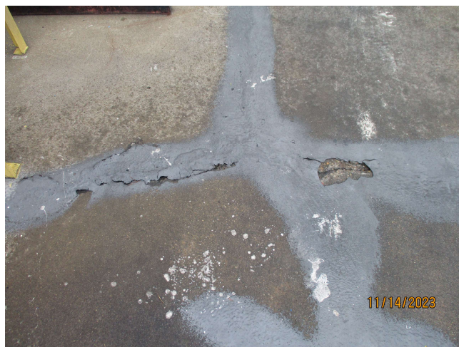
Photo #14 – Cracks on secondary containment
