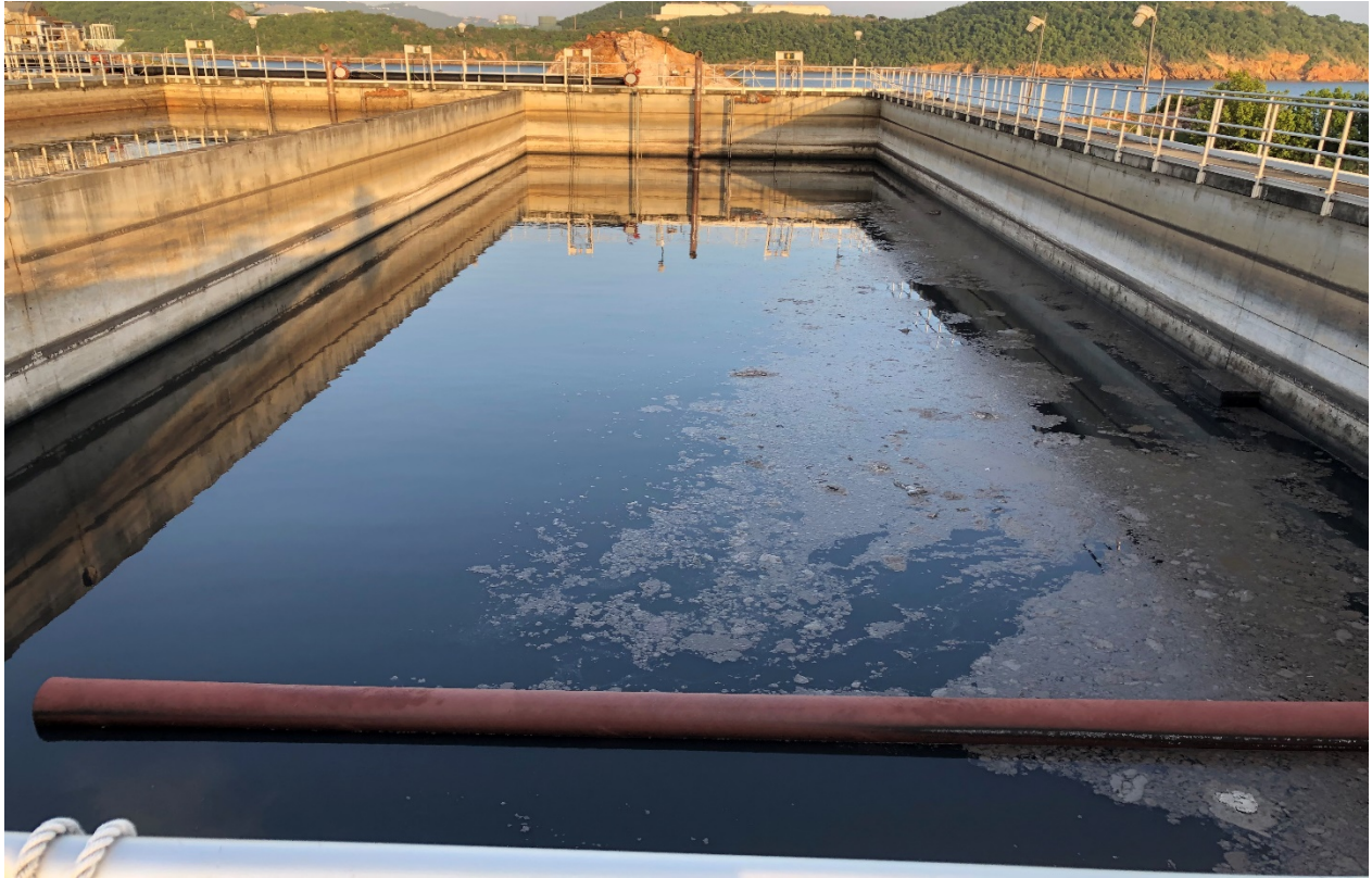
Photo #5: View of SBR 1.
