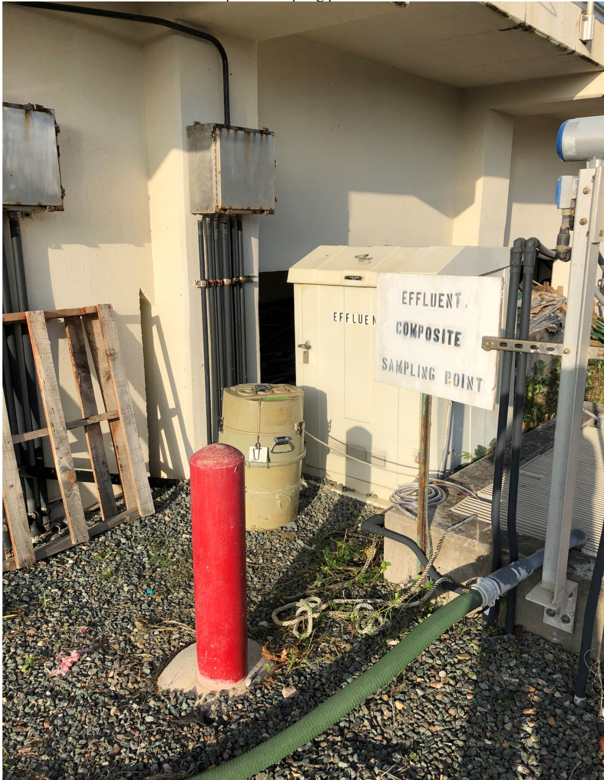
Photo #1: View of the effluent composite sampling point.
