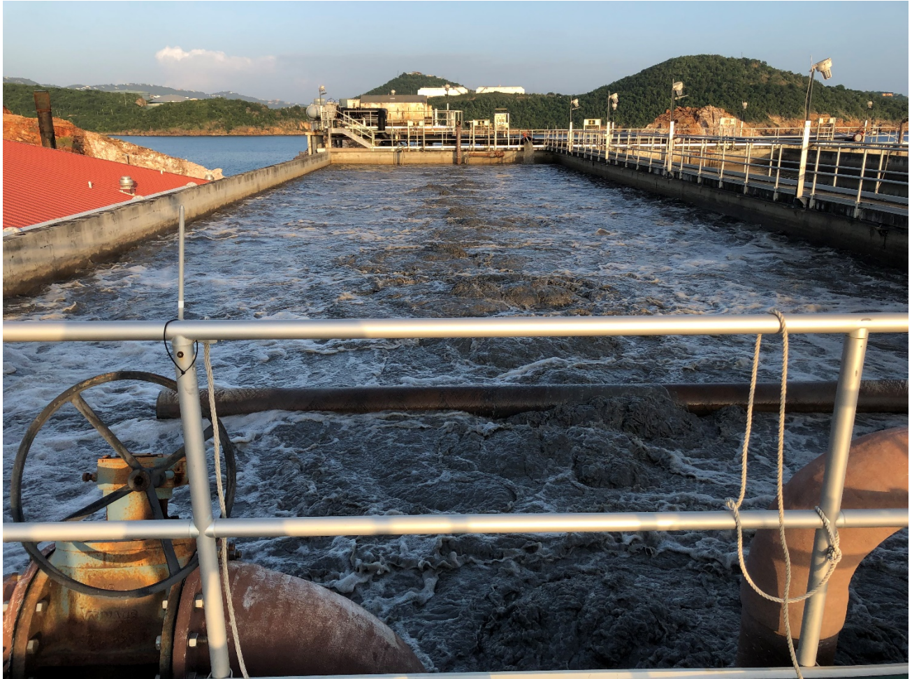
Photo #7: View of SBR 3.
