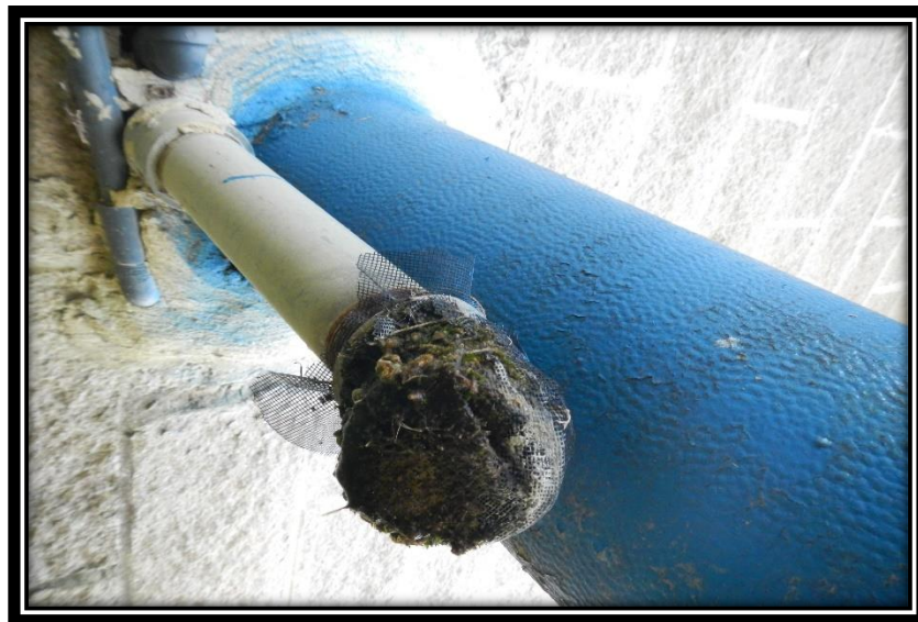
Image 4 Well air vent
