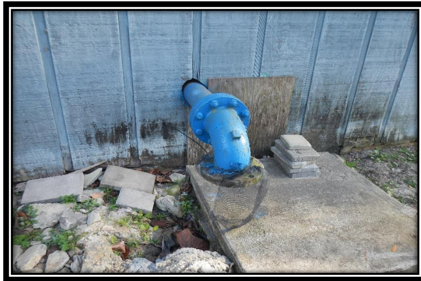
Image 5 Well air vent
