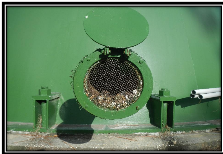
Image 6 Storage tank overflow
