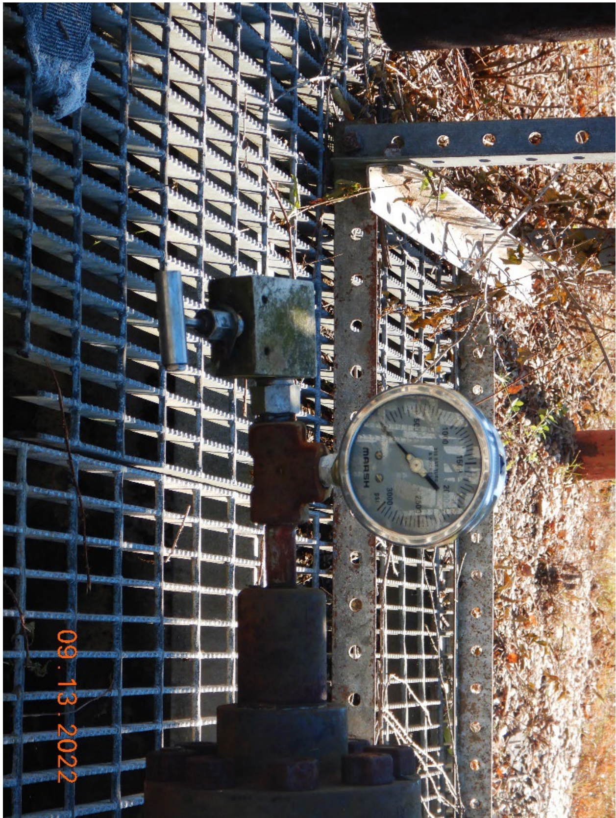
Photograph 4: Looking east, closeup view of production casing pressure gauge reading 0 psi.
