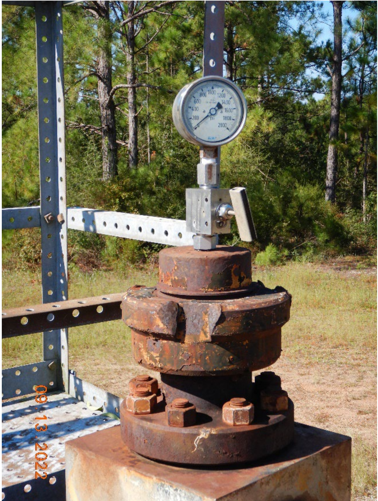
Photograph 6: Looking south, closeup view of internal pressure gauge reading 0 psi.
