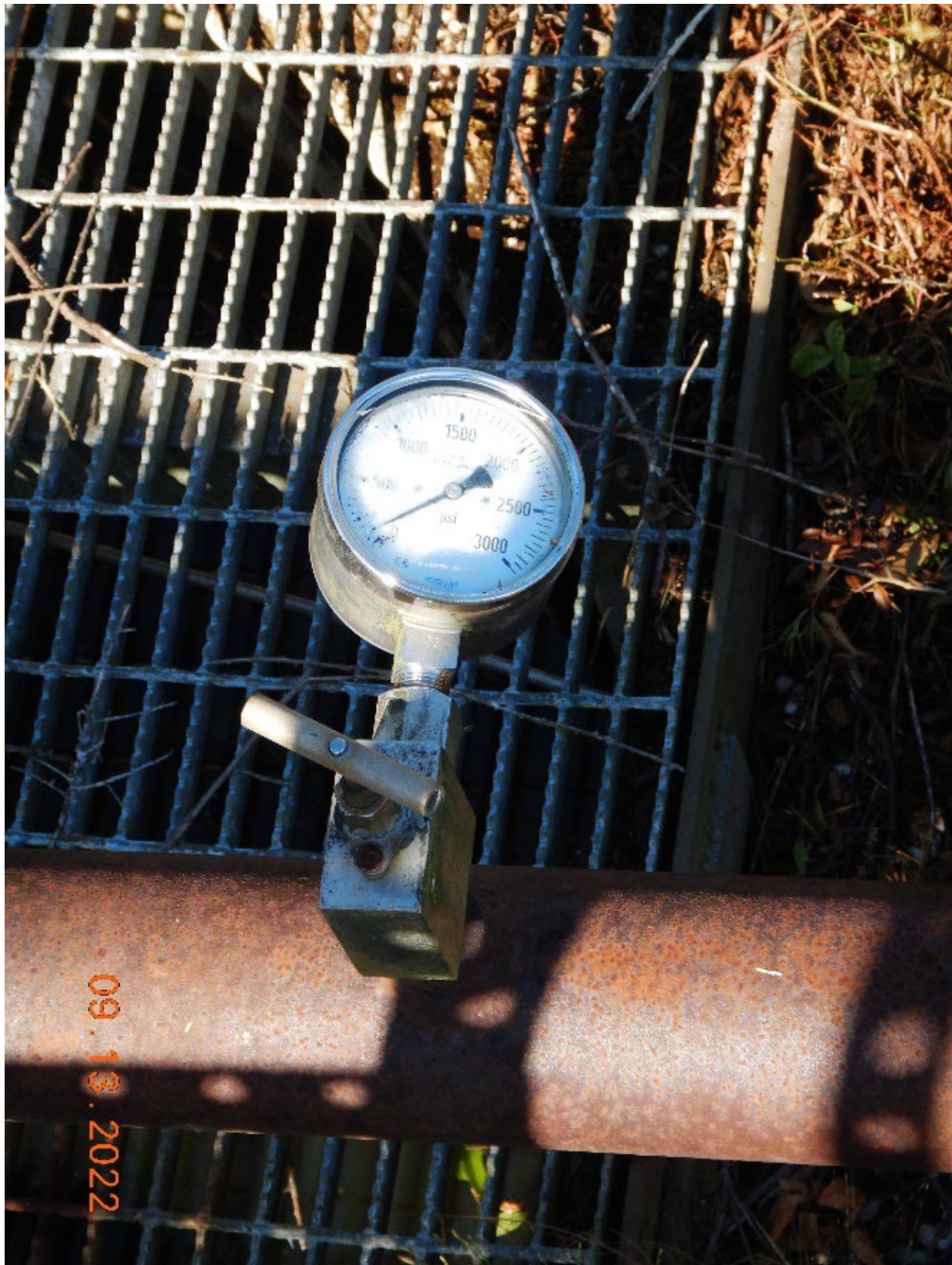
Photograph 5: Looking down, closeup view of line pressure gauge reading 0 psi.
