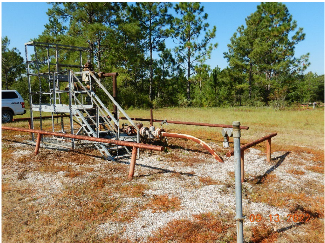
Photograph 2: Looking southwest, site overview showing well head, pressure gauges, valves, and access stairs.
