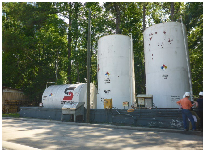
Photo 5: Three storage tanks at the Tank Farm.
