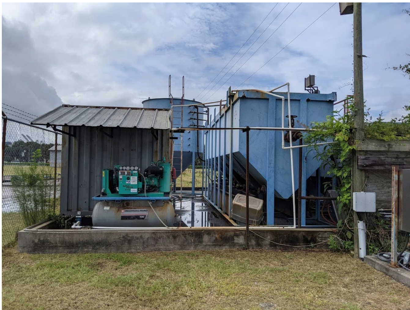
Photograph 3 of 4: Groundwater extraction and treatment system
