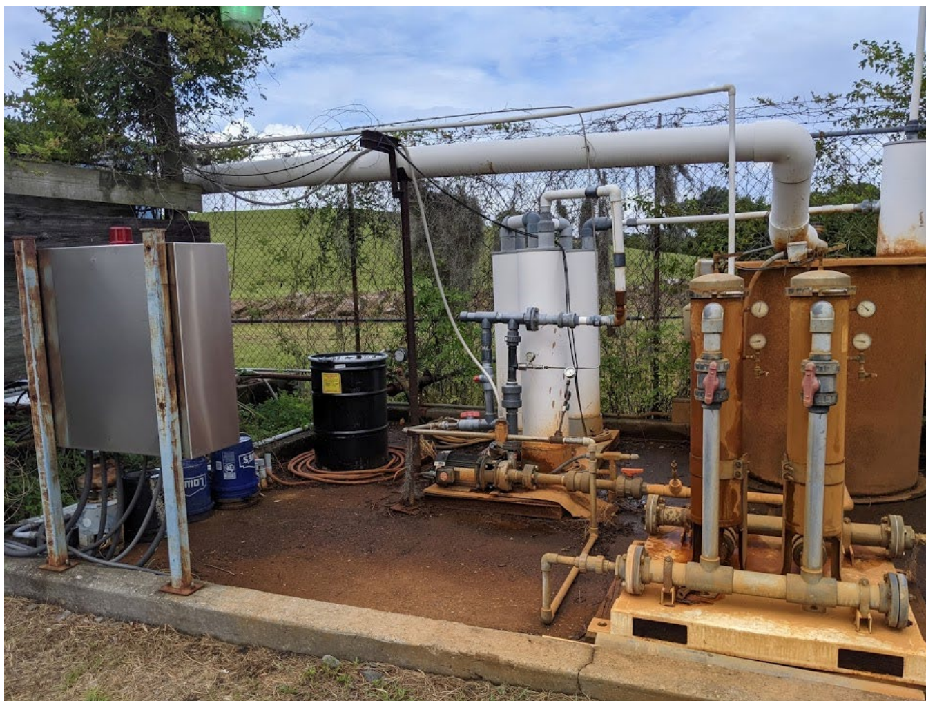
Photograph 4 of 4: Groundwater extraction and treatment system
