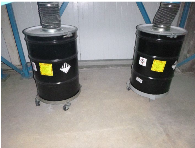
Photograph 22: Building 77 Filter Bank Room.
