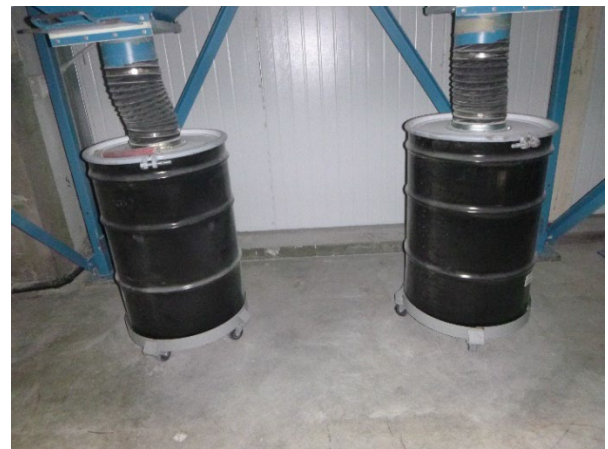
Photograph 20: Building 77 Filter Bank Room
