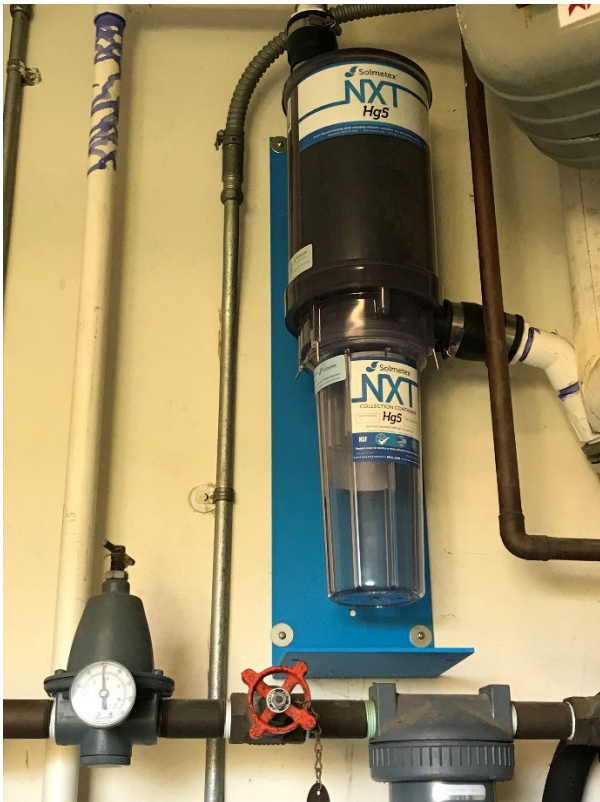
Photograph 17: Amalgam recovery system.
