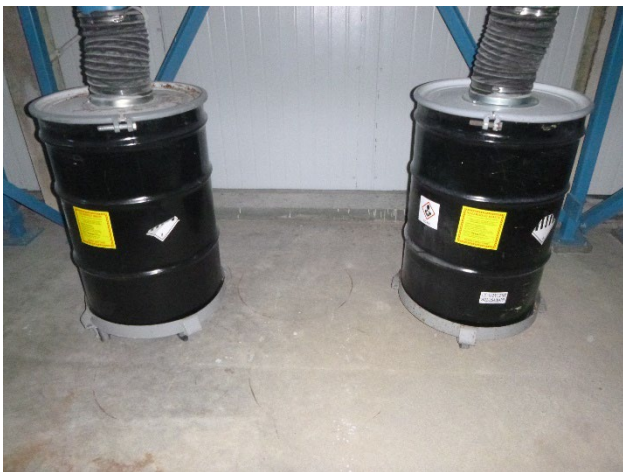
Photograph 23: Building 77 Filter Bank Room..
