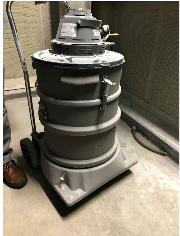
Photograph 24: Building 77 Filter Bank Room..
