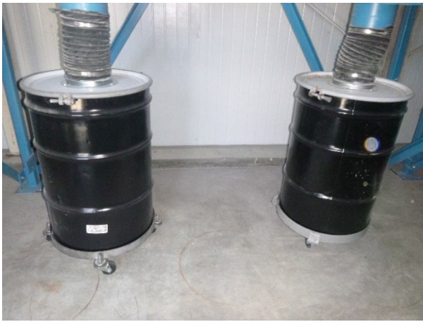
Photograph 21: Building 77 Filter Bank Room.
