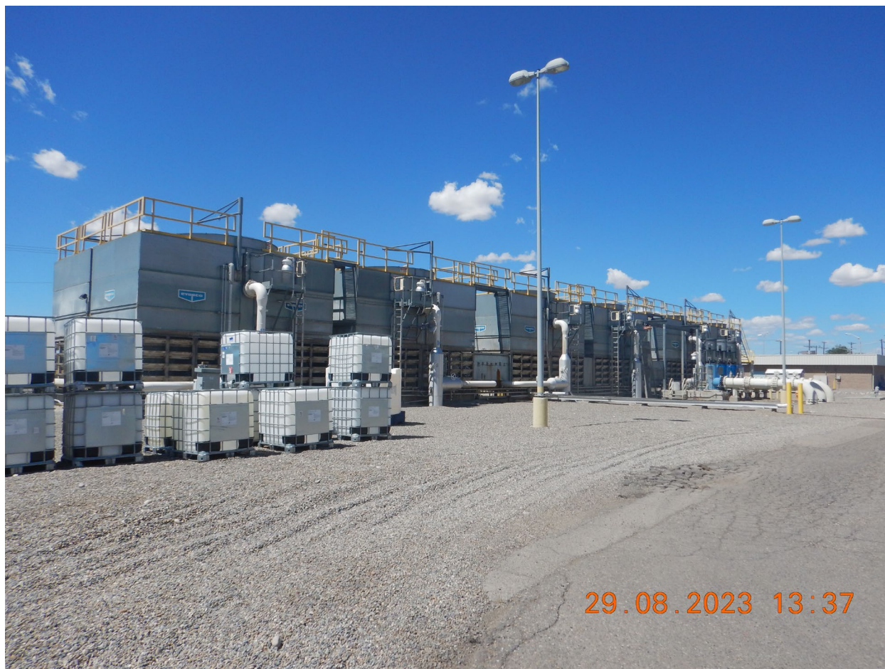
View of FEUS-Bluffview Power Plant Cooling Towers looking approximately Northwest. (DSCN2632). Photographed by D. Esparza
