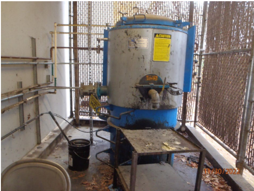
Figure 6: PB300013.JPG – Solvent Recycling Still Unit
