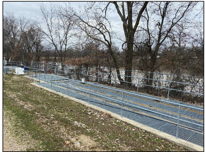
Photo 6: New chlorine contact chamber.
