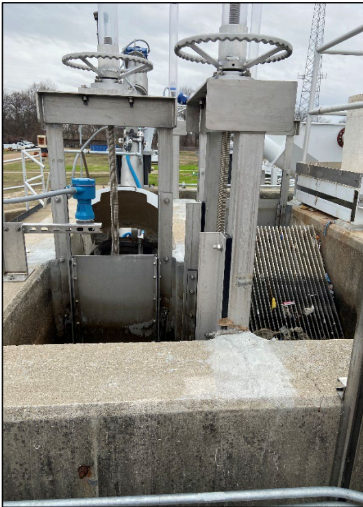
Photo 1: Auger (Left) and bar screen (Right).
