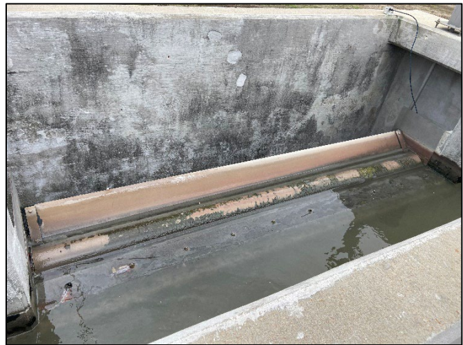
Photo 2: Bypass weir to lagoons at headworks.
