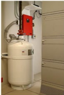
Figure 3-3: Example gas canister in FK-5-1-12 clean fire suppressant system
