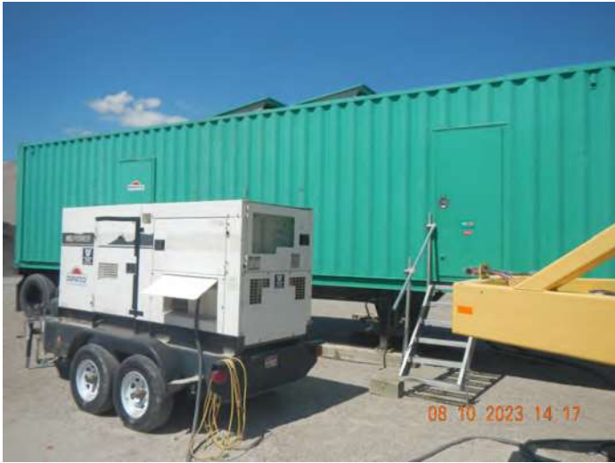
Photo #:09 (DSCN3393) Description: Photo of the two generators located at the hot mix asphalt plant.
