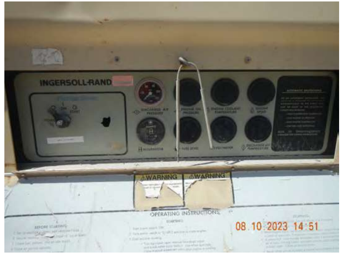
Photo #:22 (DSCN3408) Description: Photo of an auxiliary generator near the crushing operation. Ingersoll-Rand. Hour meter read at 02144.3.
