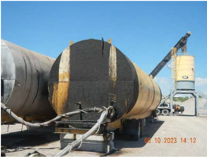
Photo #:05 (DSCN3389) Description: Photo of the 30,000-gallon and 35,000-gallon asphalt oil tanks at the hot mix asphalt plant.
