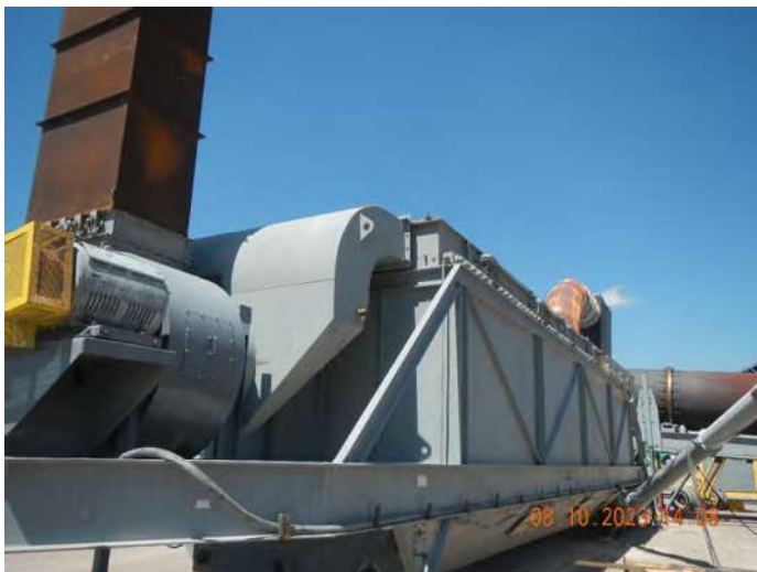
Photo #:03 (DSCN3387) Description: Photo of the ADM Baghouse associated with the drum/dyer at the hot mix asphalt plant.
