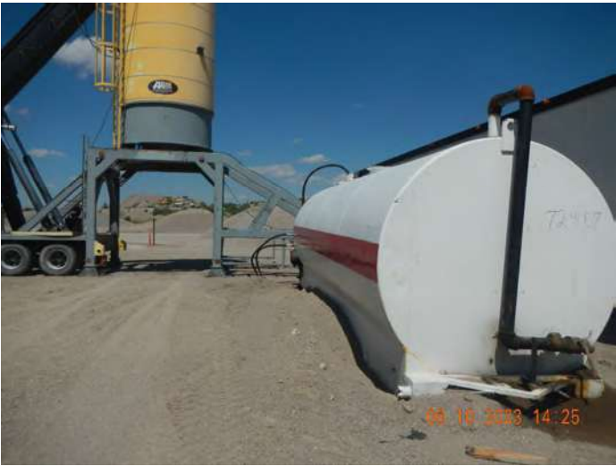
Photo #:12 (DSCN3397) Description: Photo of the diesel storage tank at the hot mix asphalt plant.
