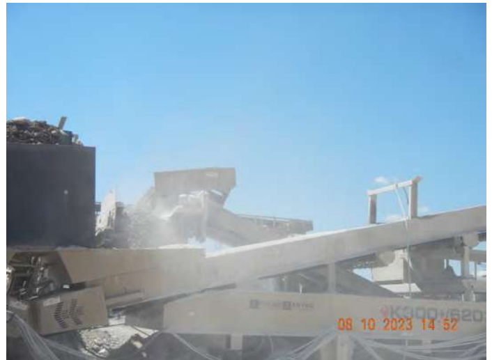
Photo #:24 (DSCN3410) Description: Photo of visible emissions/dust at one of the conveyors.
