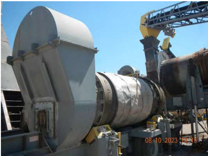
Photo #:07 (DSCN3391) Description: Photo of the mixing drum at the hot mix asphalt plant.
