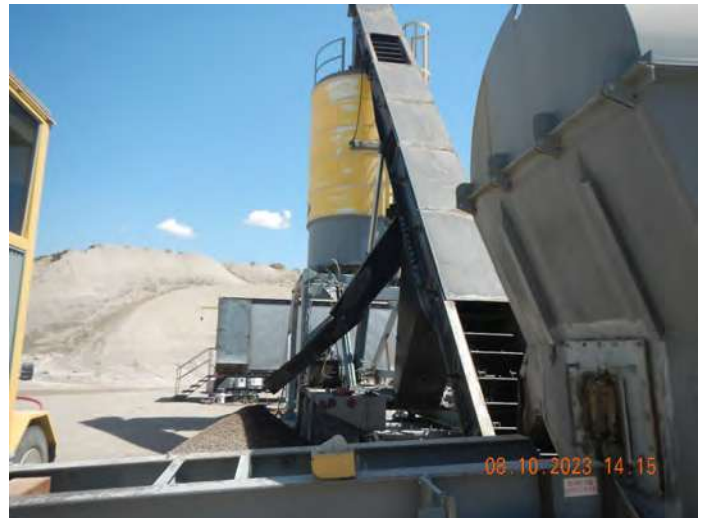
Photo #:08 (DSCN3392) Description: Photo of drag slat conveyor and silo at the hot mix asphalt plant.
