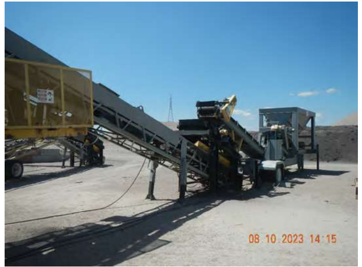
Photo #:06 (DSCN3390) Description: Photo of a conveyor and recycled asphalt bin at the hot mix asphalt plant.
