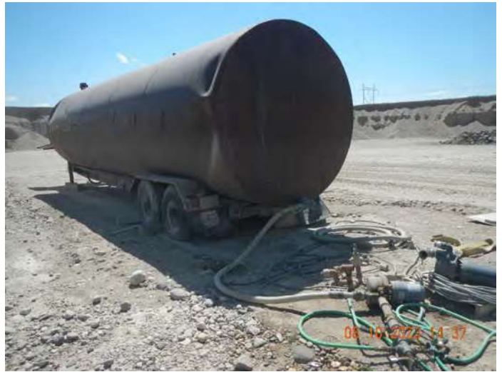
Photo #:18 (DSCN3402) Description: Photo of the water tank used at the crushing operation. Used for wet suppression.
