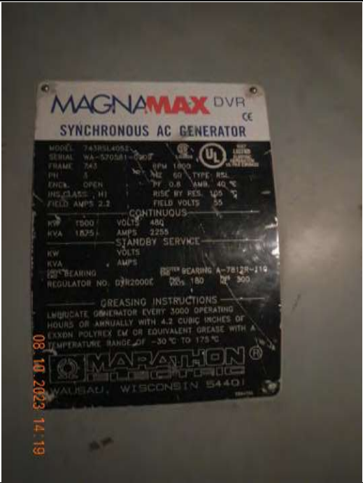
Photo #:11 (DSCN3395) Description: Photo of the nameplate off the larger generator at the hot mix asphalt plant. MagnaMax Model# 743RSL4052.
