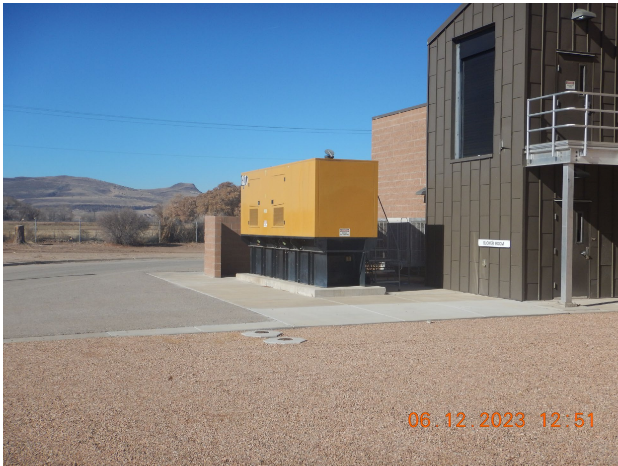
View of the back-up generator outside the Blower Room at the MBR. (DSCN2655). Photographed by D. Esparza
