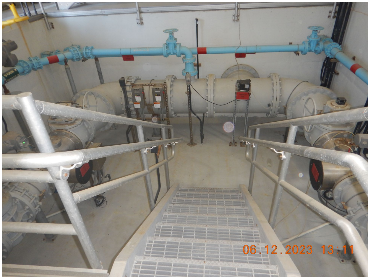
View of the MBR ultraviolet disinfection modules. The eastside module is on the left and the westside is on the right of the photograph. (DSCN2665). Photographed by D. Esparza
