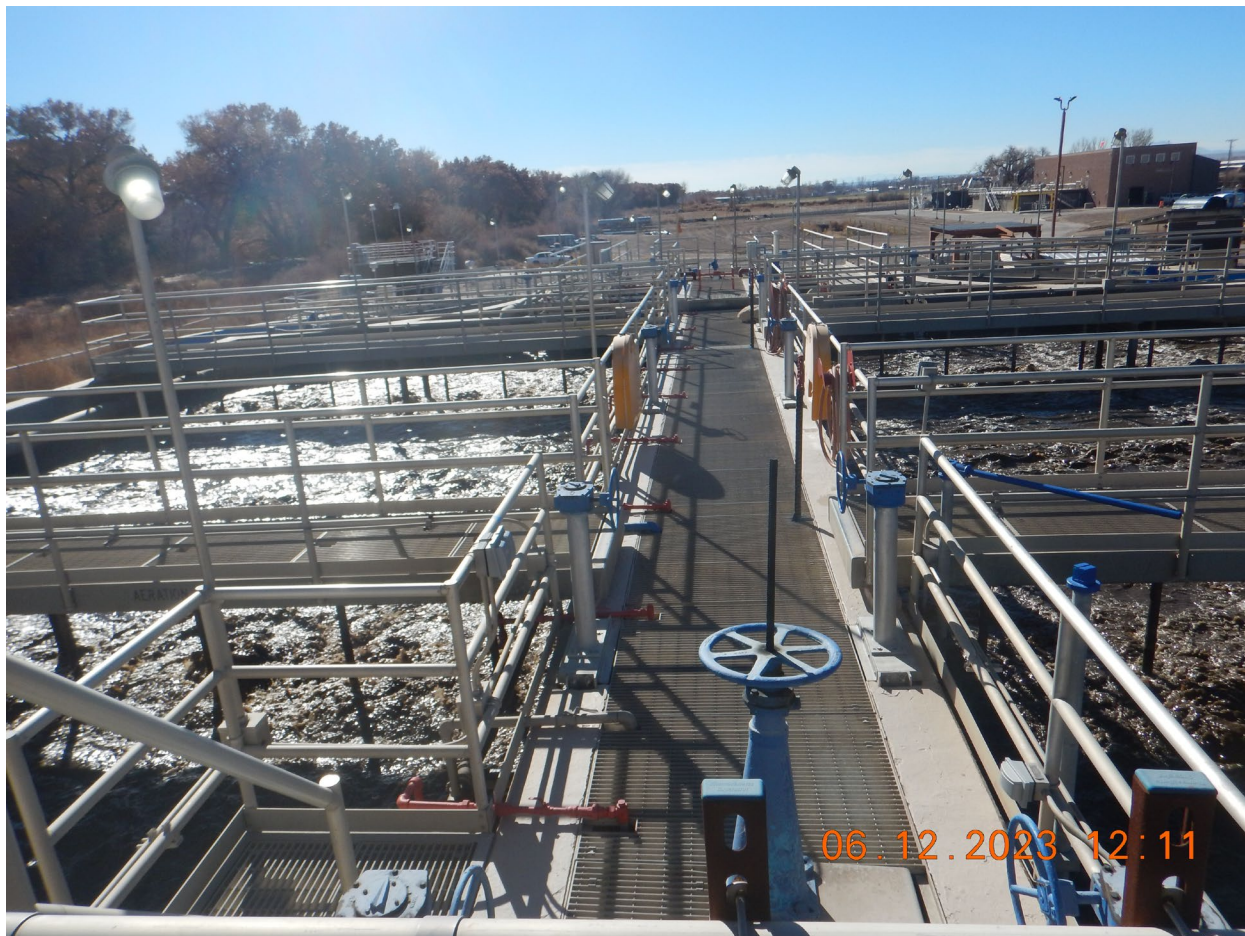
View of the CAS aeration basins looking approximately South. (DSCN2650). Photographed by D. Esparza
