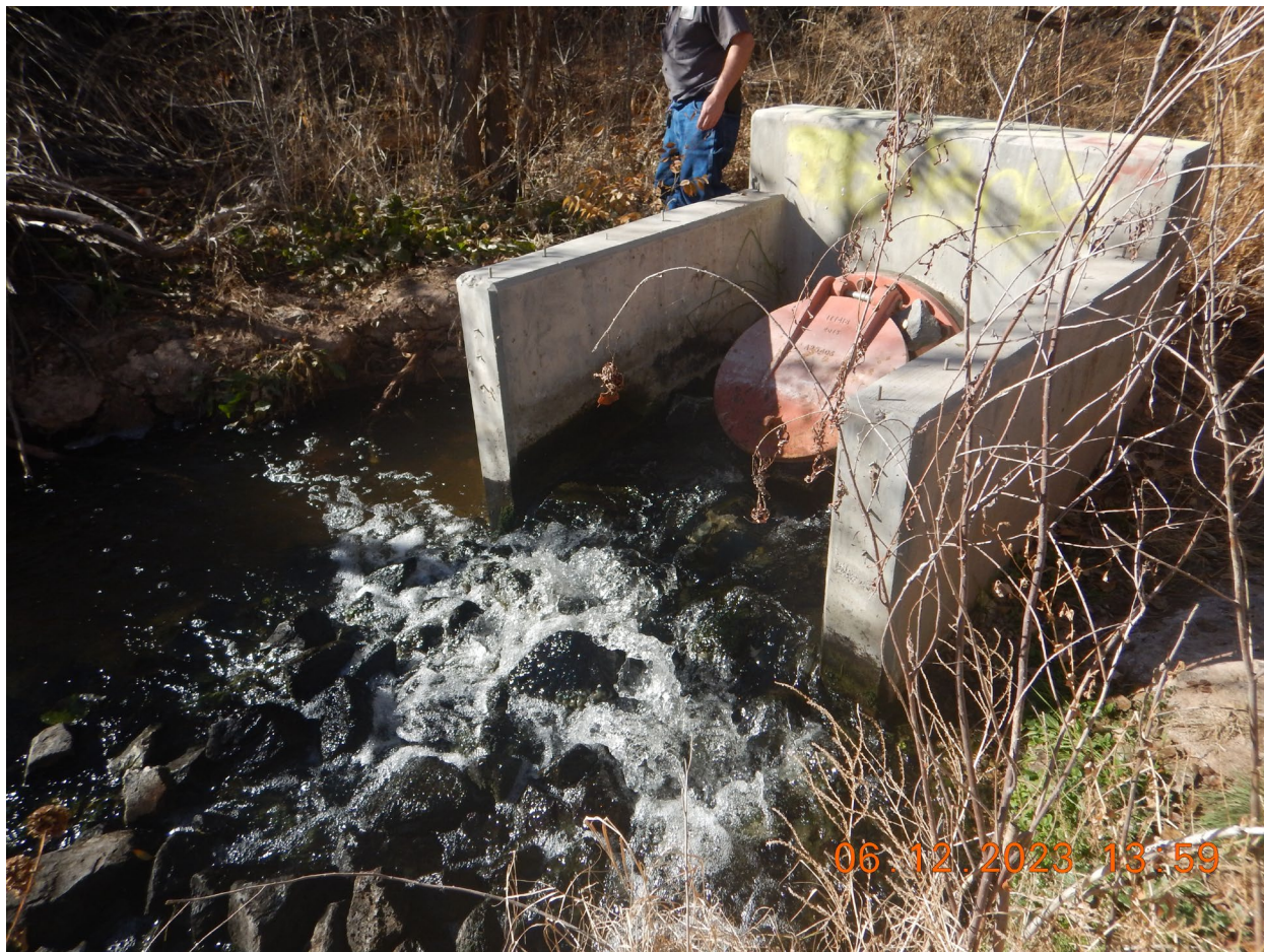
View of the WWTP effluent discharge into the Rio Grand Bosque. (DSCN2673). Photographed by D. Esparza
