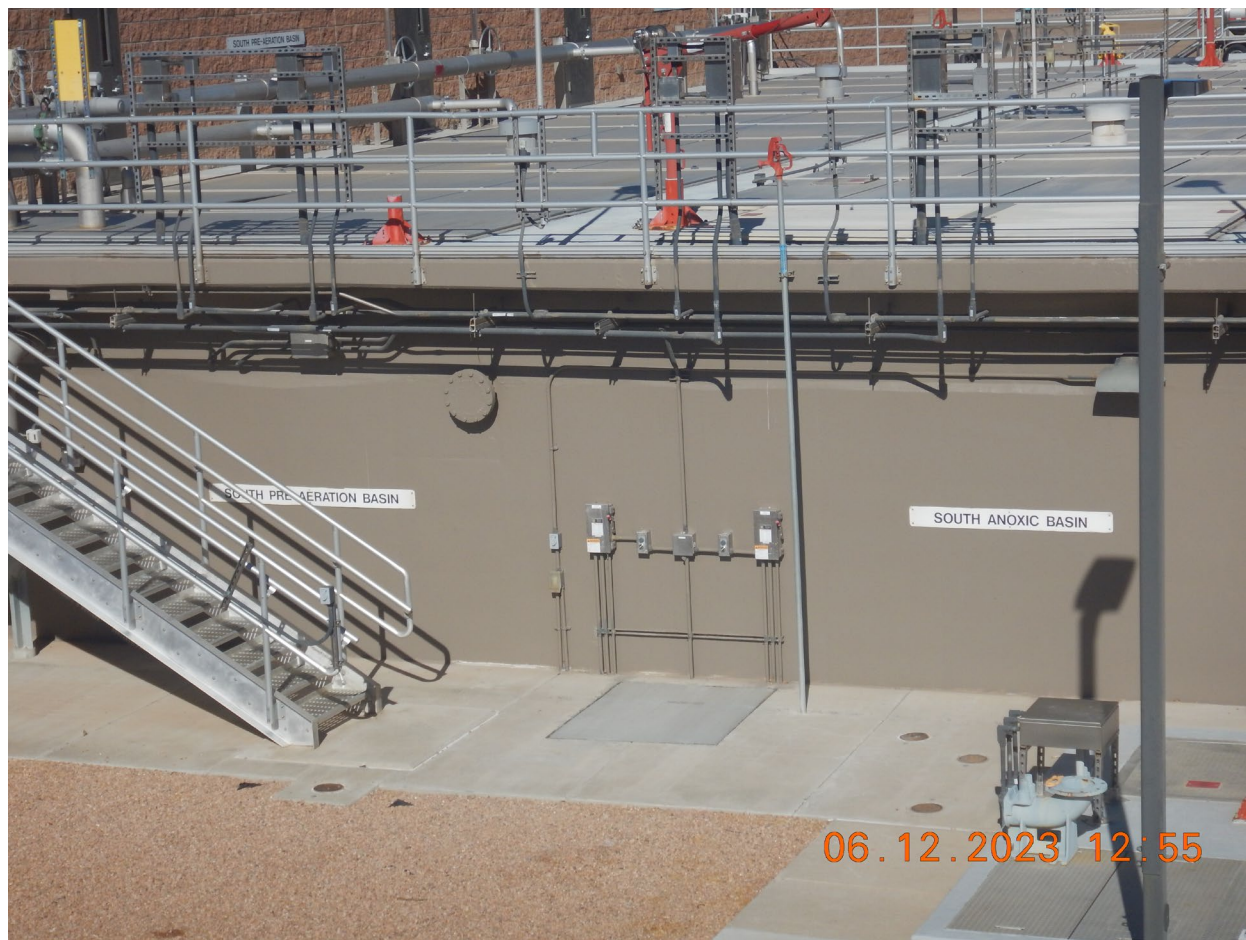
View of the MBR pre-aeration basin and south anoxic basin. (DSCN2658). Photographed by D. Esparza
