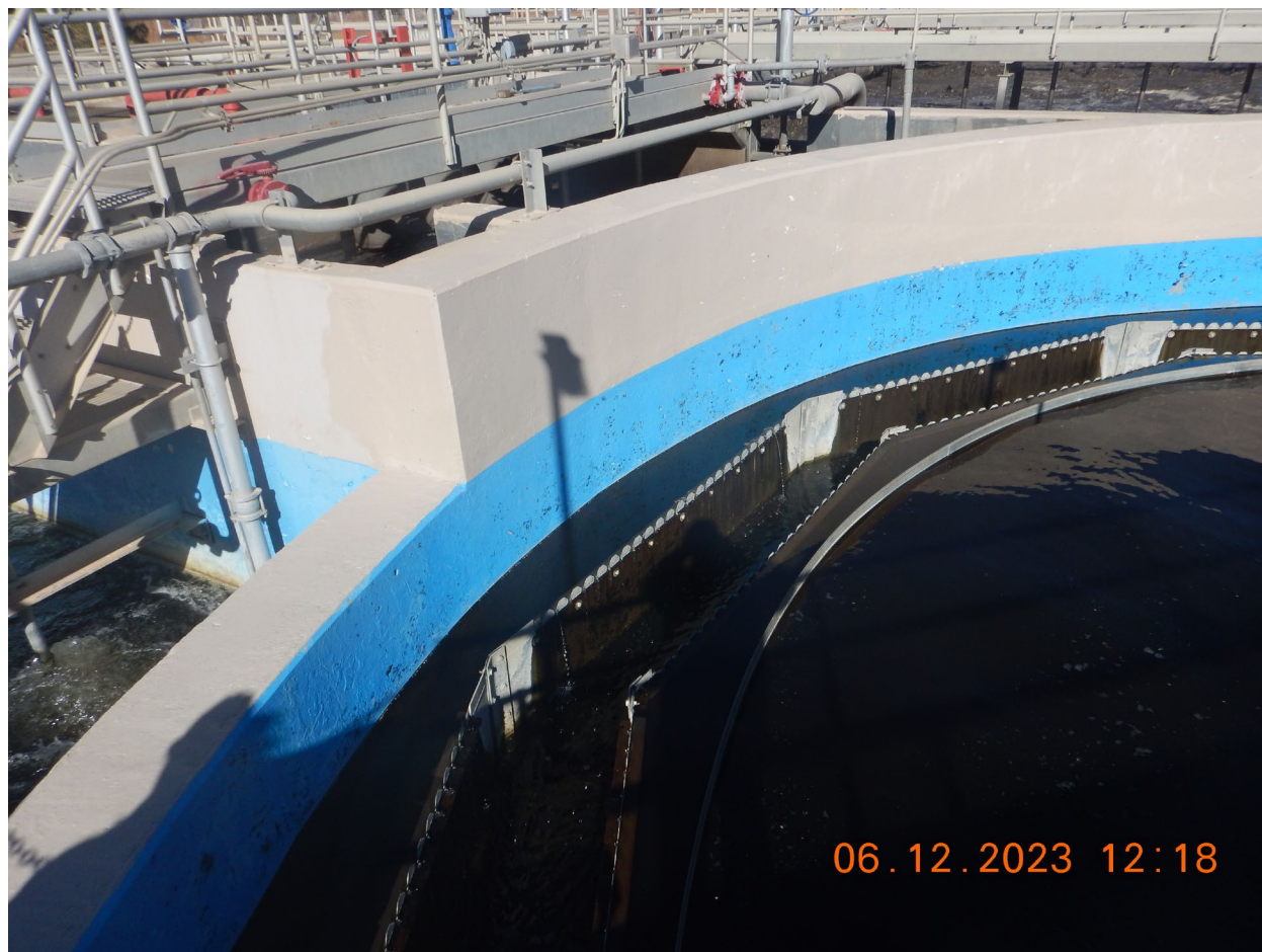
View of the one (1) of the CAS clarifiers. Note: the weir blades. (DSCN2652). Photographed by D. Esparza
