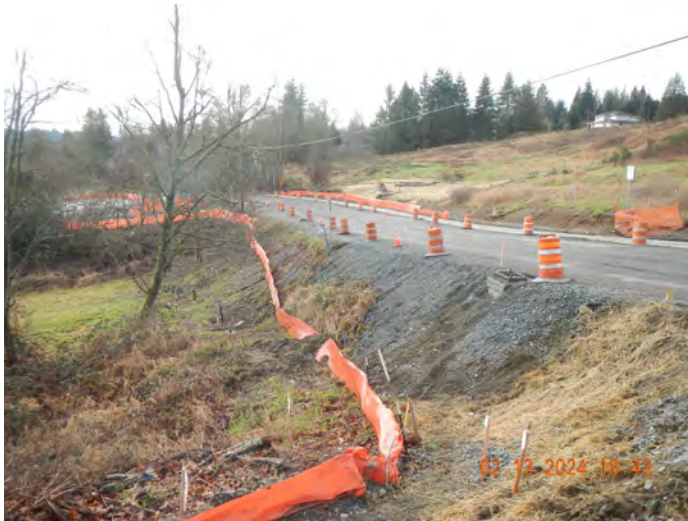
Photo #:11 (DSCN3583) Description: Facing south, photo from “Lot 50” of silt fencing in need of maintenance. Area is east of Williams Road. City of Lake Stevens recently in the area doing some water main work.
