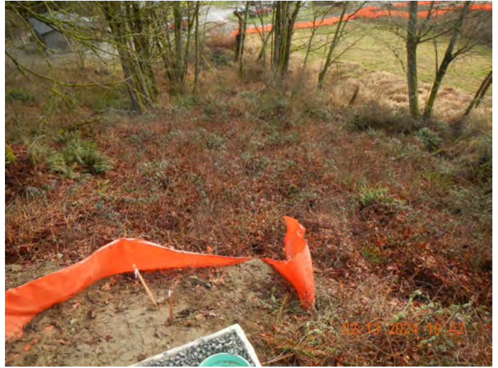
Photo #:10 (DSCN3582) Description: Facing east, photo of silt fencing in need of maintenance (southeast corner of “lot 50”).
