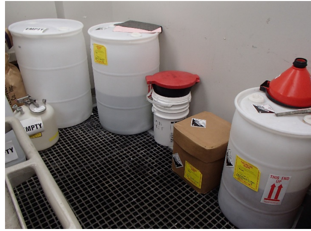
Photo 5: Room 24105A – Chem Waste Storage.
