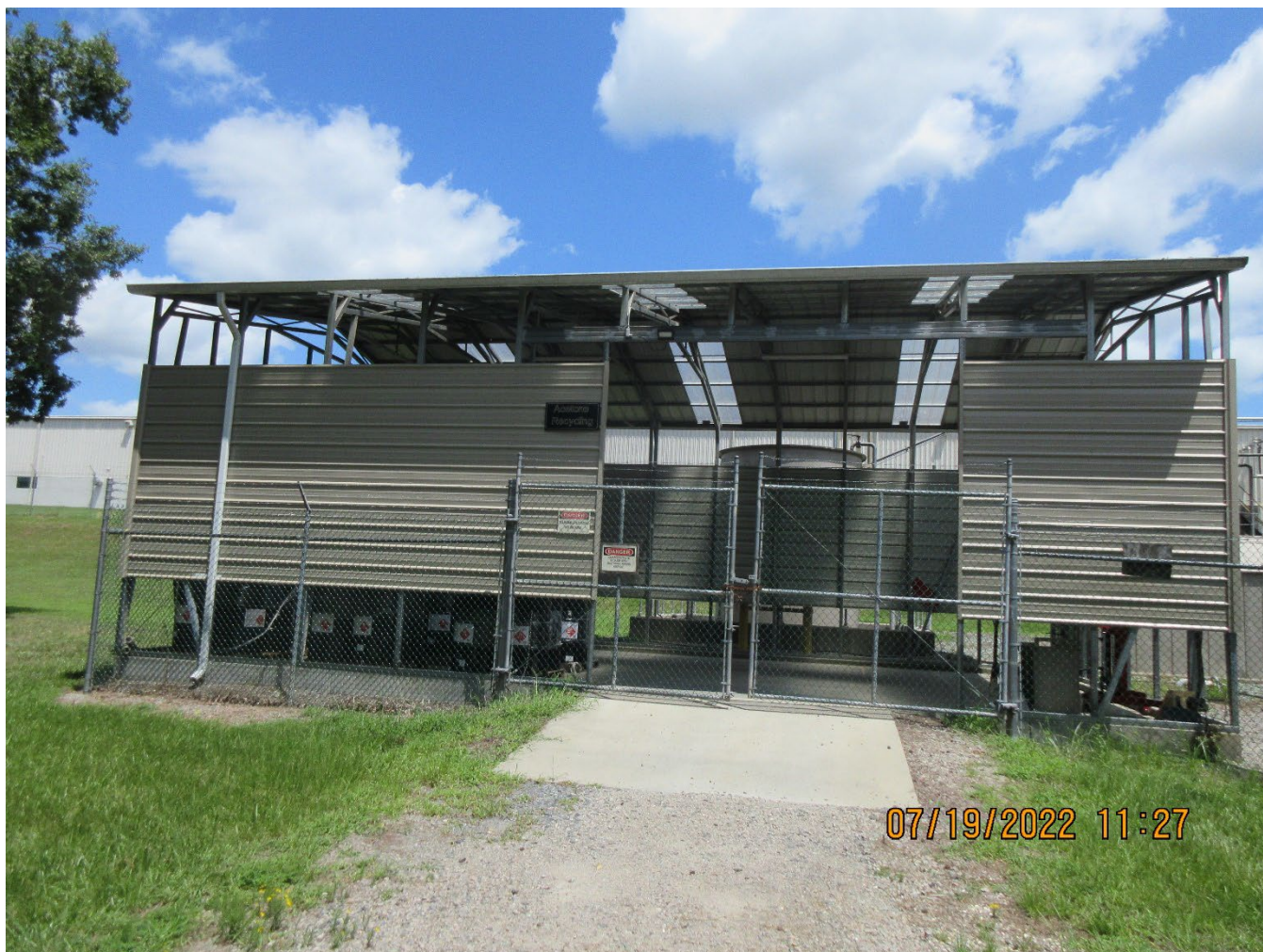
Photo 10 – Acetone Recycling Area near WWTP
