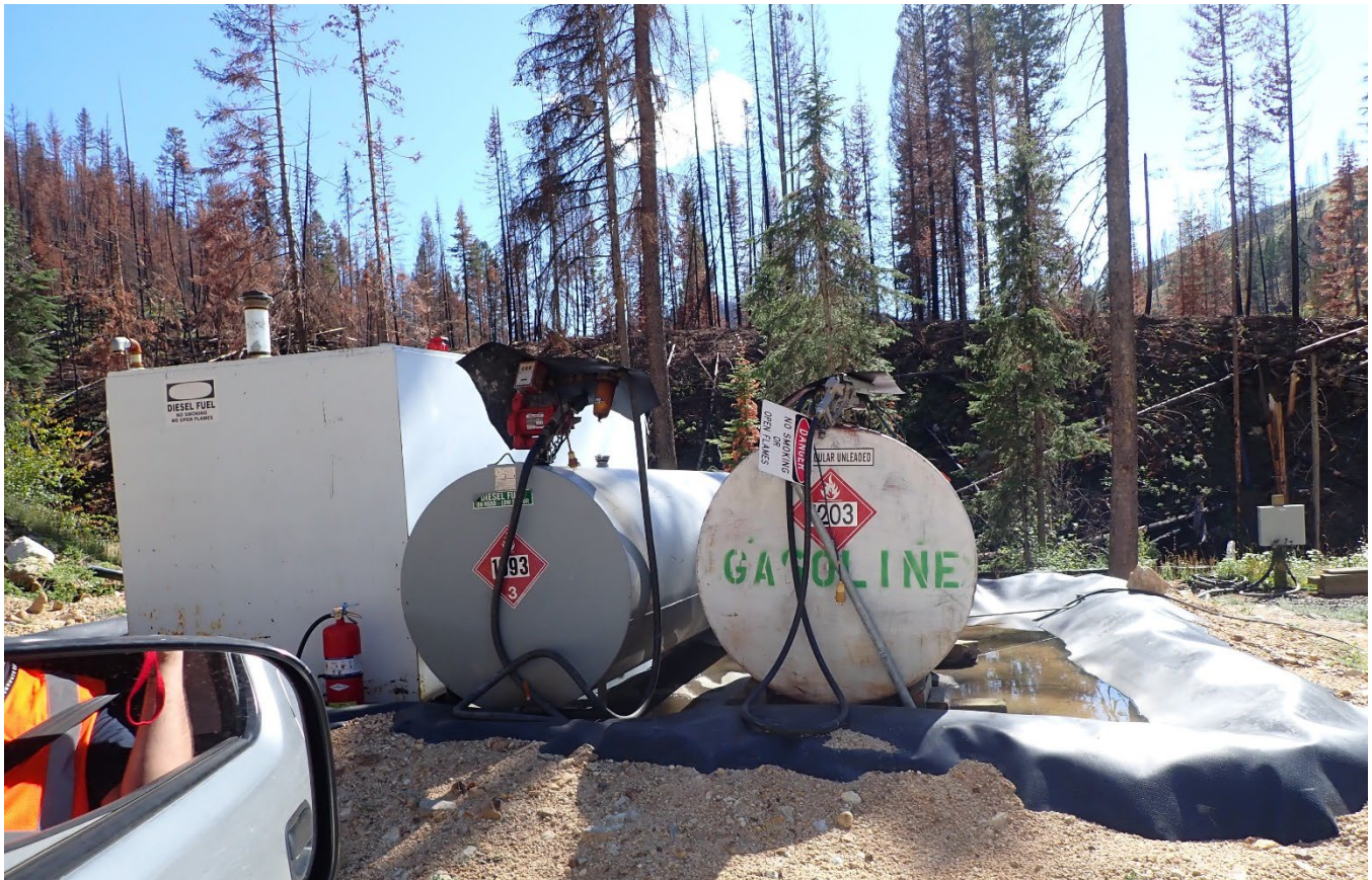
Photo 1 - Fuel storage and secondary containment
