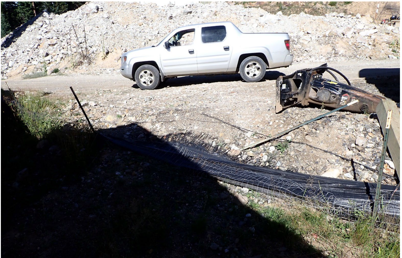
Photo 5 - Damaged and down sediment fence
