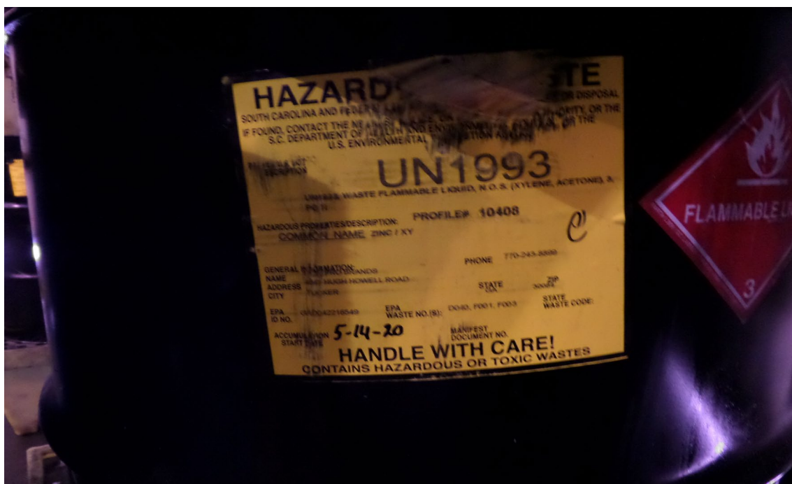
ITW Pro Brands. 90-Day or Less Accumulation Area. Inspectors observed one 55-gallon container accumulating waste acetone and xylene labeled with words hazardous waste and marked with the date 5/14/20. Photograph 7 taken at 11:16 a.m.
