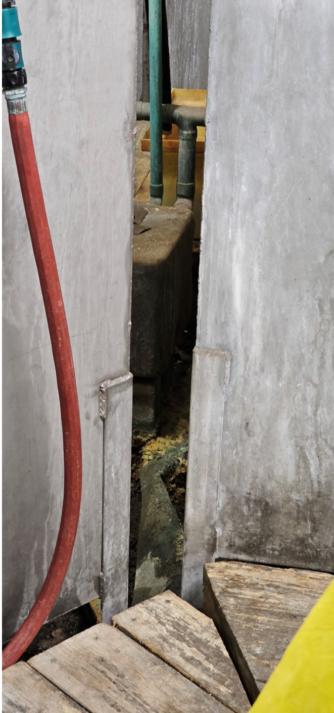
Figure 3: This figure shows hazardous waste acid observed on the floor of this area at the time of the inspection, and obvious signs of corrosion of the surrounding concrete and structural supports were observed.
