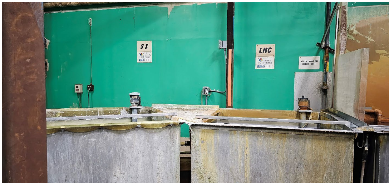
Figure 2: This figure shows the two nitric acid tanks located in the chem-line area. Apparent spill staining observed on the cross platform between the tanks as well as the sides of the tanks.
