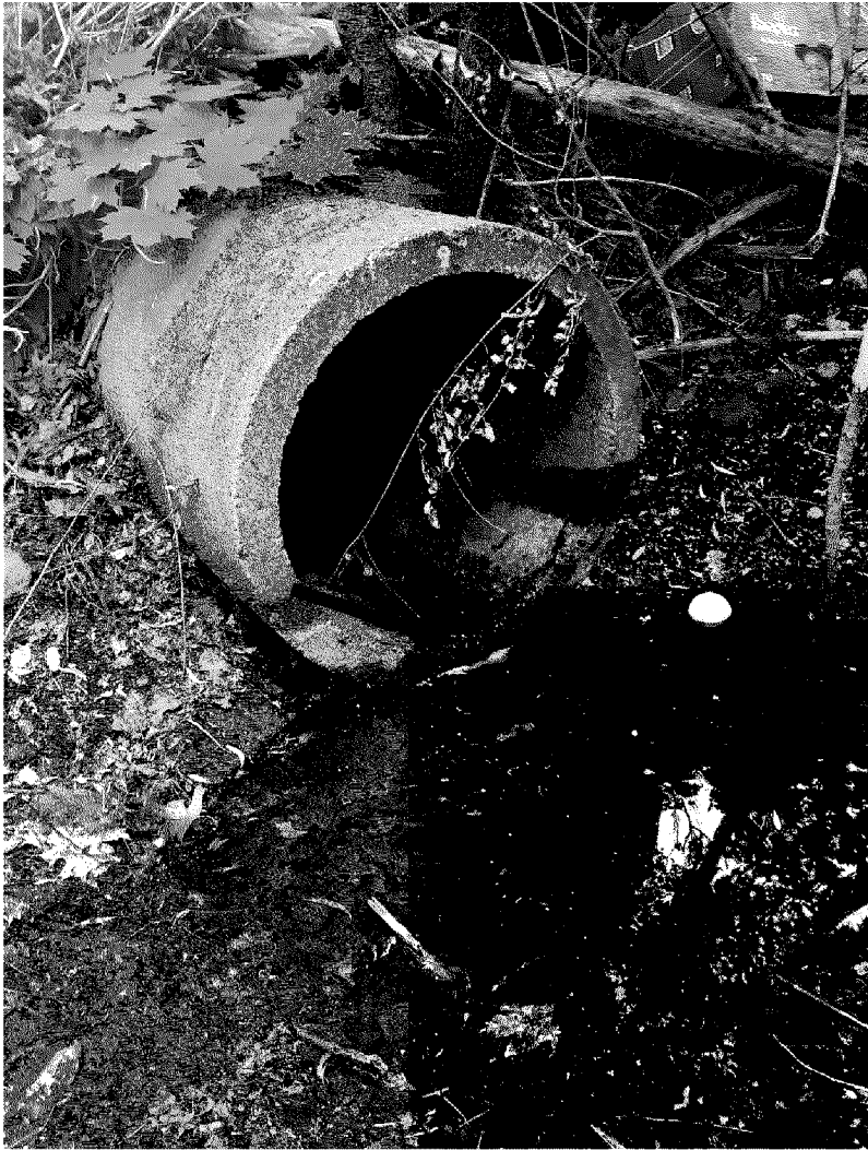
Perkins (photo taken 5/24 at 10:01 AM): Outfall located at the end of Perkins Street flowing into an adjacent wetland to the Merrimack River. Sample point is indicated by a red arrow.
