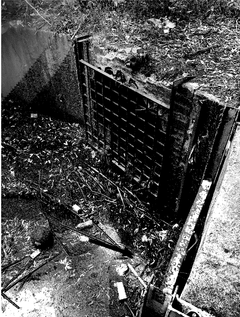
76Swan (photo taken 5/24 at 11:21 AM): Gated outfall located on the north side of the CVS parking lot at 76 Swan Street (dry at time of inspection). In-stream sample of the stream coming from Searles Pond collected just before the opening of the culvert pipe that flows under the parking lot. Sample point is indicated by a red arrow.
