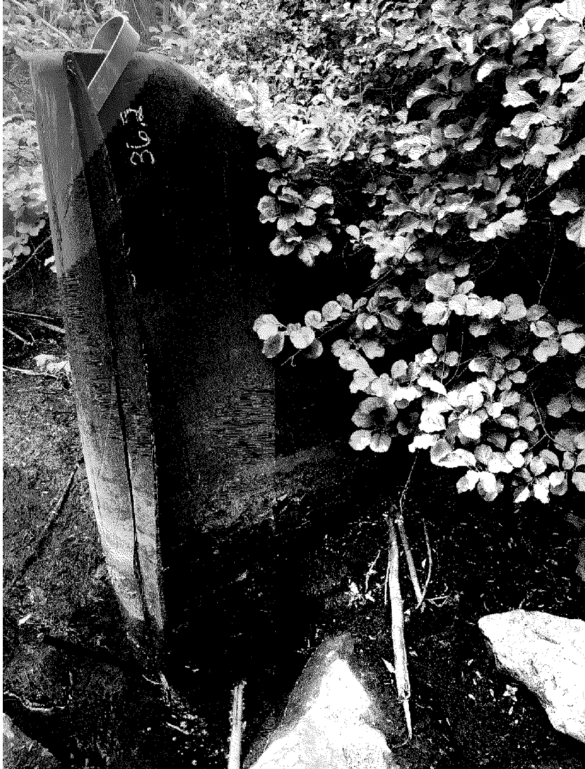
ParkStCVS (photo taken 5/24 at 12:58 PM): Outfall with duckbill located on the southeast corner of the CVS parking lot on Park Street, flowing into the Spickett River. Sample point is indicated by a red arrow.
