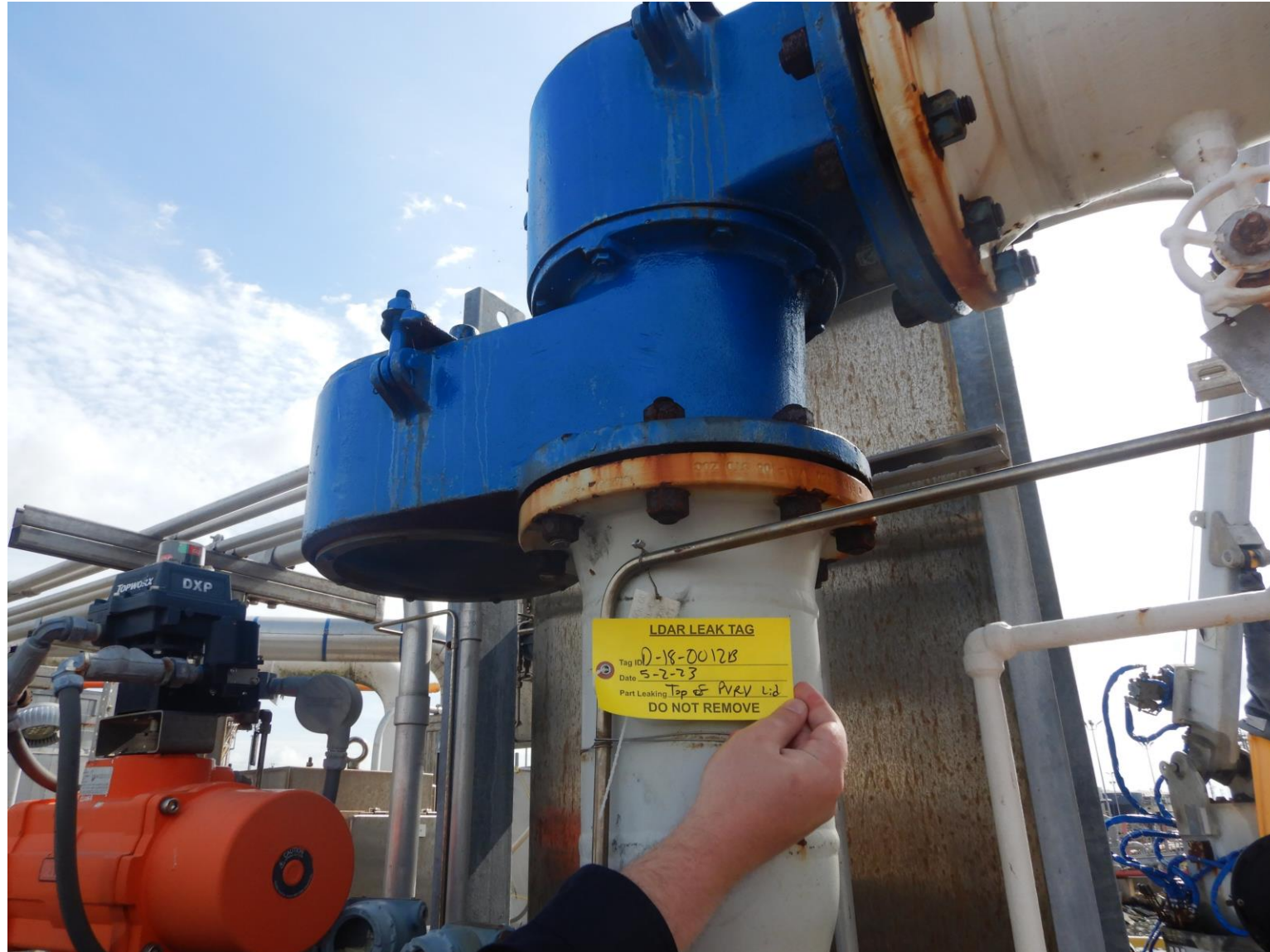
Photo 1158: LDAR Tag D-18-0012B on the Dock 54 PRV 5/2/23 9:47 DSCN1158.jpg
