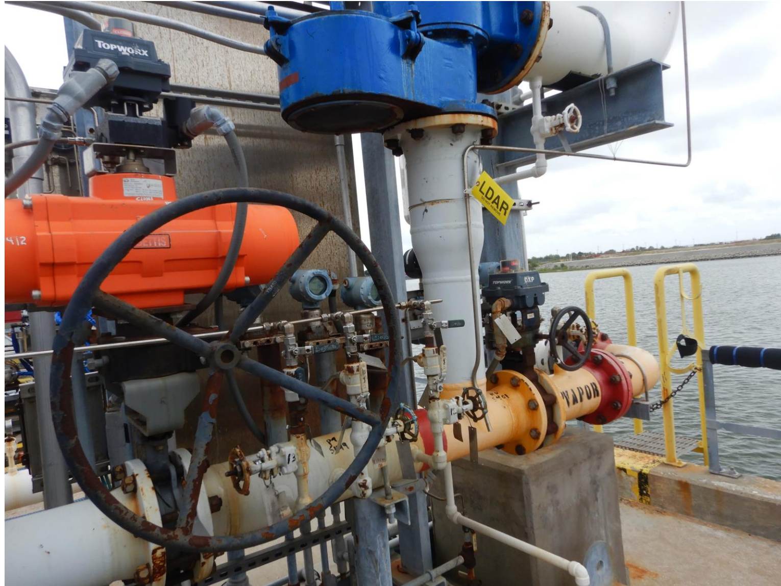
Photo 1166: Manual valve and PVRV for Dock 54 vapor line 5/4/23 12:15 DSCN1166.jpg
