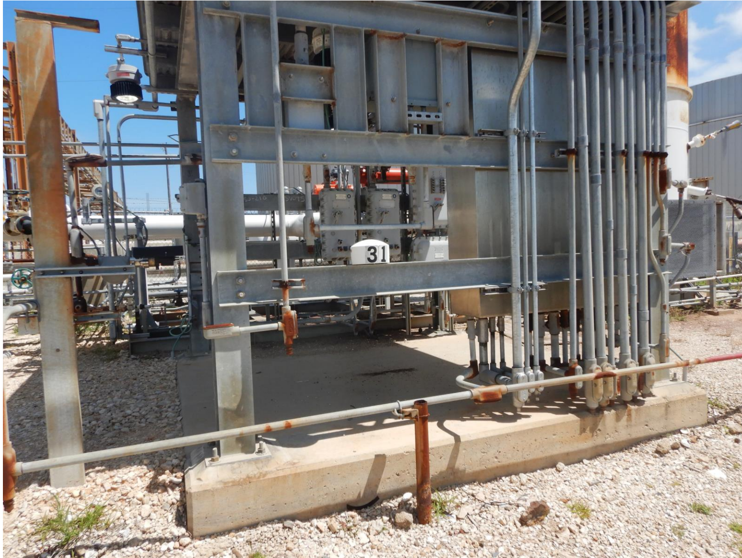
Photo 1154: Shelter 31 improper placement - 5/1/23 11:51 DSCN1154.jpg
