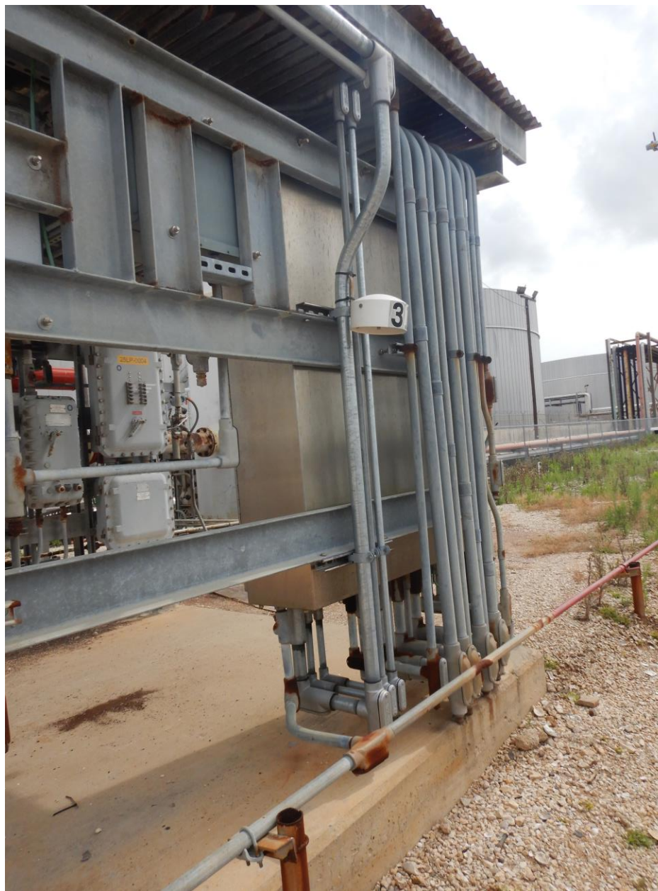
Photo 1160: Shelter 31 placement after facility corrected 5/2/23 10:28 DSCN1160.jpg
