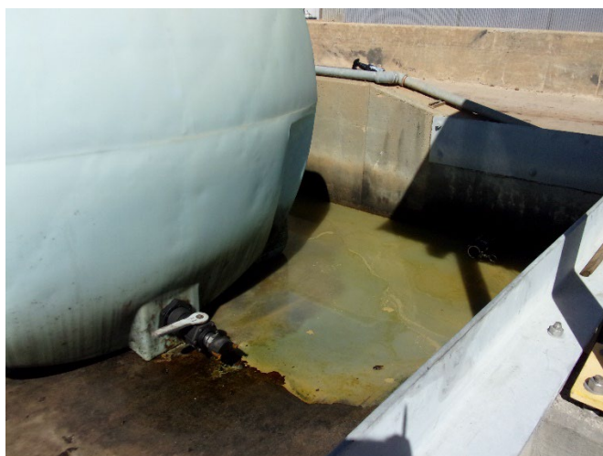
Photo-8 Oily Residue in Secondary Containment
