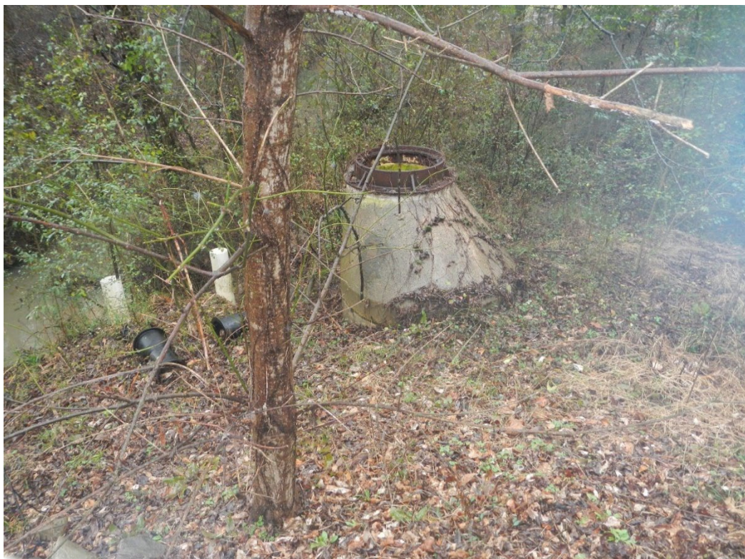
Figure 6: Inlet structure with missing manhole.
