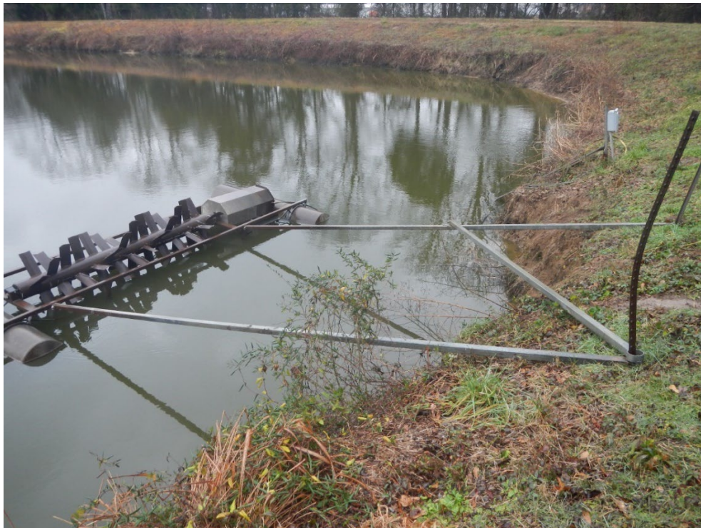
Figure 12: Lagoon aerator was not operational.
