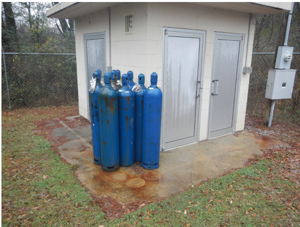
Figure 13: Empty and partially empty chlorine tanks
