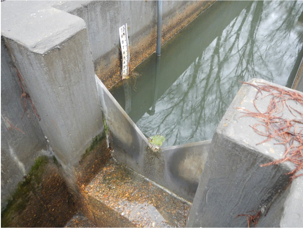
Figure 9: Effluent V-notch weir with staff gauge.
