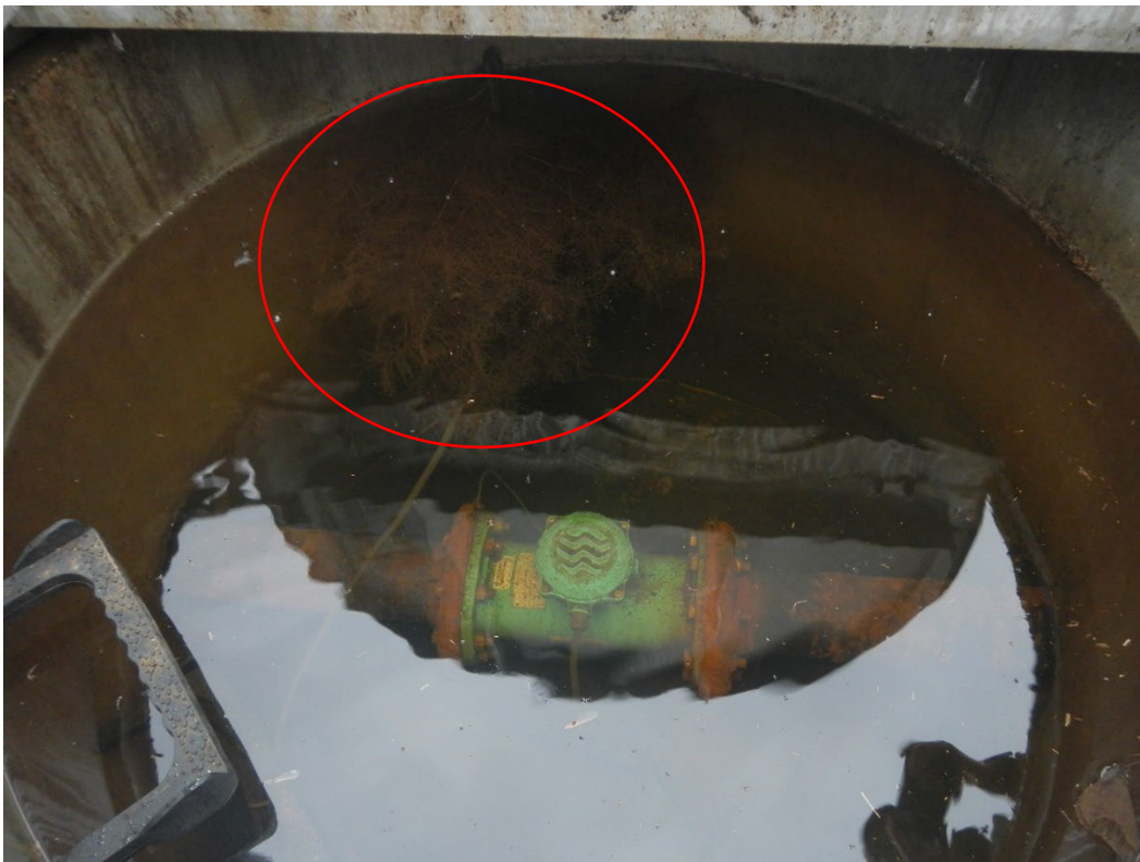
Figure 3: Inline flow meter located between final lagoon and chlorine contact chamber. Flow meter access hole is shown flooded with plant roots growing into chamber.
