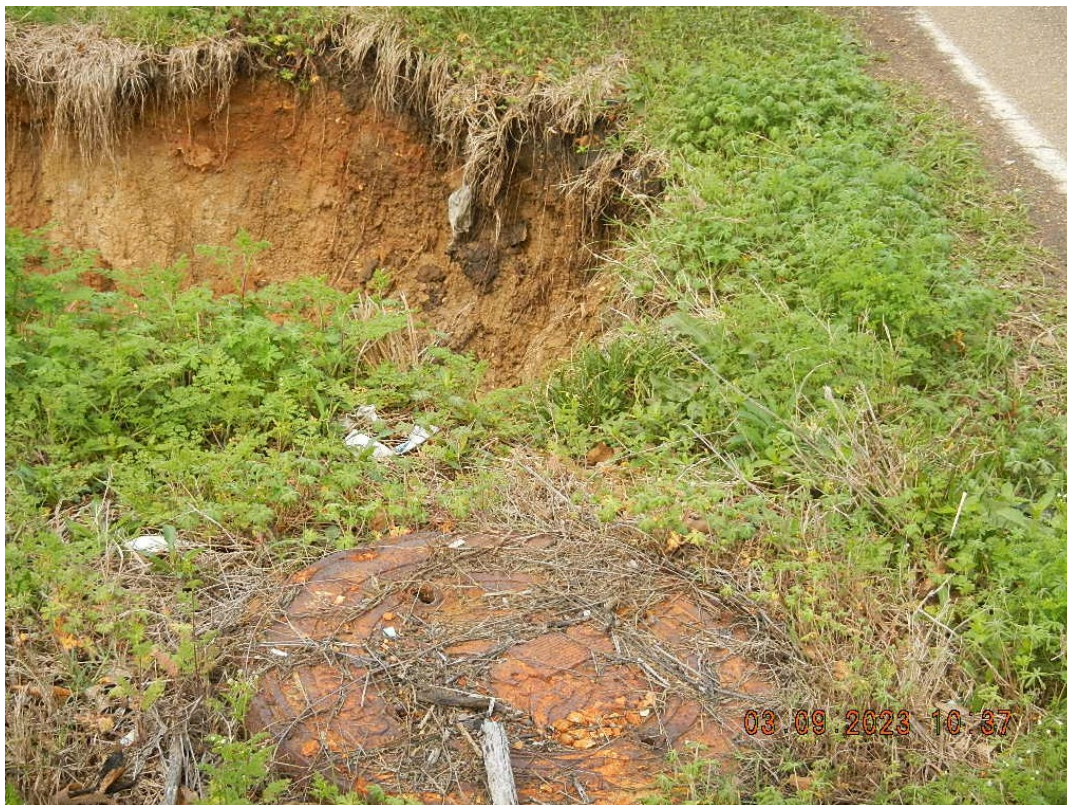
Photo 6: Sink hole likely caused by collapsed sewer main.
