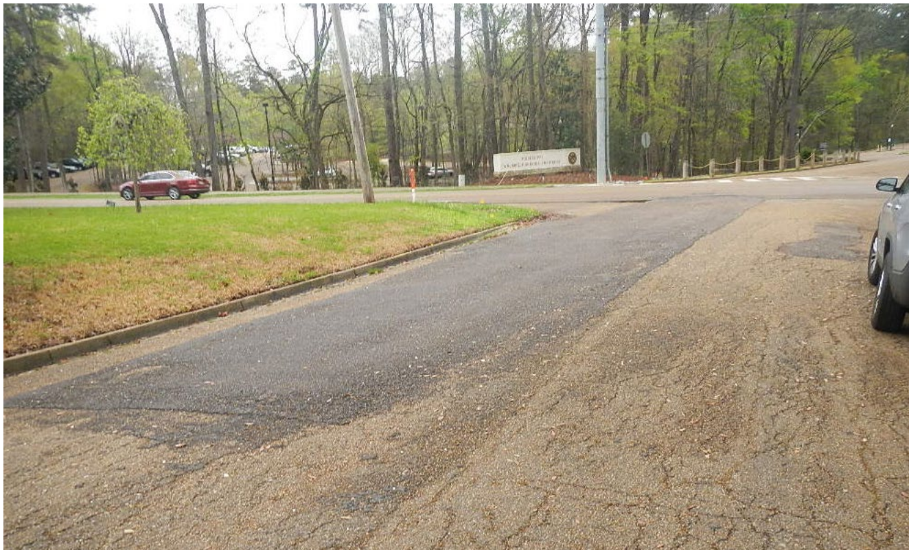
Photo 5. Previous point repair on Eastline Road.
