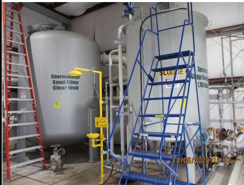
PHOTO #2 – Stormwater Treatment System
