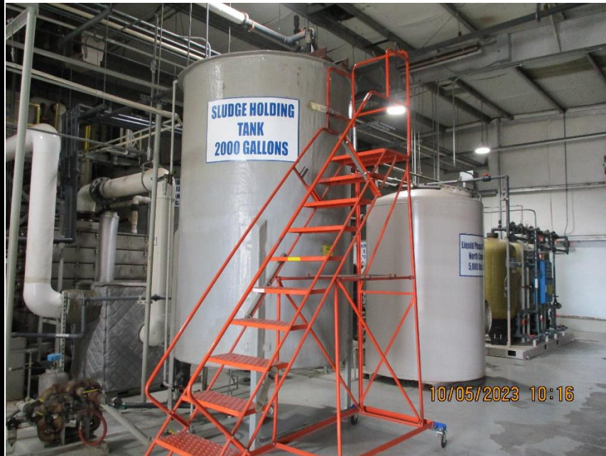
PHOTO #1 – Groundwater Treatment System
