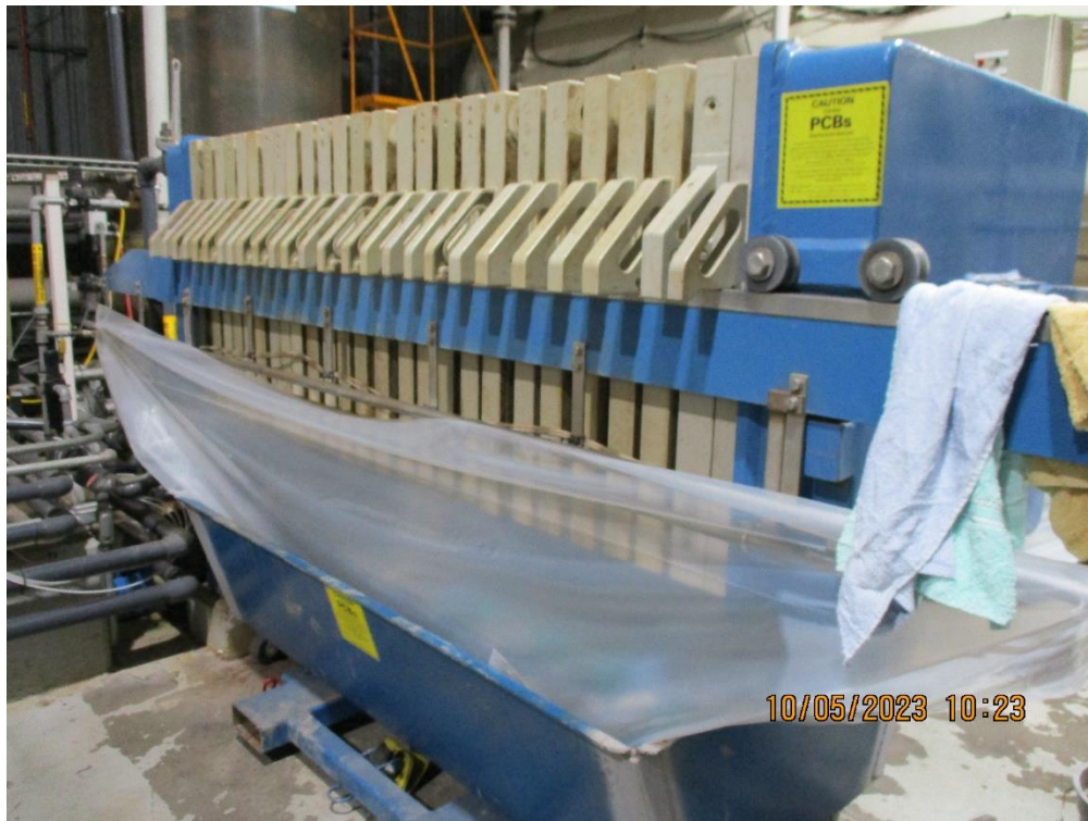
PHOTO #3 – Press sludge system and container with “PCB” label
