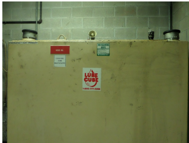
Picture 5: 650-gallon Used Oil Tank
