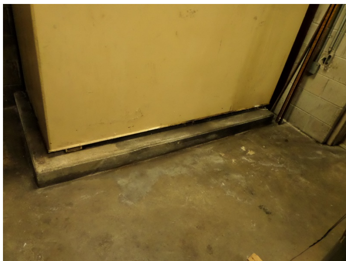
Picture 7: Used Oil Spill Cleaned during Inspection
