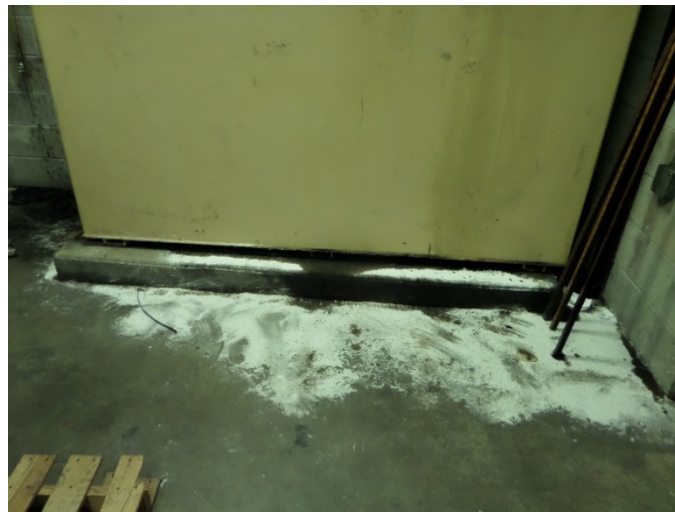
Picture 6: Absorbent material covering the used oil spill
