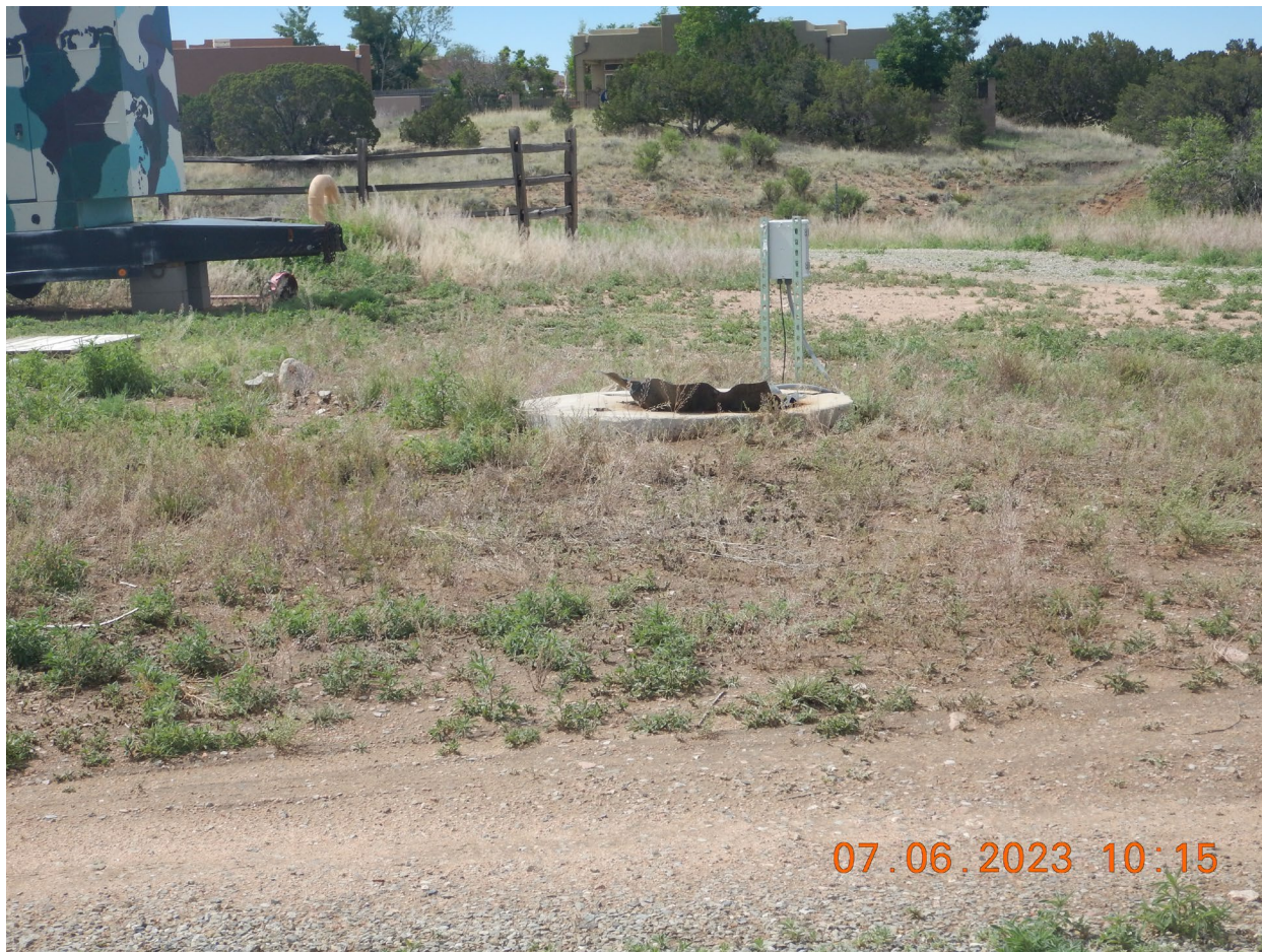
View of the adjacent wet well located at the approximate Northwest corner of the Operators Building. Note: the lack of perimeter fencing and vegetative overgrowth. (DSCN2551) Photographed by D. Esparza
